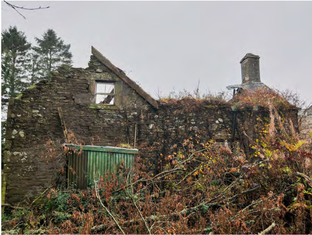
Fig. 9 - The NE side elevation of the farmhouse with part of its gable and window
