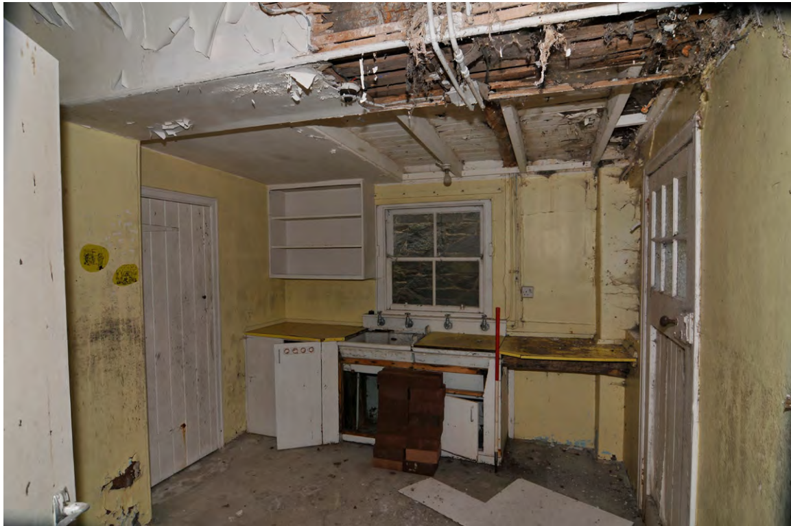
Fig. 23 - Building 3, Unit 32, kitchen and boarded window
