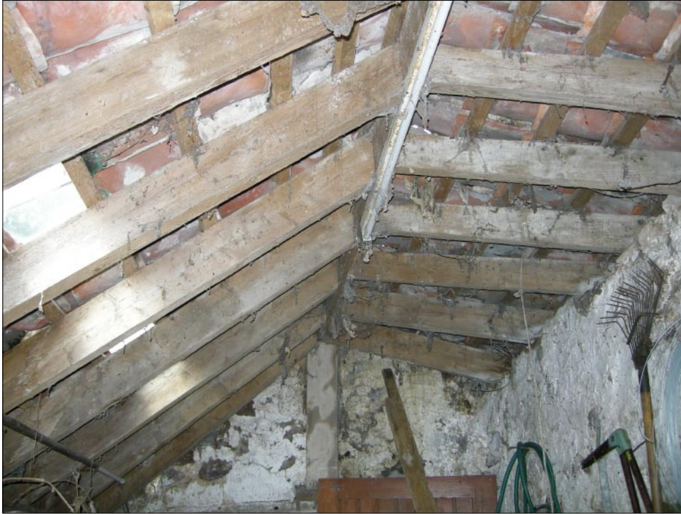
Fig. 24 - General shot of Potting shed western compartment interior roof from the east
