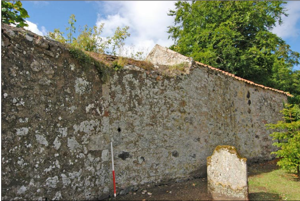
Fig. 30 - General shot of north facing elevation of Potting shed and 'Manse' wall with stone wall between - from the north-east
