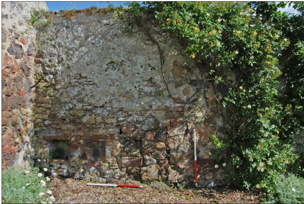
Fig. 26 - South facing elevation of stone wall between Potting shed and 'Manse' wall
