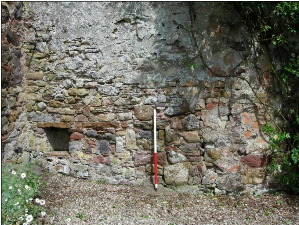
Fig. 27 - South facing elevation of stone wall between Potting shed and 'Manse' wall - close-up of Bee Boles
