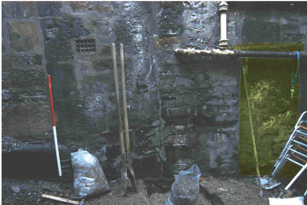
Plate 16 - Bishop's Close, blocked doorway
