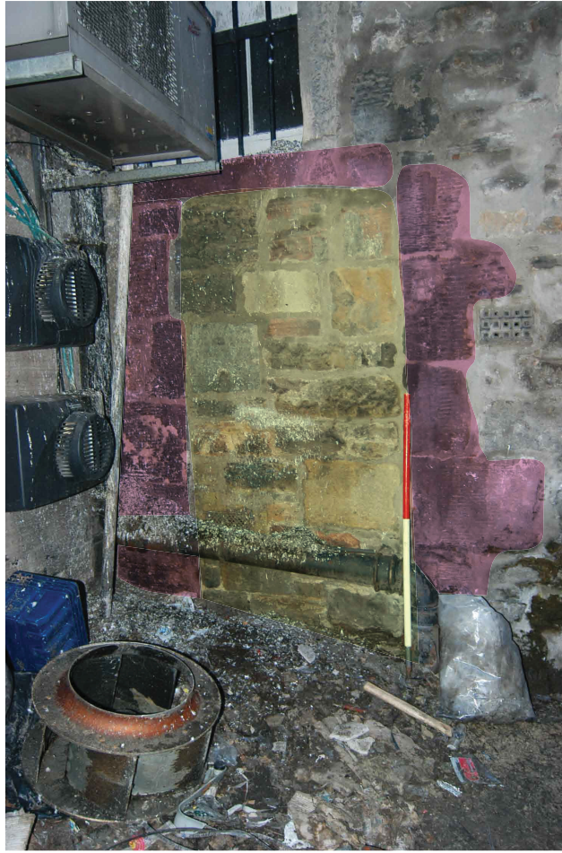
Plate 15 - Bishop's Close, blocked doorway
