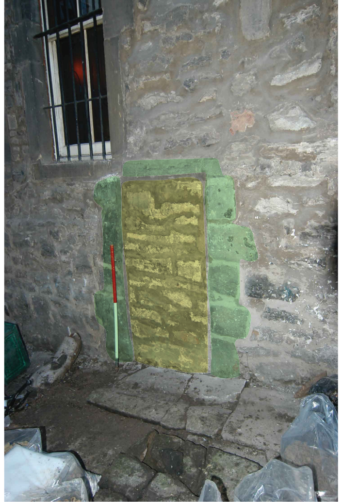
Plate 14 - Bishop's Close, blocked doorway
