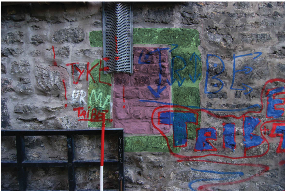
Plate 7 - North Gray's Close, blocked window
