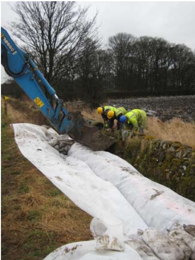
Fig. 24 - Flume pipe in place within ditch and demolition of upper courses of boundary wall FB05 in progress
