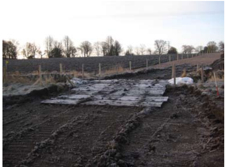
Fig. 25 - Completed access point across the top of the flume pipe and boundary wall FB05
