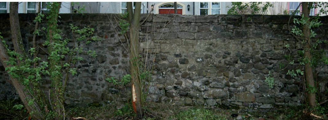
Plate 8 - North-facing elevation, section of wall that is bulging outwards
