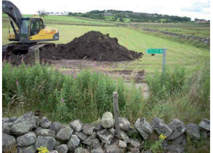
Fig. 3 - General view of the pipeline route pre-excitation looking east with the location of the northern tie-in top left and Wall 8 in the foreground
