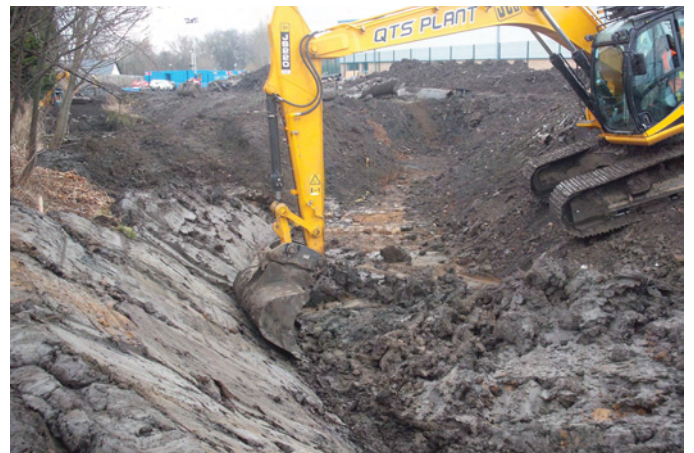
Fig. 8 - Shot of grading batter for new course of Braid Burn from NE
