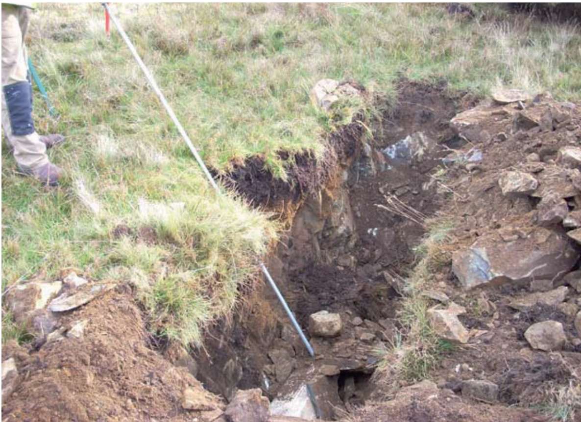
Fig. 3 - A typical anchor hole with the anchor stay in place. Thin topsoil and subsoil overlies bedrock.
