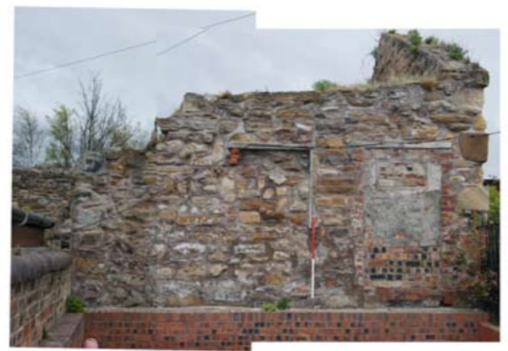
Fig 22a - North Elevation, Photo montage showing the external wall of the Custom House
