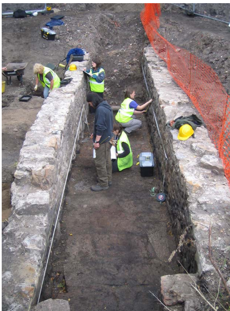
Fig. 7: The interior of the glassworks flue, with flagstone and brick floor visible
