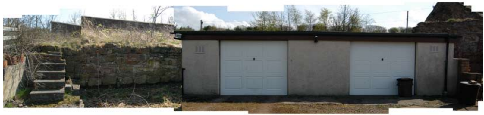
Fig 22c - North Elevation, Photo montage showing the external wall of the Custom House
