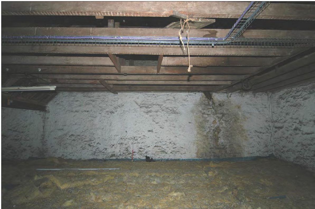
Plate 10 - M-shaped profile of an earlier roof line visible on the internal west gable of the grain store in Unit 20.
