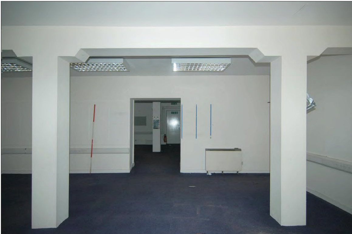
Plate 8 - Boxed in columns and wall finishes within the ground floor of the former grain store (Unit 16).
