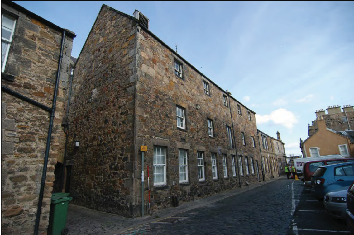
Plate 1 - East-facing elevation of the former City Bank (No 52) and the north-facing elevation of 53-54 High Street.
