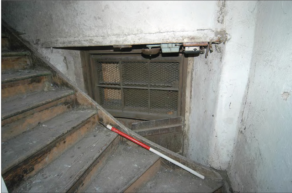
Plate 9 - Blind window situated on the partition wall between Units 20 and 40 on the second floor.
