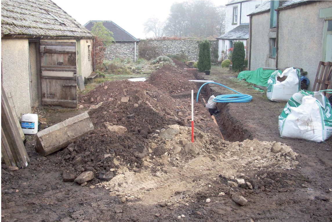
Fig. 3 View of the sewer pipe route passing through the yard to the west of the Manse
