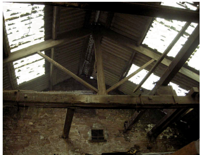
Plate 10 - South-facing interior gable of Unit 5) showing the A-frame trusses with king post
