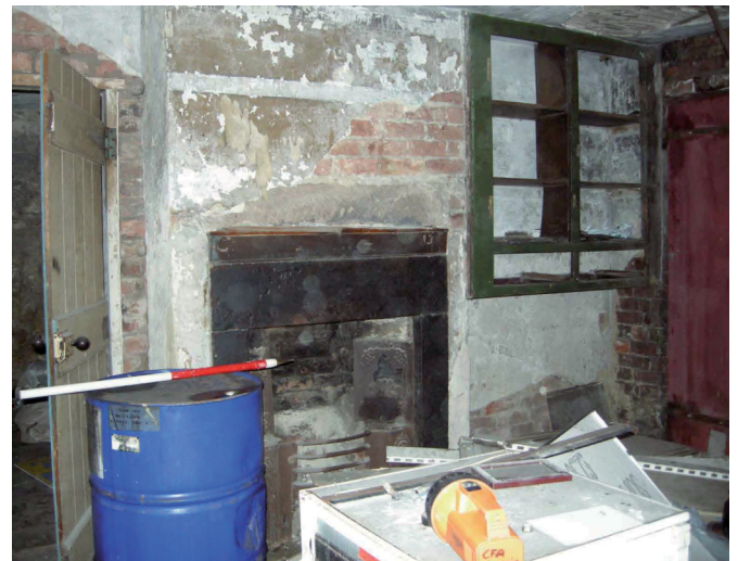
Plate 4 - Interior south facing elevation in Unit 6c with ornate early Victorian fire-surround
