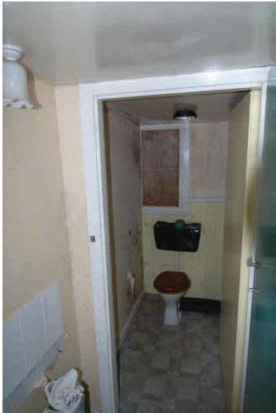
Fig 18. Interior: toilet with partition and blocked window
