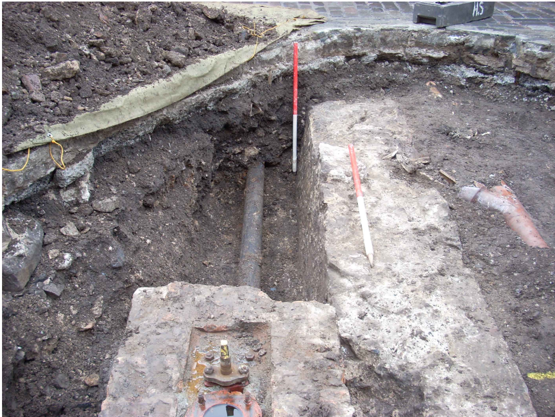
Fig. 5 - The location of the fire hydrant (662) adjacent to the Blast Wall 665. The vertical ranging rod shows the batter of the wall
