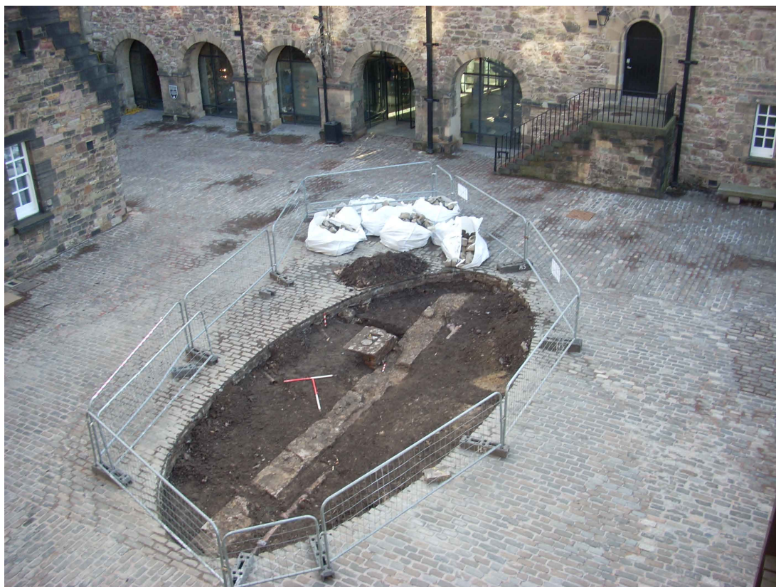
Fig. 2 - View of the 'flower bed' from the north-west once the setts and underlying grout were removed. Most of the overlying drains have also been removed
