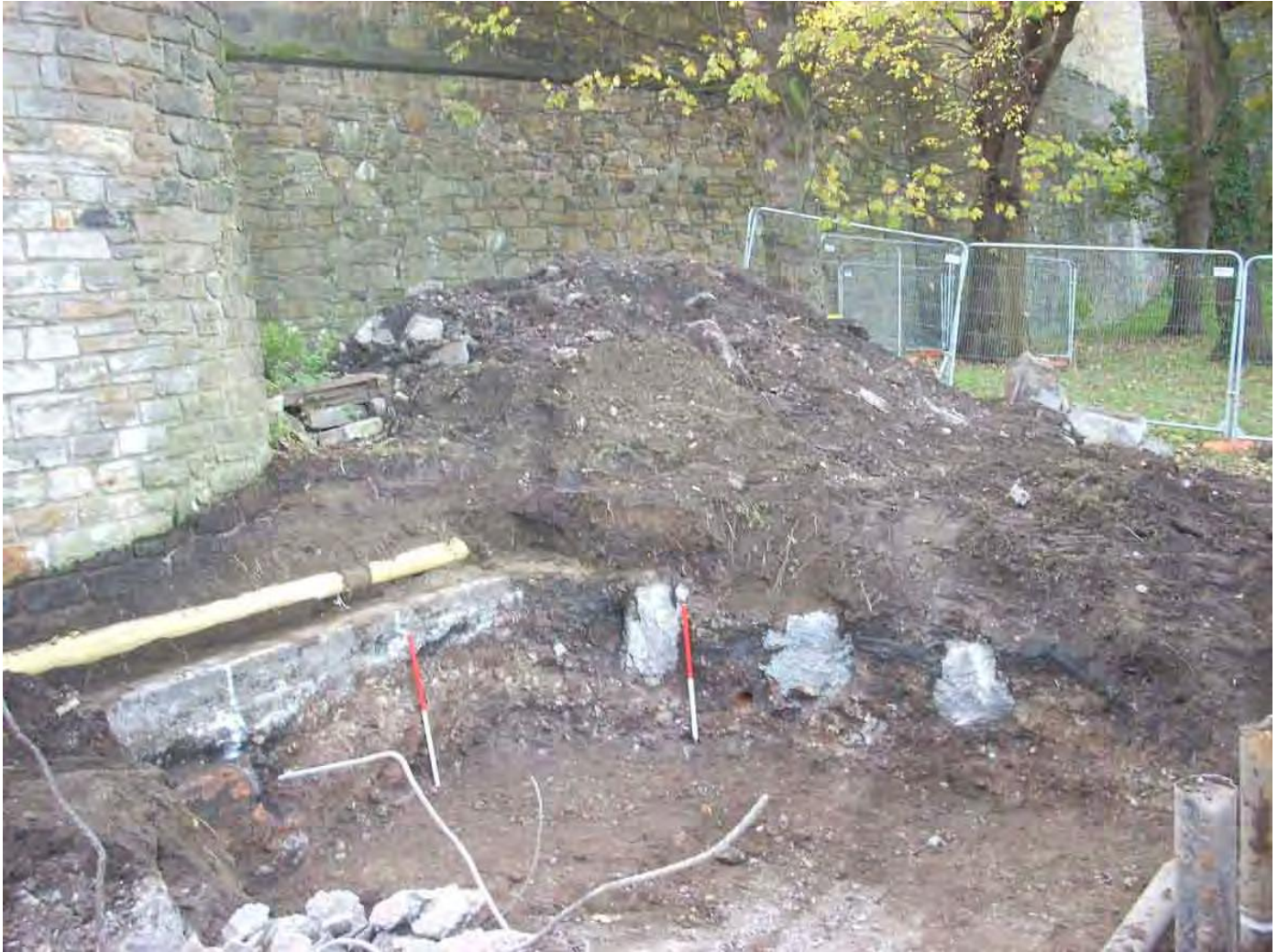
Fig. 9 View of the east and north facing sections at the west end of the works in Princess St Gardens showing the extent of the 1960s Raker foundations 515
