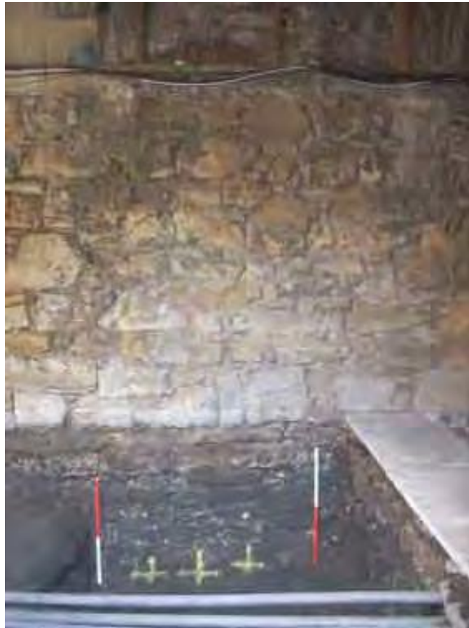
Fig 15. General view of Moat Vault rear wall face prior to core drilling
