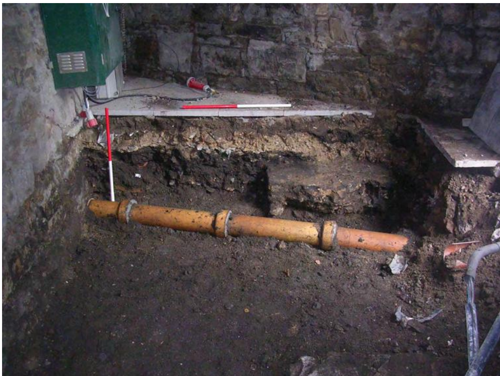
Fig 22. Moat Vault. General shot of west-facing section through Moat Vault showing masonry 472
