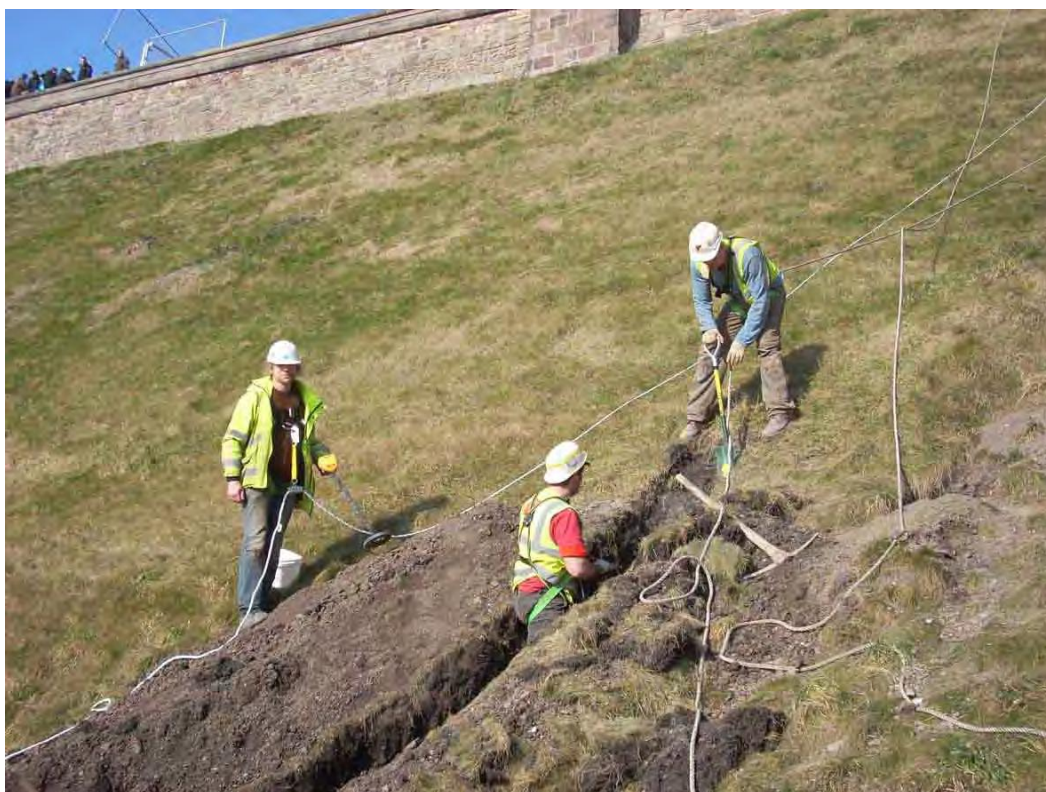
Fig 31. Water Main trench between the Esplanade and Johnston Terrace showing hand excavation and metal detecting in progress
