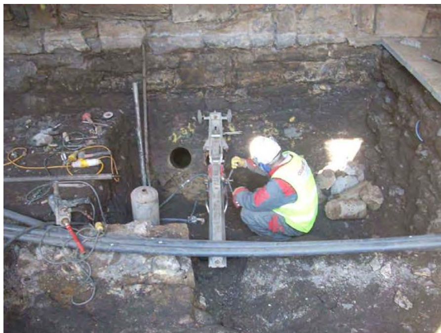
Fig 16. View of the exposed interior Moat Vault Wall face during core drilling
