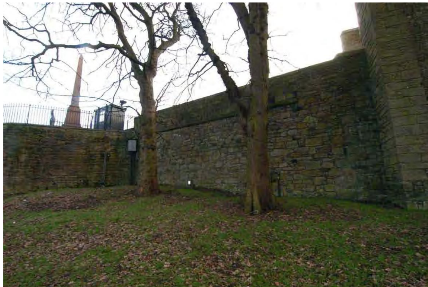
Fig 2. General view of the Moat Vault exterior wall and the Princes Street Gardens excavation area prior to trenching works
