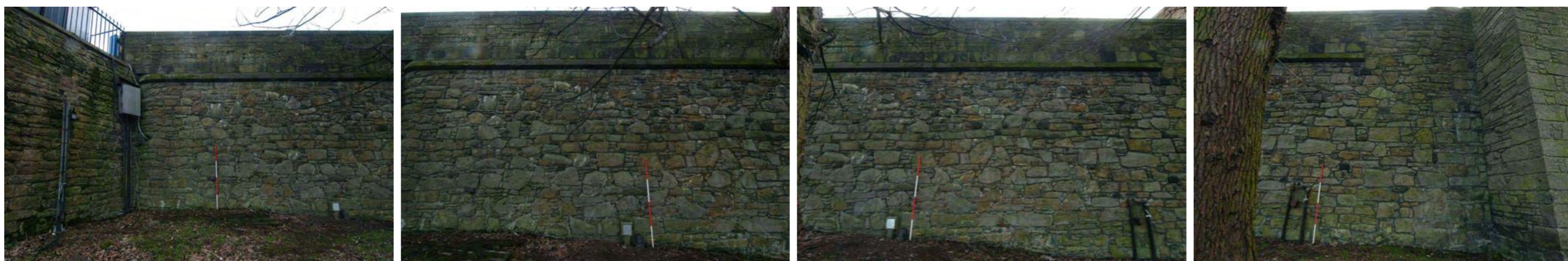
Fig 3. Photographic survey of the Moat Vault exterior wall above existing ground level
