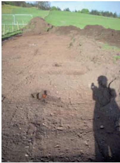
General shot of topsoil stripping for temporary compound showing bases of modern fence posts
