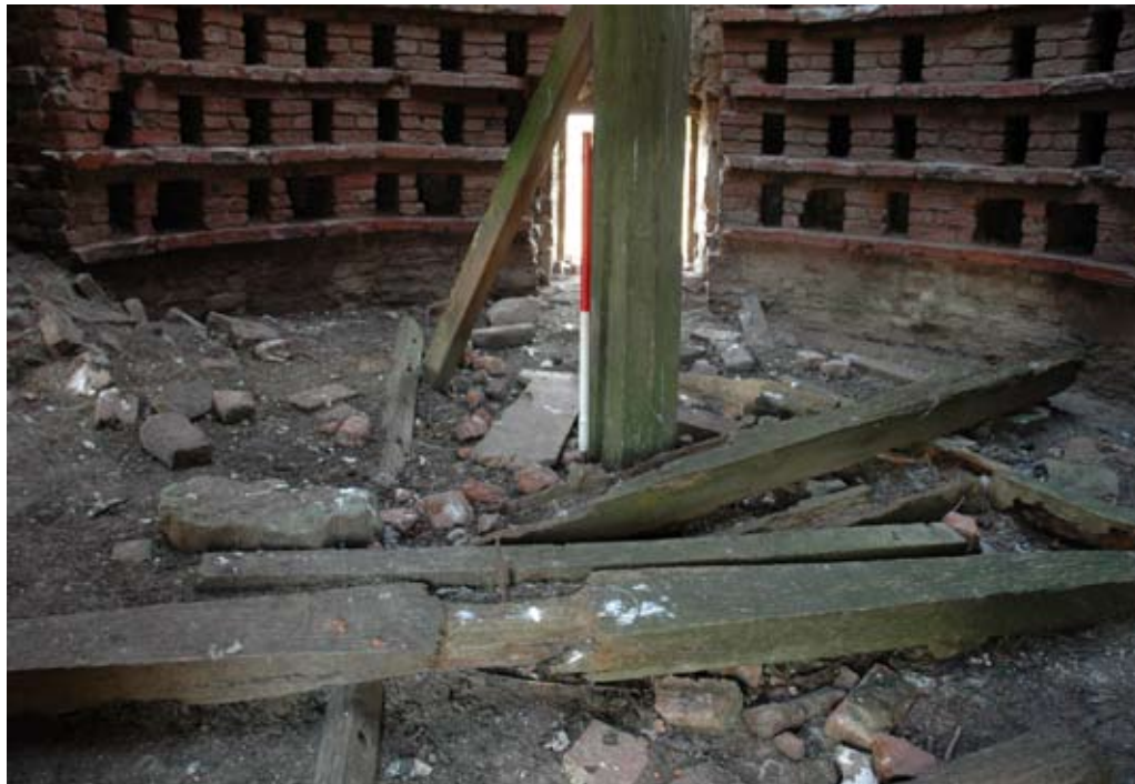
Fig. 11 - Fallen timbers prior to clearance
