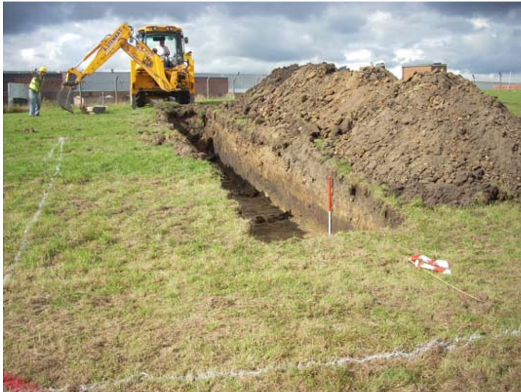
Fig. 3 Trench 1, general view from the east showing the made ground deepening to the west
