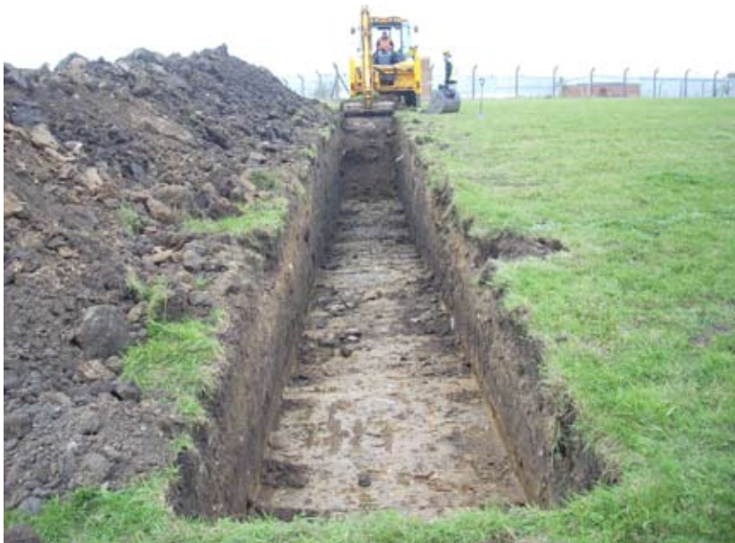
Fig. 5 Trench 3, General view from the east during excavation showing the depth of made ground to the west
