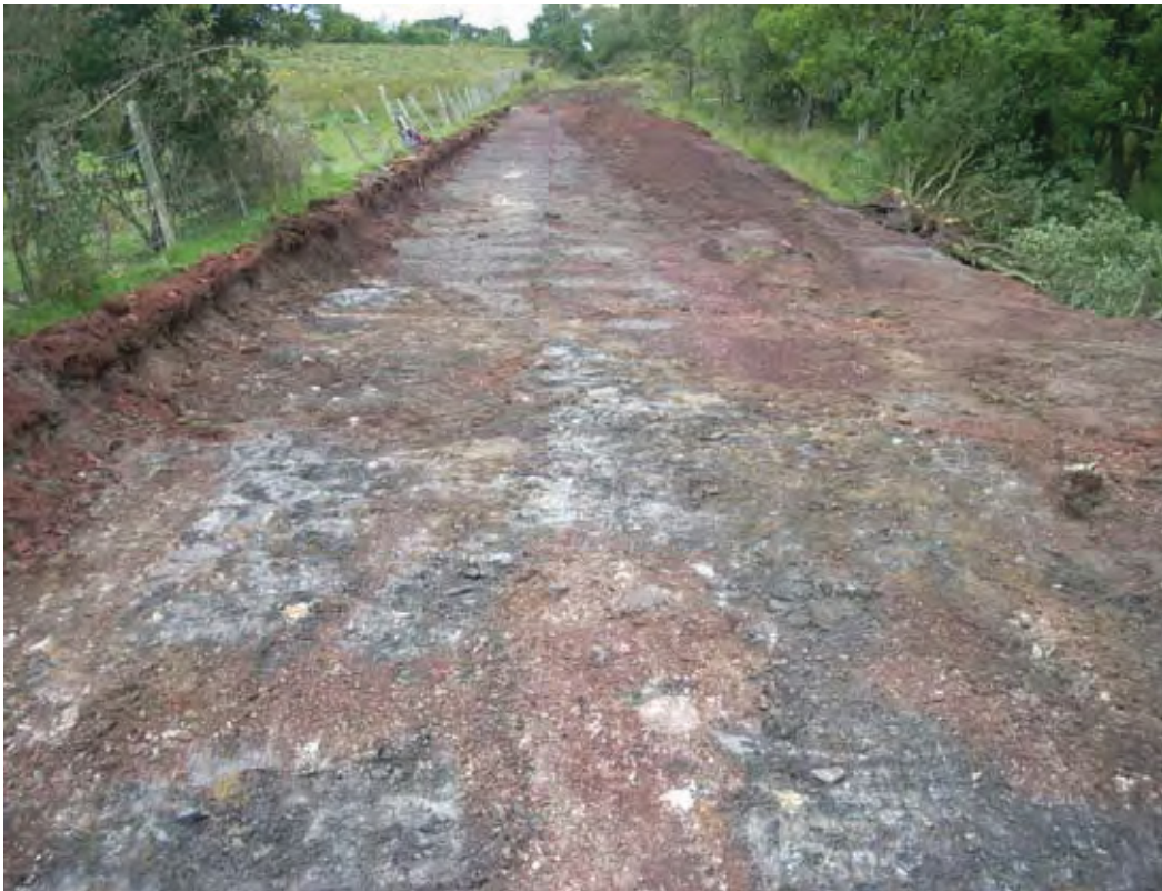
Fig. 3 View of access track with exposed railway formation level on RSK Site 13
