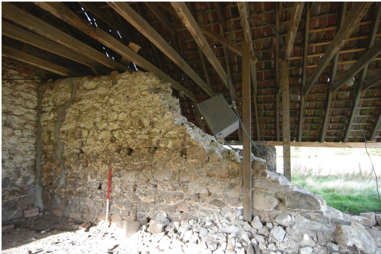
Plate 7. East-facing interior wall of the west gable and adjoining central partition wall
