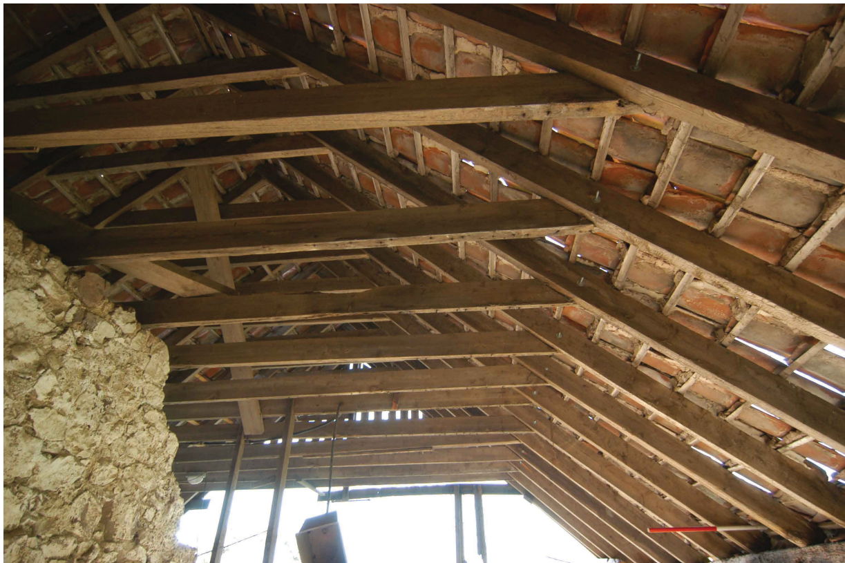
Plate 8. South-facing elevation of the central partition wall and scarf-joint details on the tie beam
