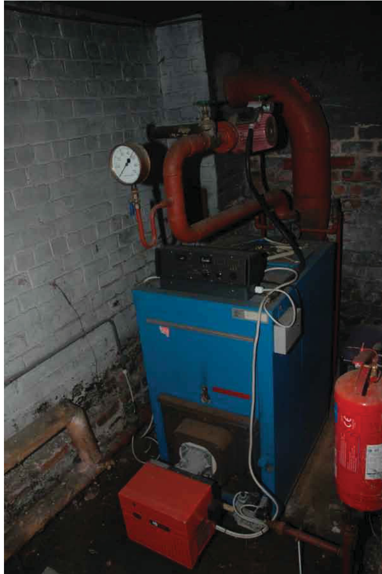
Fig. 28 View inside boiler room (Unit 19)
