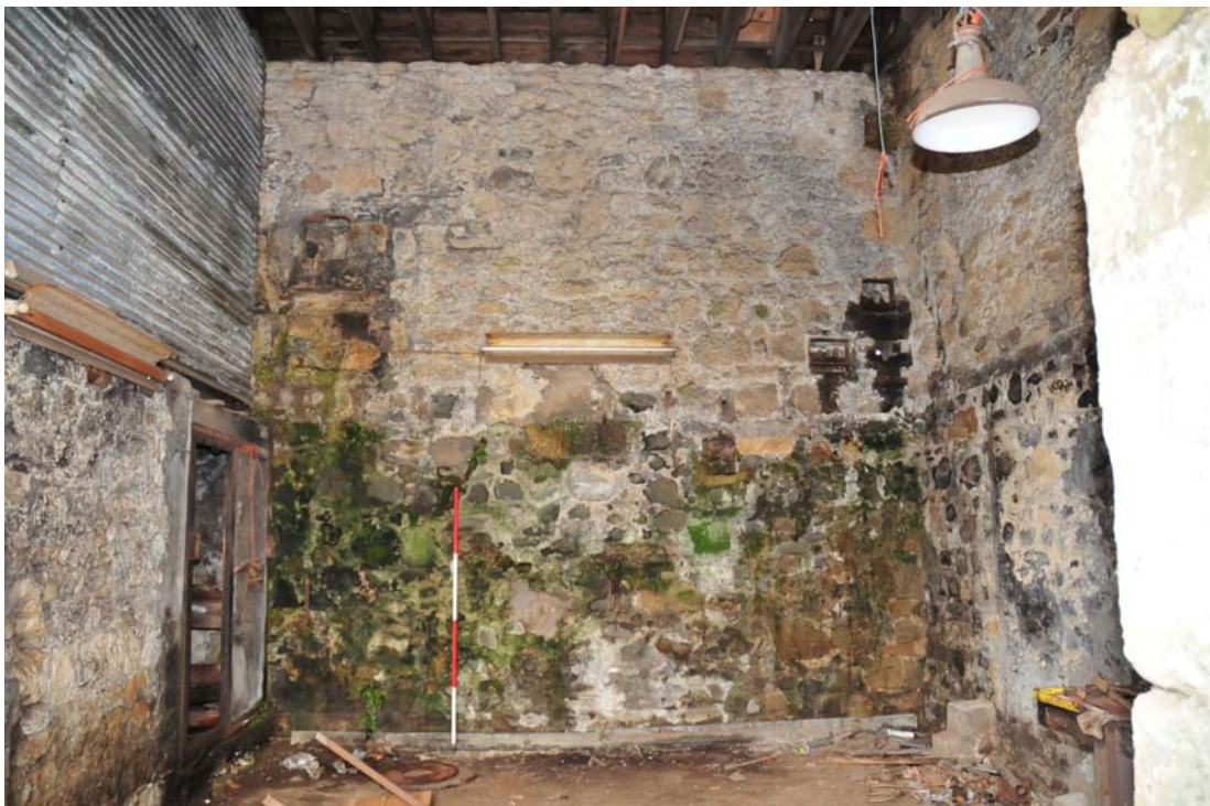
Fig. 24 Building 4 interior, south-west facing elevation and oil stained walls
