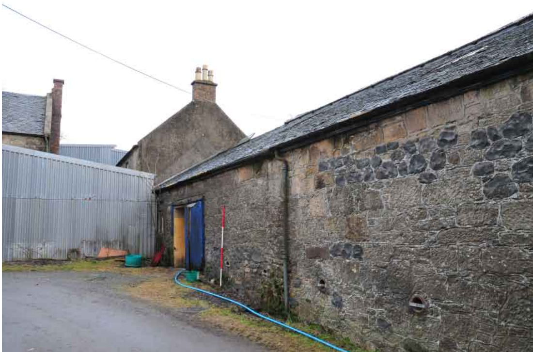
Fig. 28 Building 6 exterior showing the pitched roof stain on gable of Building 5
