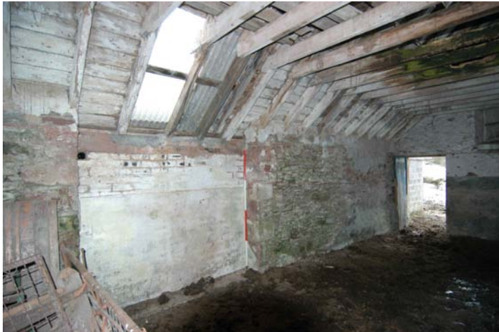
Plate 21- Building 5, general shot of a brick blocking work in an earlier doorway on the north-west-facing elevation
