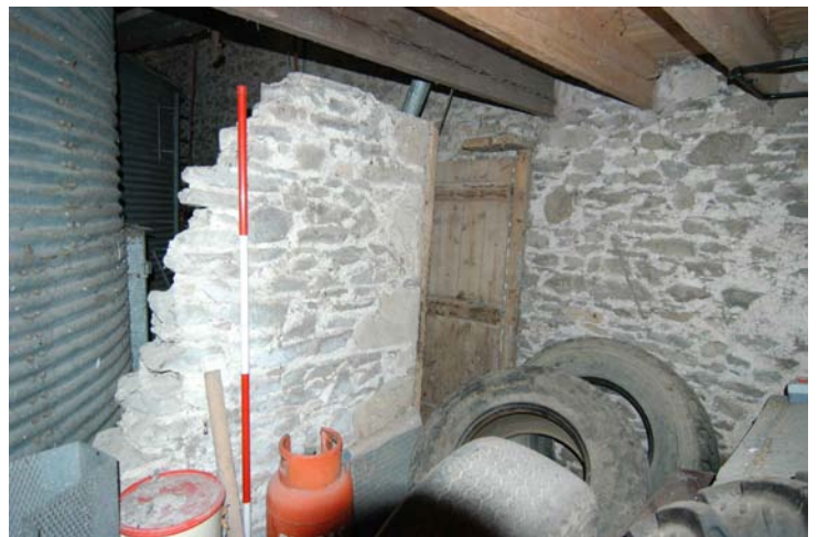
Plate 16- Building 4, interior ground floor, remains of a partition wall near the grain silos
