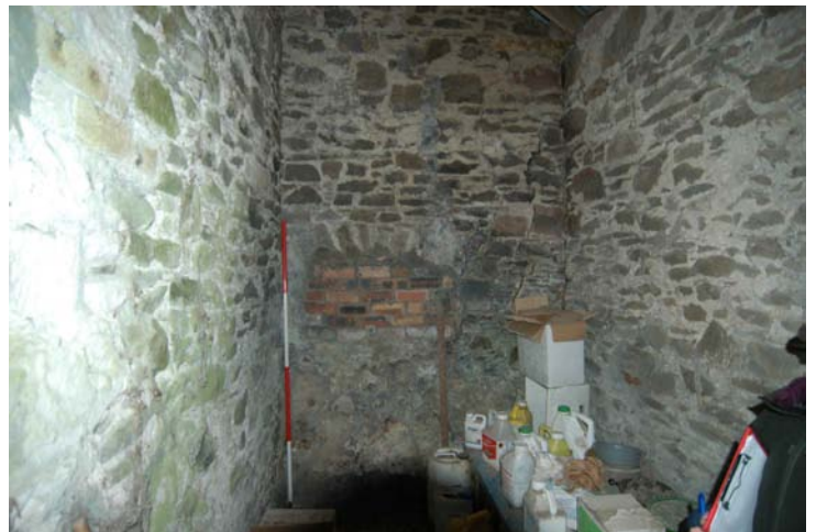
Plate 18-Building 4, interior of rear outshot building, west-facing interior wall with relieving arch for lade
