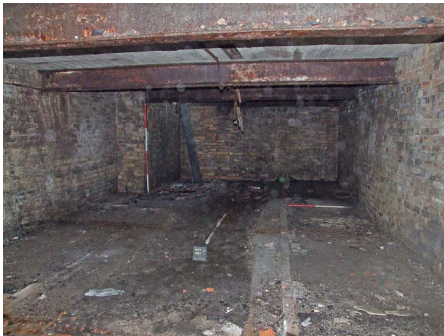
PLATE 6 View of cellar 001, looking north. Note concrete kerbs denoting former shelving extending along either side of the room (scales: 1.0m, 2.0m).
