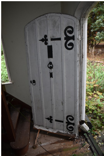
Photograph 9 Exterior door on eastern elevation, with ornate hinges. Photograph taken facing north.
