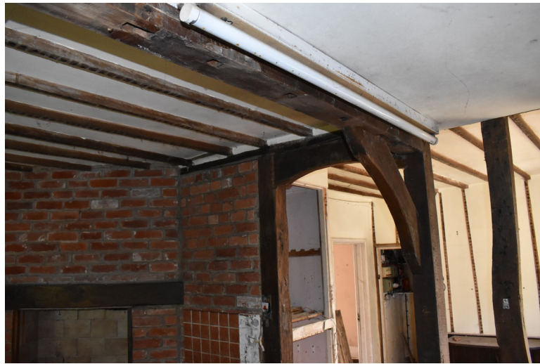
Photograph 15 Underside of beam in ceiling of room 6, showing empty mortices. Photograph taken facing south-east.
