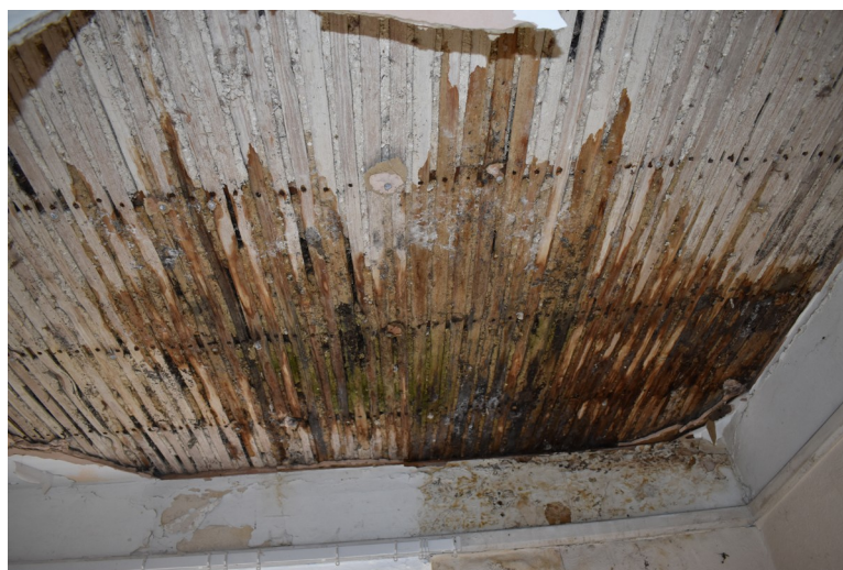
Photograph 28 Roof of room 17, showing exposed lath and plaster. Photograph taken facing south.
