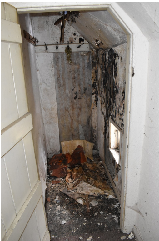
Photograph 27 Interior of room 16, showing water damage due to hole in roof. Photograph taken facing south.
