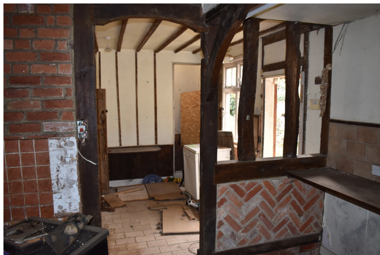
Photograph 16 Herringbone brick plinth and studwork between rooms 6 and 9. Photograph taken facing south.
