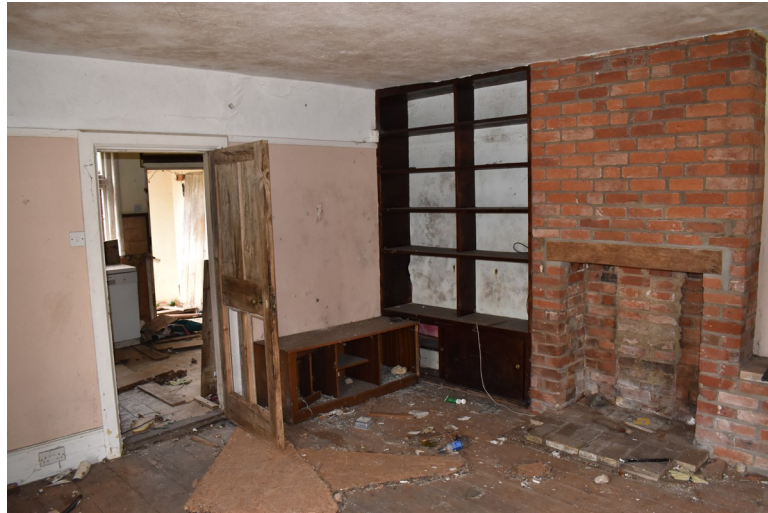
Photograph 21 Interior of room 10, showing rebuilt fireplace and inserted shelving. Photograph taken facing north-west.
