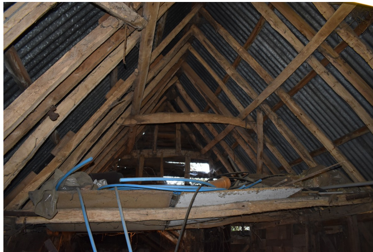
Photograph 9 Interior of bay 2, showing roof structure and suspended floor. Photograph taken facing north-west.
