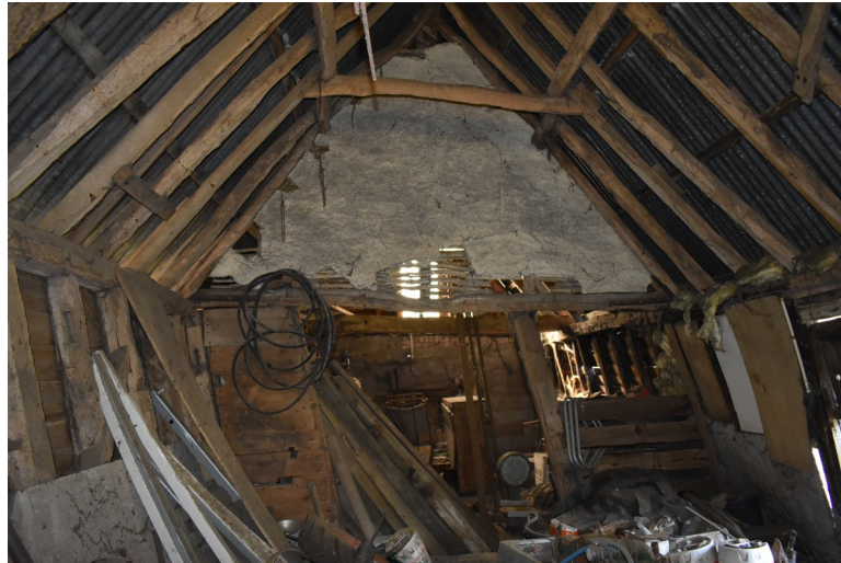
Photograph 10 Interior of bay 2, showing bay division between bays 2 and 3. Photograph taken facing south-east.
