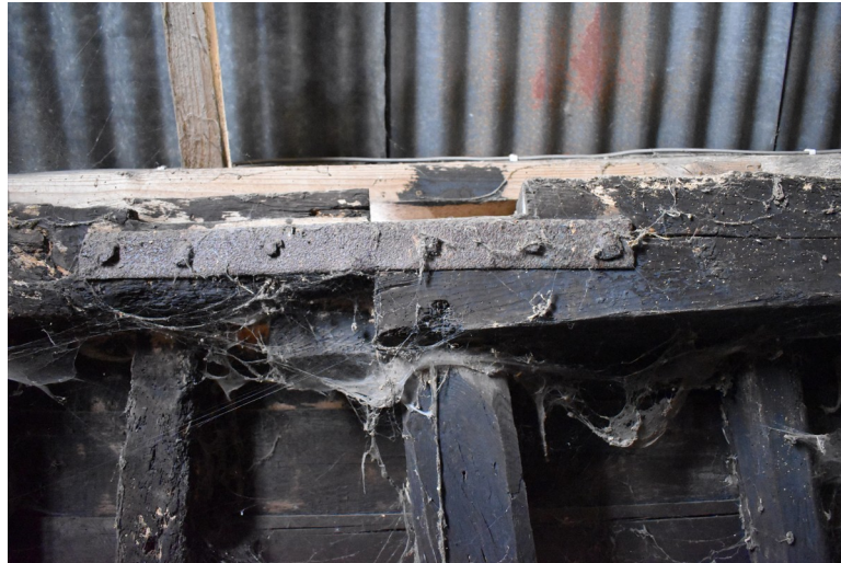
Photograph 17 Detail of rudimentary scarf joint supported by metal strap in bay 3, connecting wall-plate to rebuilt gable-end. Photograph taken facing south-west.
