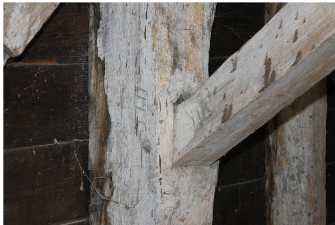
Photograph 29 Detail of north-east corner-post of building, showing carpenter's mark 'IIII' on post and brace. Photograph taken facing south-east.
