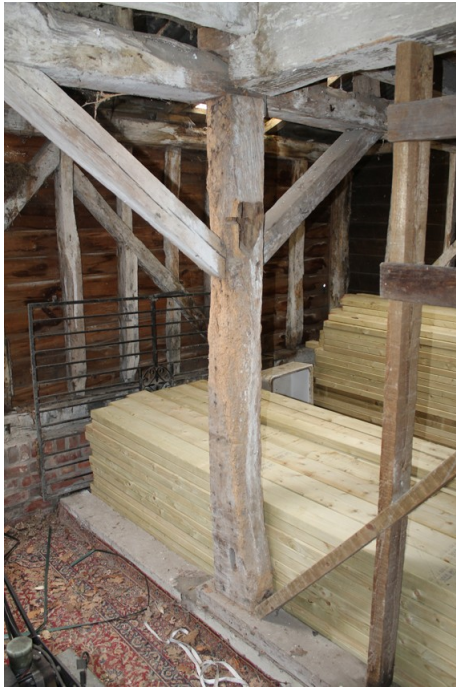
Photograph 28 Detail of northern principal-post between bays 4 and 5, showing mortice on southern face. Photograph taken facing north-east.
