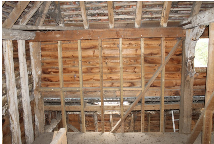
Photograph 11 Northern elevation of bay 1 on first-floor, showing modern studs and wall-plate. Photograph taken facing north.
