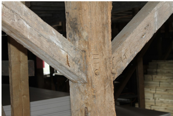
Photograph 27 Detail of northern principal-post between bays 4 and 5, showing carpenter's marks 'II' and 'III'. Photograph taken facing south-west.
