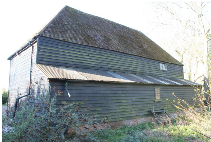
Photograph 4 Northern elevation of building, show lean-to supported on brick plinth. Photograph taken facing south-west.
