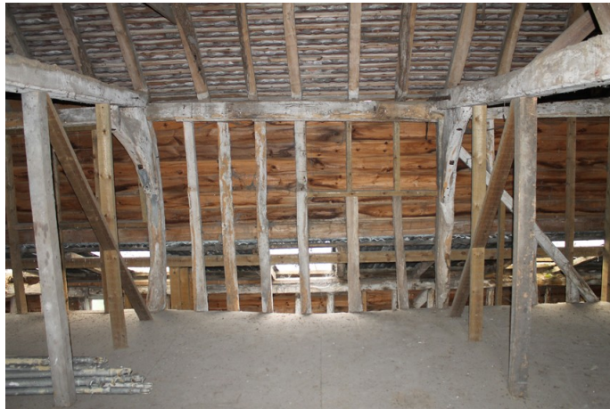
Photograph 26 Northern elevation of bay 4, showing inserted, and subsequently blocked, window opening. Photograph taken facing north.
