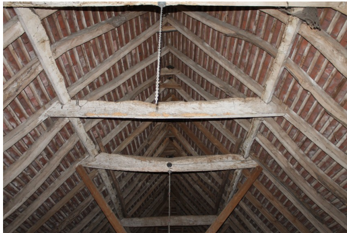
Photograph 6 Detail of roof, showing hand-sawn collars, rafters and purlins. Photograph taken facing east.
