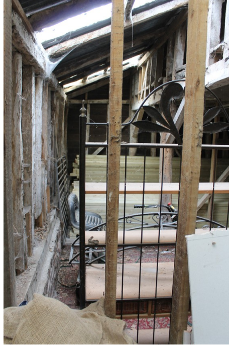
Photograph 30 Interior of lean-to, with re-used hand-sawn studs to left of frame. Photograph taken facing east.
