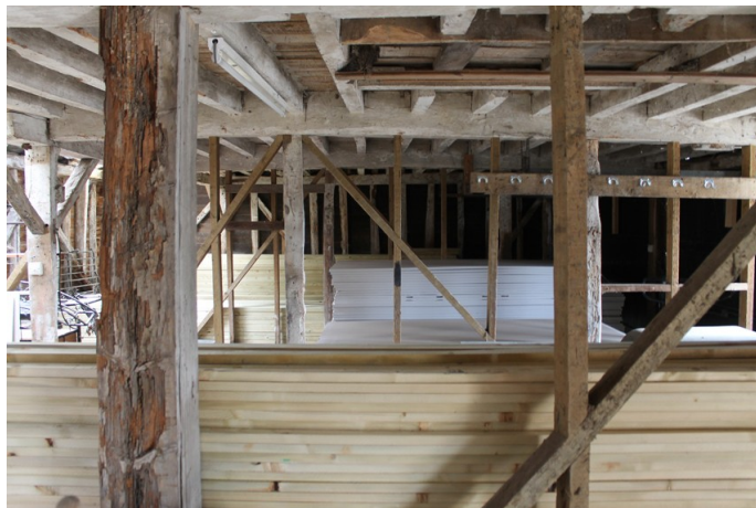
Photograph 22 Ground-floor of building. Trapdoor in bay 3 visible to top right of frame. Photograph taken facing east.
