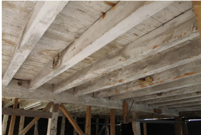
Photograph 8 Floor joists above bay 3, showing binding-beam between bays 3 and 4. Photograph taken facing south-east.
