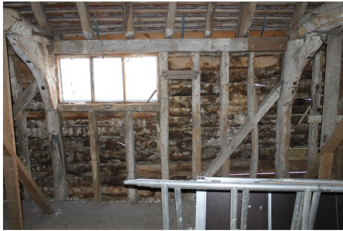
Photograph 25 Southern elevation of bay 4 on first-floor, showing inserted window and scarf joint on wall-plate. Photograph taken facing south.
