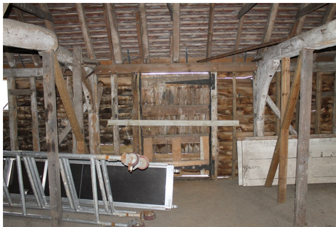
Photograph 19 Southern elevation of bay 3 on first-floor, showing modern studs and original pitching-door. Photograph taken facing south.
