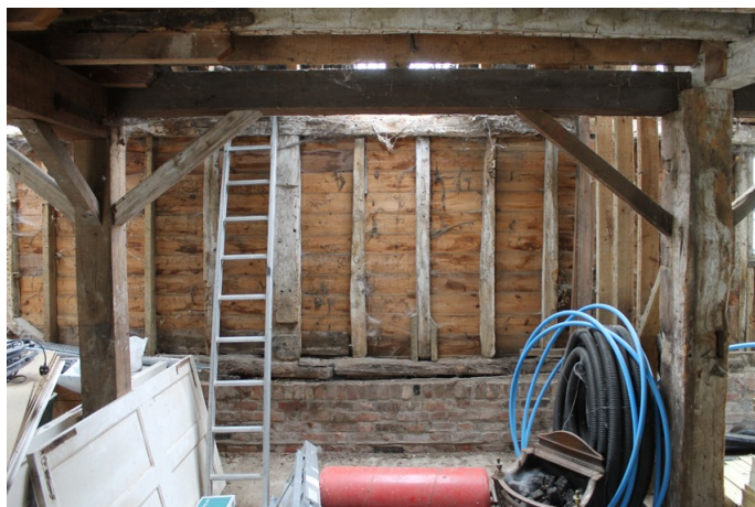
Photograph 15 Northern elevation of bay 2 on the ground-floor, showing modern girding-beam and braces. Photograph taken facing north.
