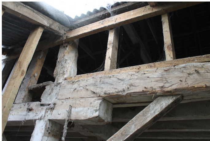
Photograph 21 Detail of girding-beam of bay 3 sitting on top of bay 4's girding-beam. Photograph taken facing south-east.
