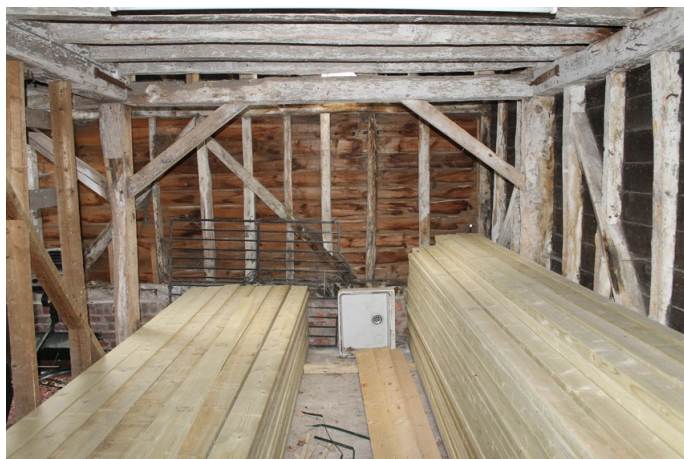
Photograph 10 Northern elevation of bay 5, showing open lower register leading into lean-to and bracing supporting girding-beam. Photograph taken facing north.
