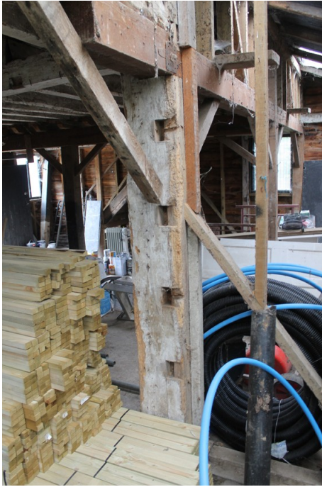
Photograph 16 Detail of re-used northern principal-post between bays 2 and 3, showing mortices. Photograph taken facing south-west.
