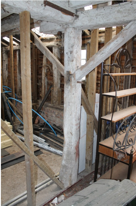
Photograph 23 Detail of principal-post between bays 3 and 4, showing empty mortice on southern face. Photograph taken facing north-west.
