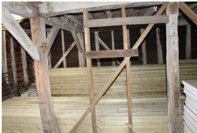
Photograph 9 Detail of original posts and modern additions supporting binding-beam between bays 3 and 4. Photograph taken facing east.
