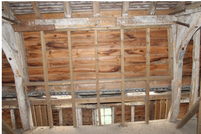
Photograph 20 Northern elevation of first-floor of bay 3, showing wall-plate and scarf joints. Photograph taken facing north.
