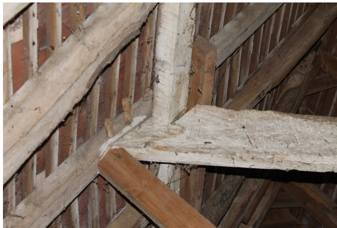
Photograph 24 Carpenter's mark 'II' on southern end of collar between bays 3 and 4. Photograph taken facing south-west.
