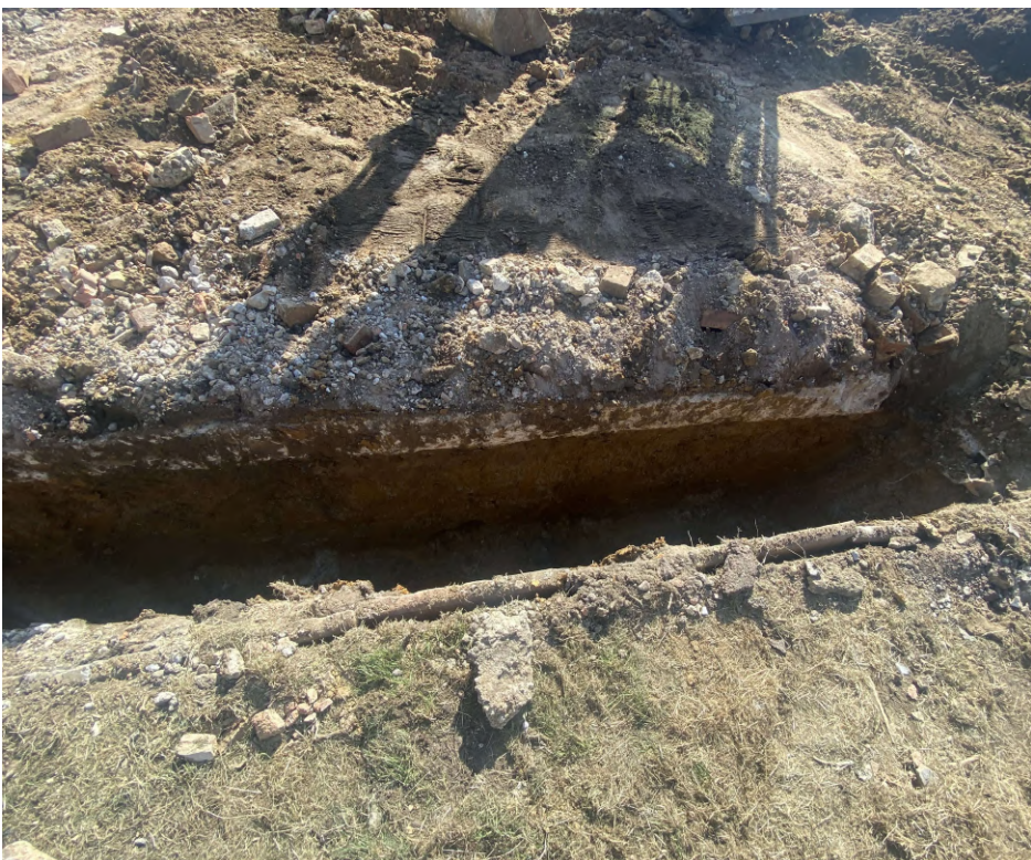
Photograph 4 Excavation of footings on north-west side of property, showing concrete footings of former garage, looking west
