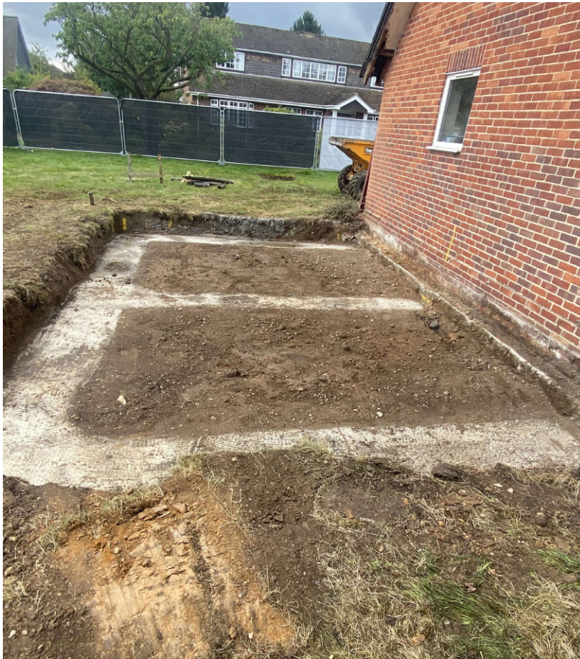
Photograph 2 Completed excavation of footings on south-east side of property, with concrete, looking south
