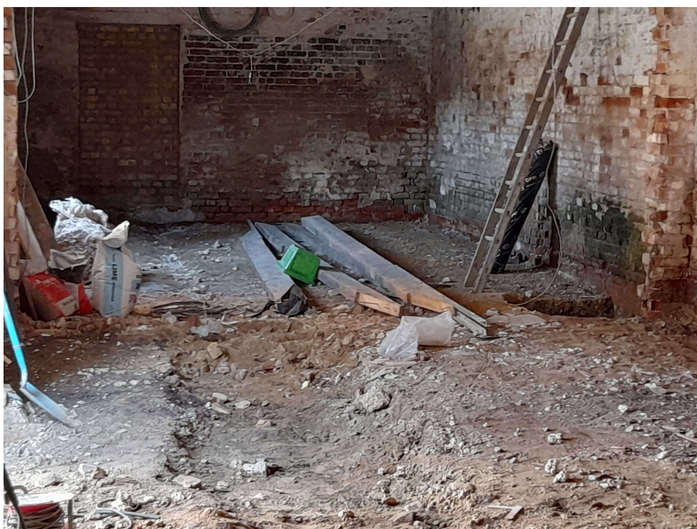
Photograph 2 View of north end of building, showing excavated area on right hand side.
