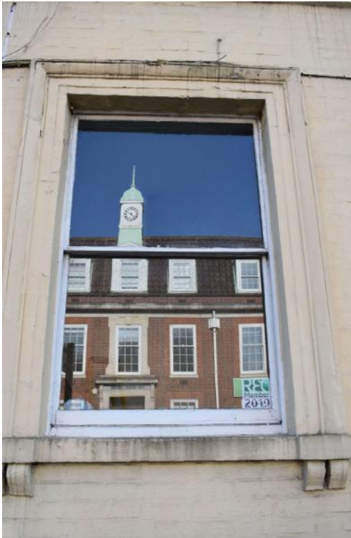
Photograph 2 Detail of window on north-west elevation of no 63 (ground floor). Photograph taken facing north-west.
