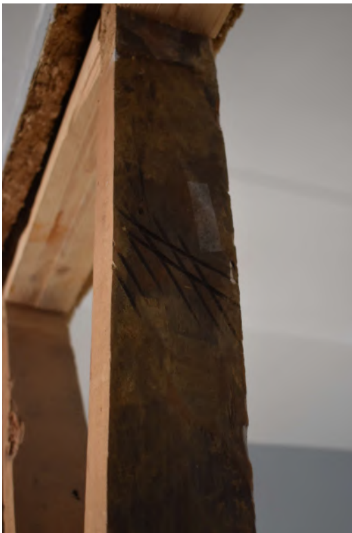
Photograph 18 Detail of Baltic Timber marks in stud wall of room 16 and 17 (1st floor of no 63). Photograph taken facing east.
