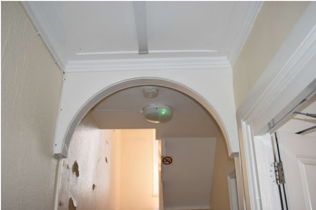
Photograph 14 Detail of original timber arch in room 11 (ground floor of no 63). Photograph taken facing south-east.
