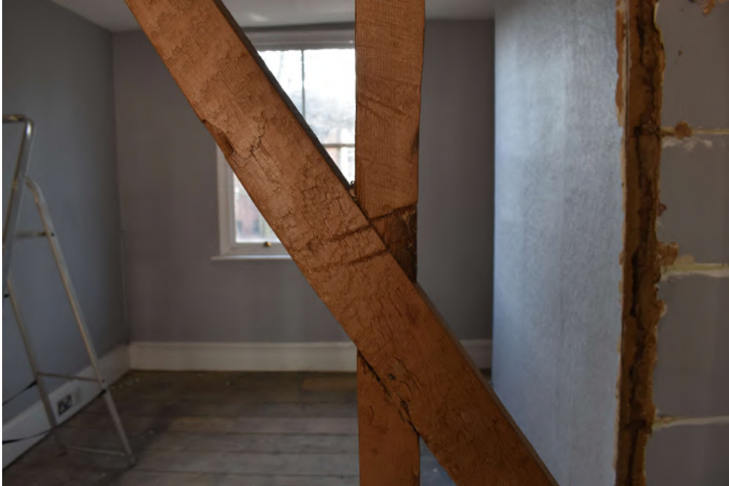
Photograph 17 Detail of carpenters marks 'II' on stud and brace of stud wall of room 16 and 17 (1st floor of no 63). Photograph taken facing south-east.
