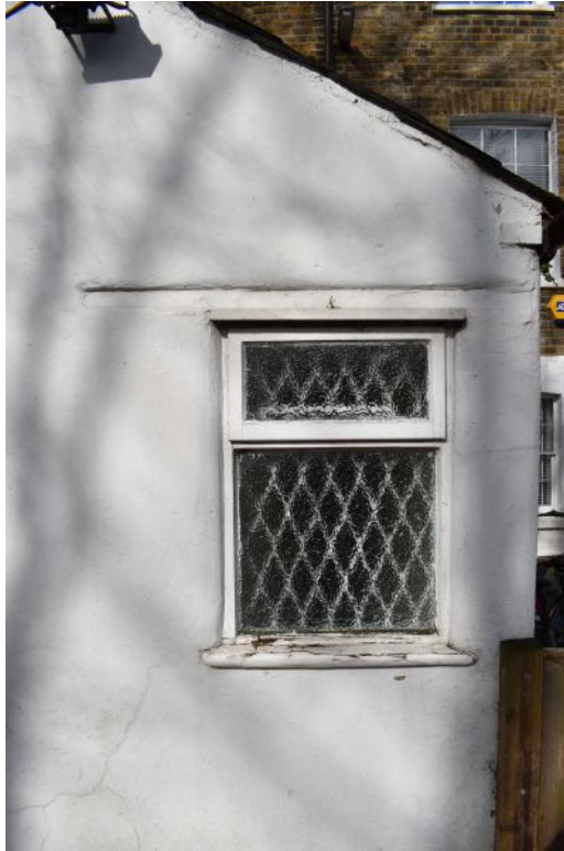
Photograph 8 Detail of window on south-east elevation (ground floor of no 63). Photograph taken facing north-west.
