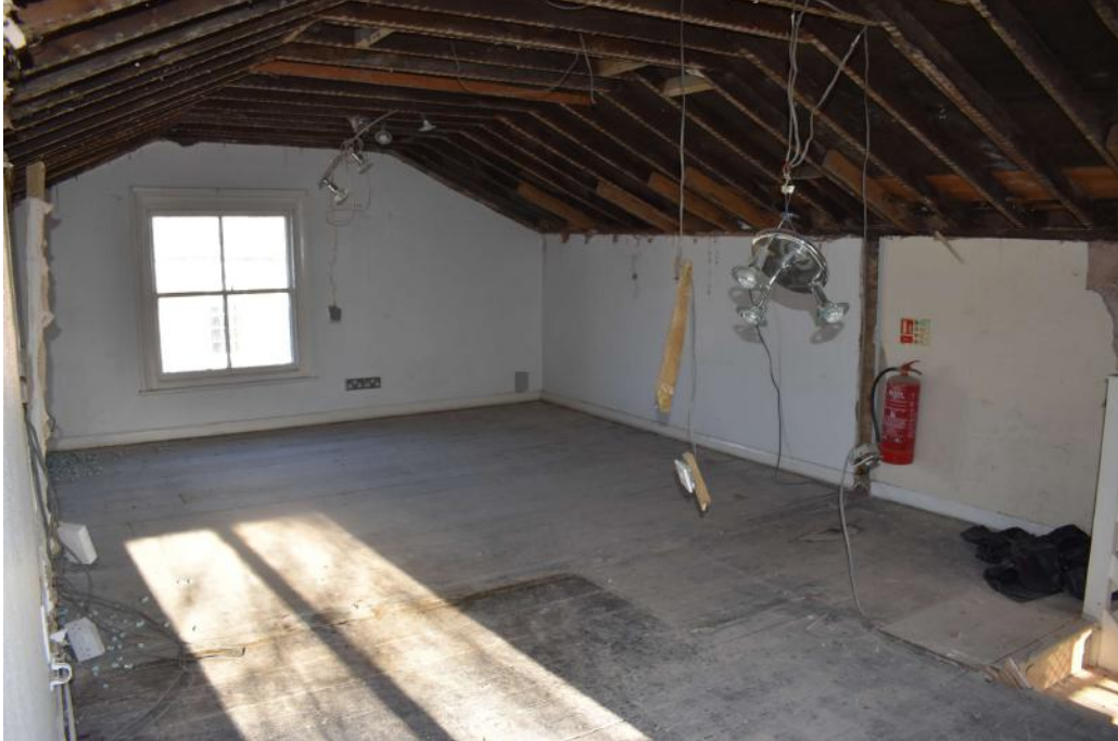
Photograph 22 Interior shot of room 19 (2nd floor of no 63). Photograph taken facing north.
