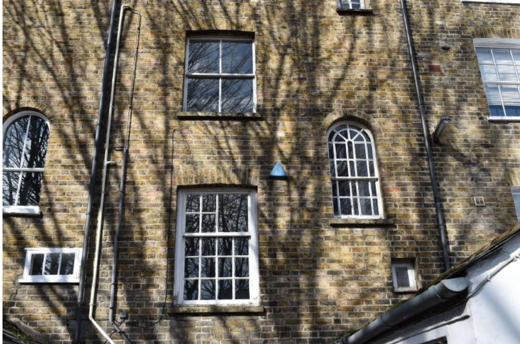
Photograph 6 Detail of windows on south-east elevation (ground and first floor of no 63). Photograph taken facing north-west.
