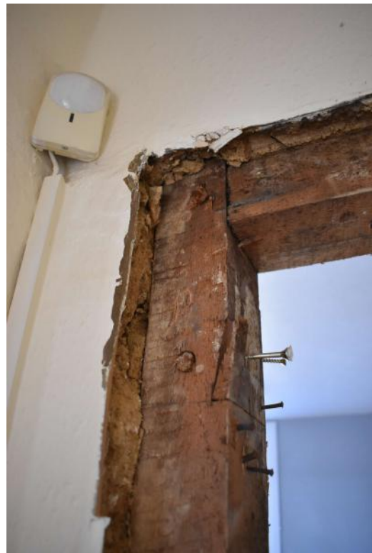
Photograph 19 Detail of timber pegs in doorway in room 17 (1st floor of no 63). Photograph taken facing south-east.
