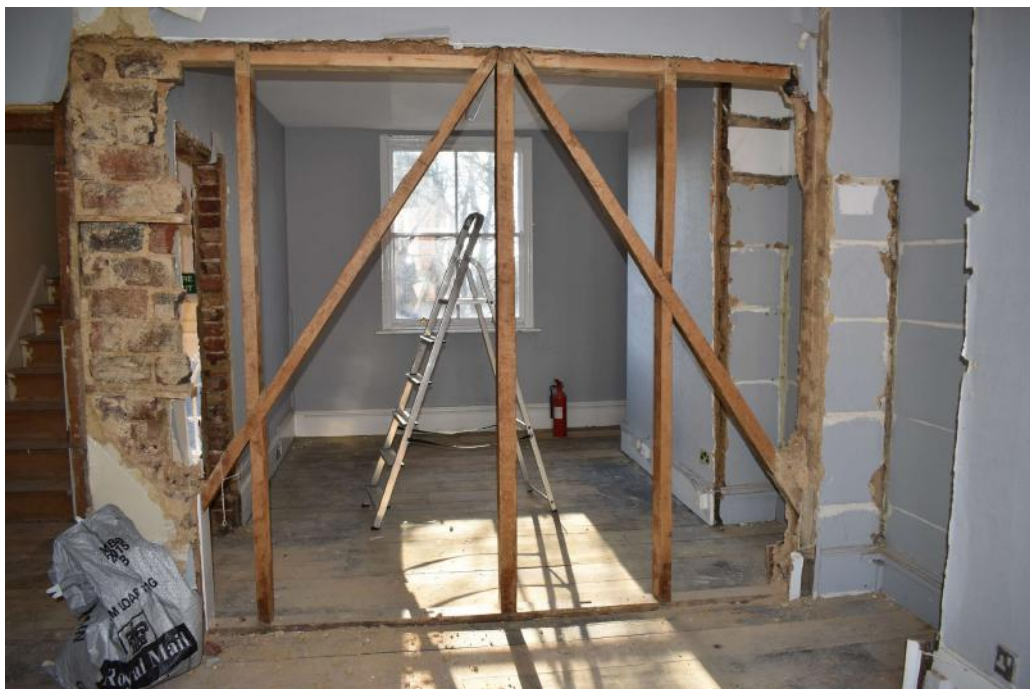
Photograph 16 Detail of stud wall between room 16 and 17 (1st floor of no 63). Photograph taken facing south-east.
