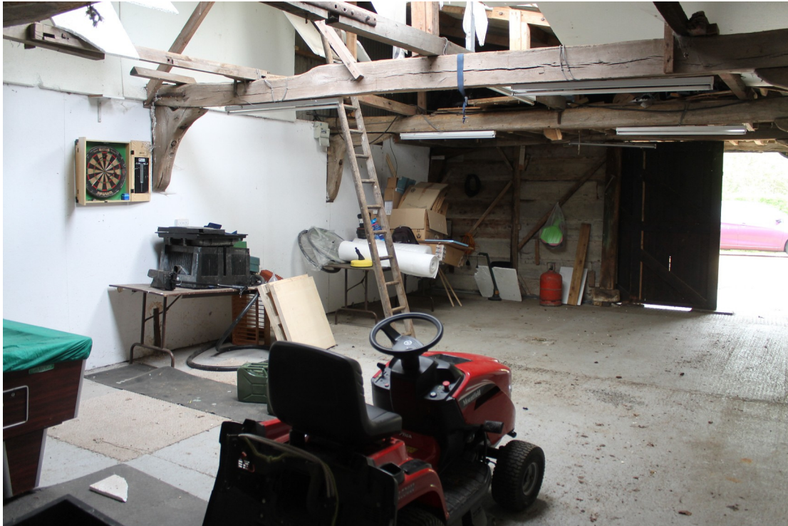
Photograph 13 Inserted loft above bays B4 and B5, accessible only by ladder – view north-east.
