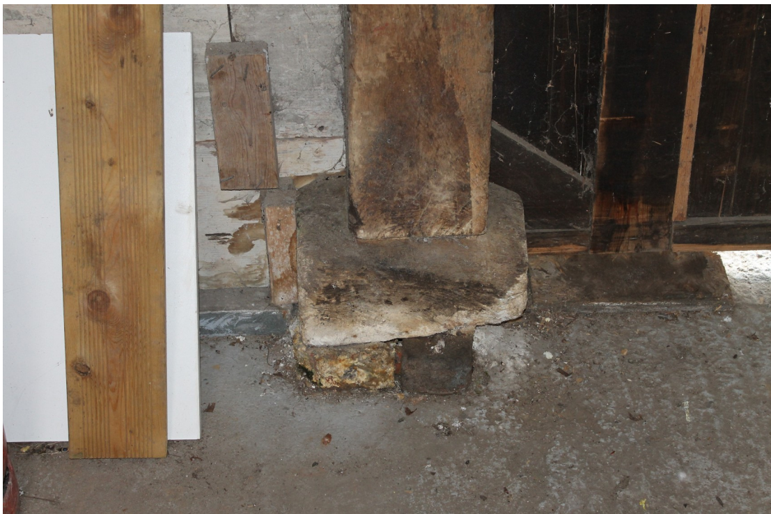
Photograph 15 Inserted post below tie-beam T4 providing support for the loft, with a timber pillow carried on bricks – view east.
