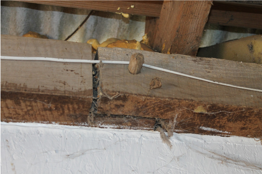
Photograph 7 Face-halved and single-pegged scarf joint in the wall plate of the south wall.
