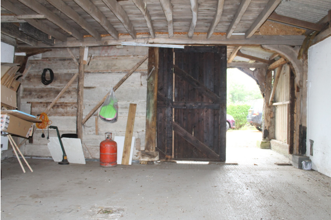
Photograph 9 Inserted dividing wall between bays B4 and B5 with the loft above.
