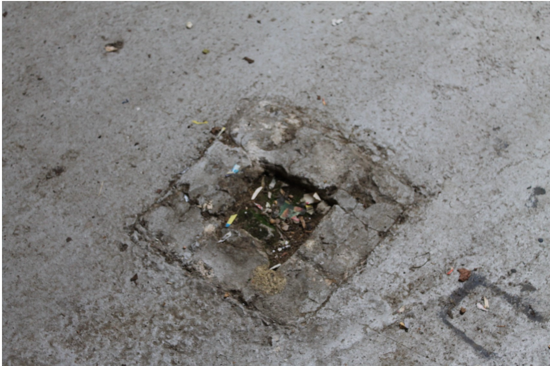
Photograph 14 Scar in the concrete floor from the removal of the inserted post below tie-beam T3, which provided support for the loft.
