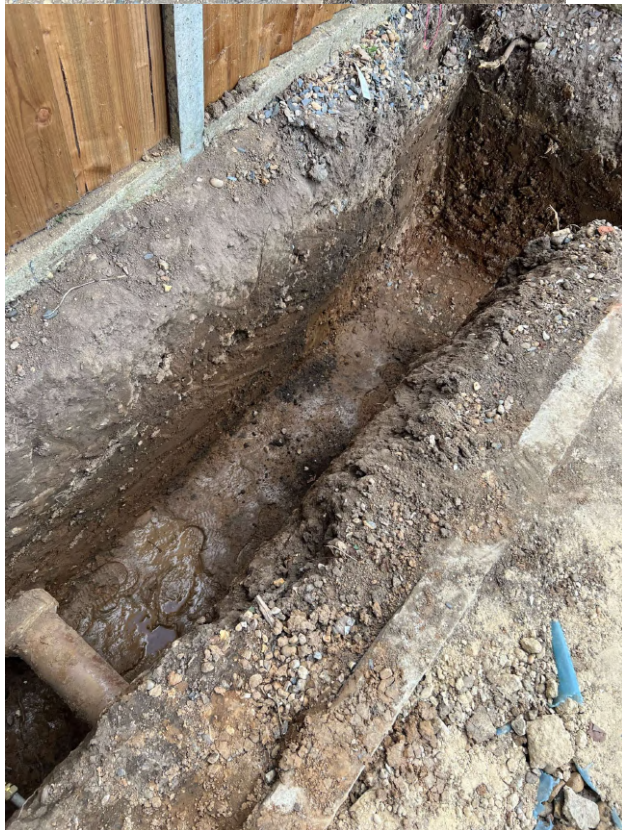
Photograph 4 Unsupervised foundation trenches, image supplied by the homeowner
