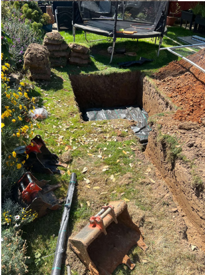
Photograph 6 Unsupervised soakaway, image supplied by the homeowner
