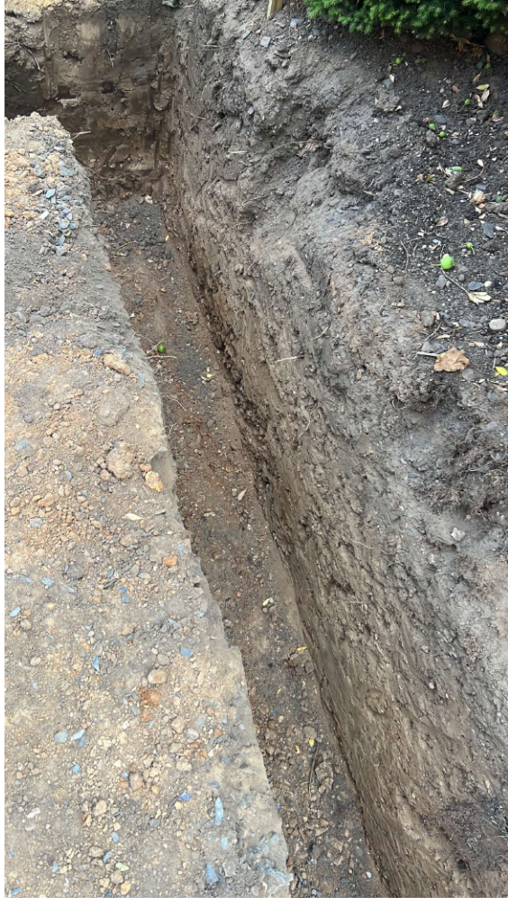
Photograph 3 Unsupervised foundation trenches, image supplied by the homeowner
