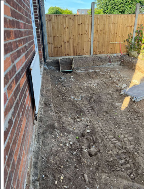
Photograph 5 Unsupervised ground reduction area inside of foundations, image supplied by the homeowner
