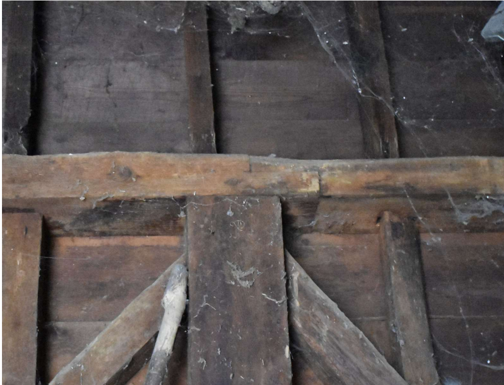
Photograph 15 Detail of scarf joint in wall plate of Store 3. Photograph taken facing north-west.
