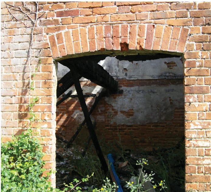
Plate 10: south elevation, east ground-floor room, showing oak bridging beam and blocked-in window.
