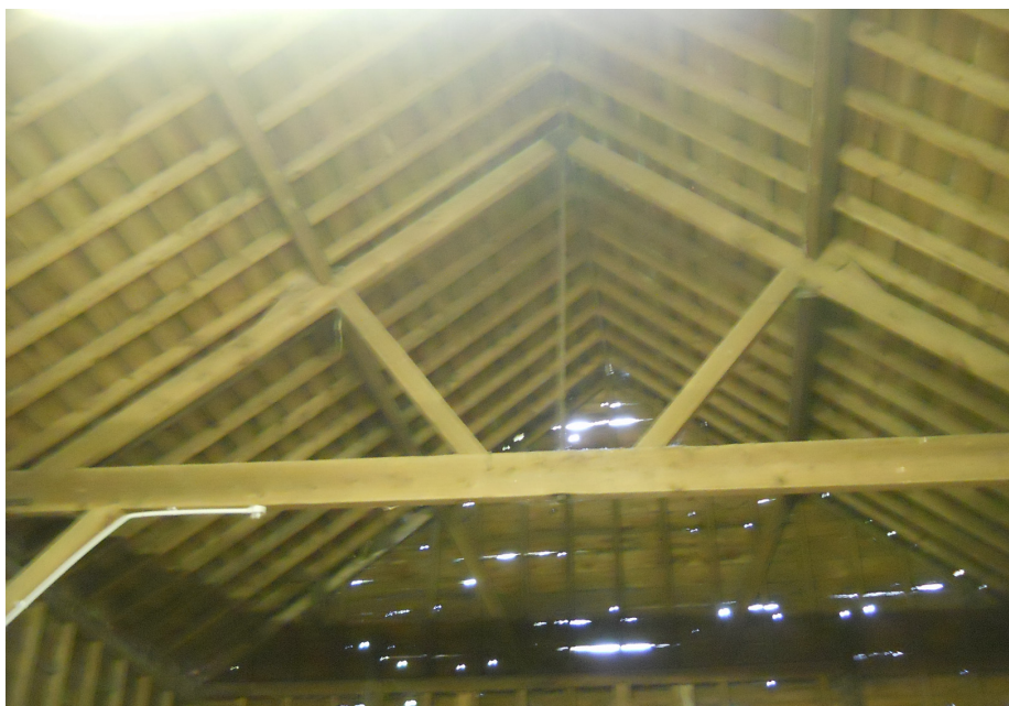
Plate 10 Large barn (E), interior, roof truss with part of down brace to post.
