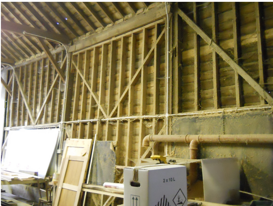
Plate 9 Large barn (E), interior, north-east wall, showing blocking of central door by matching framing.
