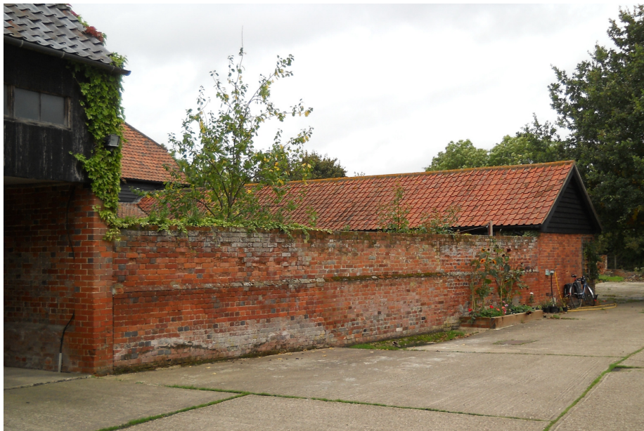
Plate 6 19th-century brick wall attached to northern corner of cart lodge/granary (M), viewed from the south-east.
