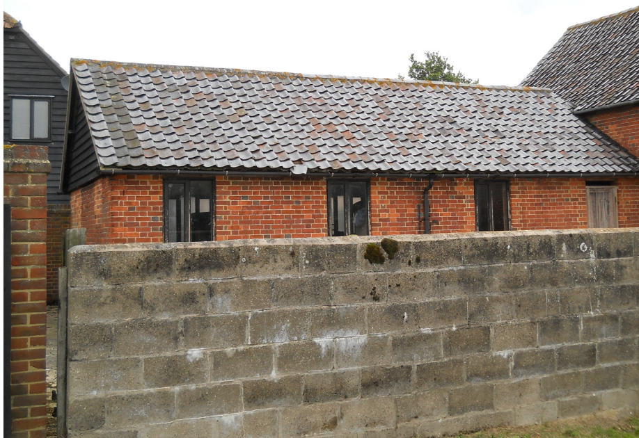
Plate 4 19th-century stable (N) attached to rear of cart lodge/granary (M), viewed from the south.
