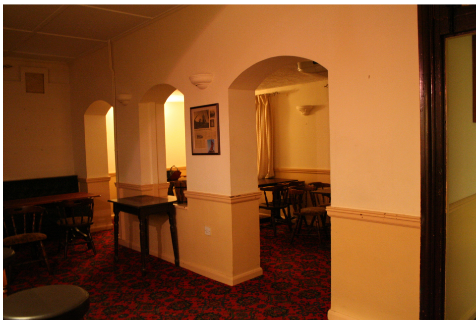
Appendix Plate 10 The extension to the lounge cut through the original west wall.
