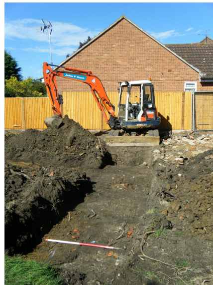
Plate 2: the north-west/south-east orientated trench showing the remains of the demolished garage, view from south-east.
