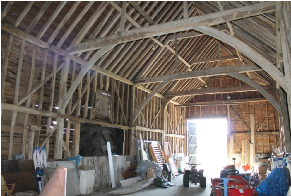
Plate 4 Interior of barn 1a showing trusses B and C with curved bracing and queen posts and truss D with knee braces – view south-east
