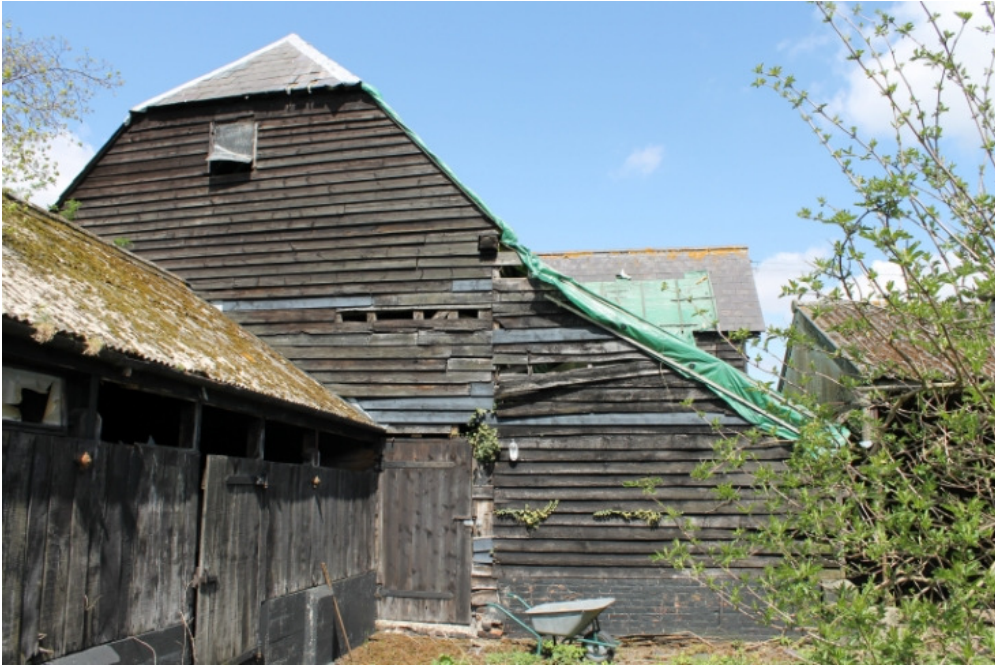
Plate 21 South elevation of barn 3a, with shelter shed 3b to the right and stable block 8 to the foreground – view north-west
