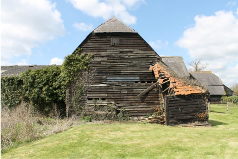
Plate 17 Outbuilding 2b at east end of barn 2a, not also the small hatch under the eaves of the barn - view west
