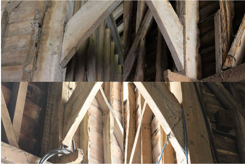
Plate 5 Carpenters' marks on posts and braces of trusses B (top) and C (bottom)
