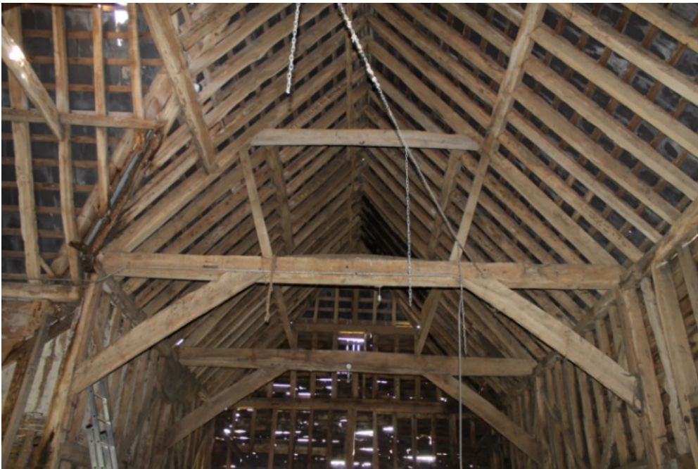
Plate 14 Barn 2a, showing truss B with lightly curved braces, inclined queen struts and joggled purlins - view east
