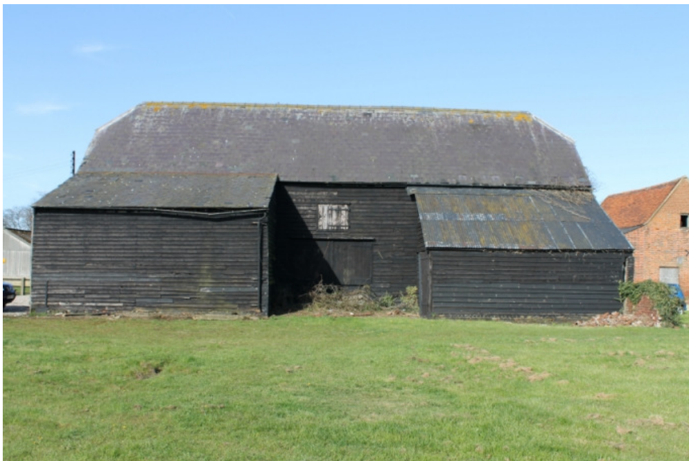
Plate 2 North-east elevation of structure 1, showing rear barn doors and pitching door of barn 1a with lean-to 1f to the left and lean-to 1e to the right – view south-west
