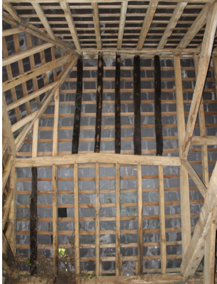
Plate 15 Barn 2a, detail of fire-blackened and reused timbers in roof of bay 1
