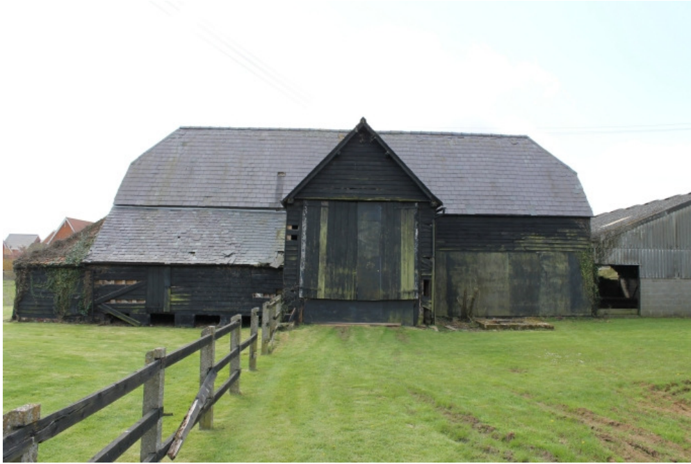
Plate 11 North elevation of structure 2, showing the threshing barn 2a and outbuilding 2b and granary 2c/d to the left of the midstrey – view south
