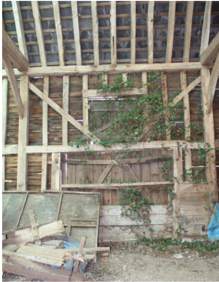
Plate 25 Barn 3a, showing rear barn doors with replacement girding beam and threshold leap – view west
