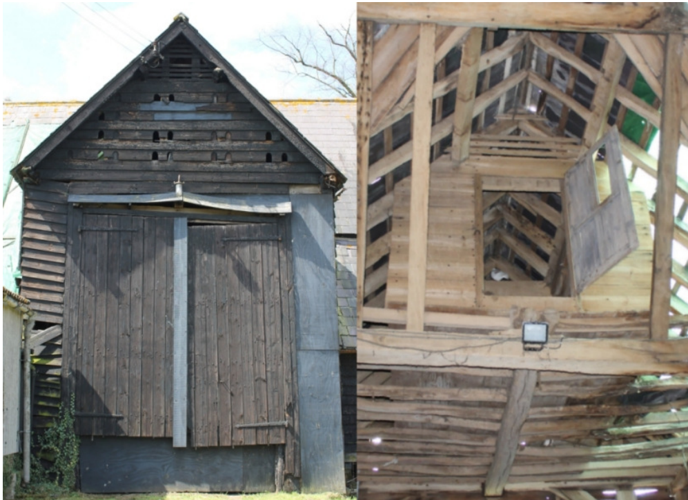
Plate 28 Barn 3a, showing exterior and interior of midstrey with pigeon loft in gable
