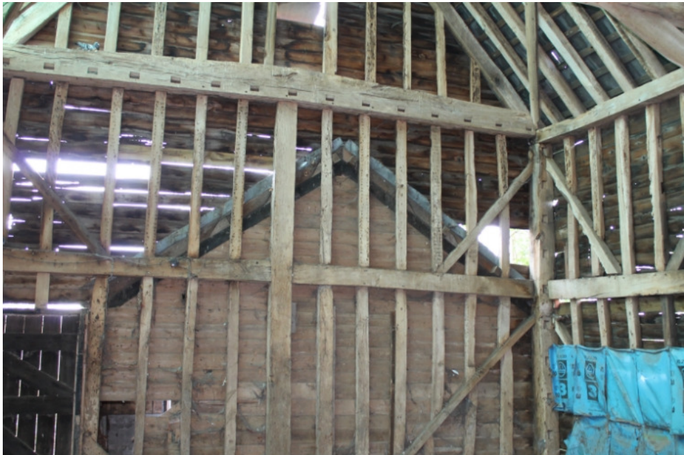
Plate 24 Barn 3a, showing the reused tie beam in place of the wall plate – view north-west
