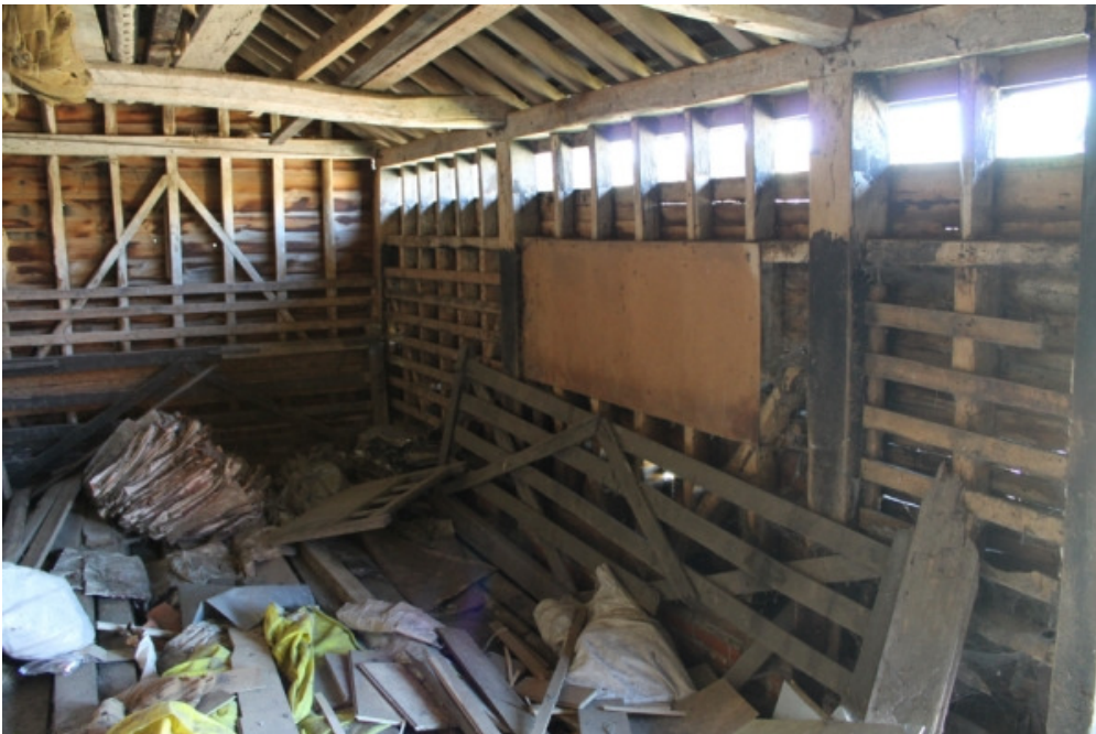
Plate 8 Interior of lean-to 1d, showing the differences between the framing of the short end and long side – view south
