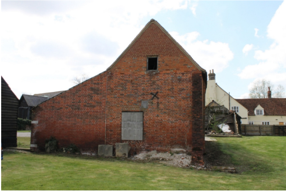
Plate 35 Stable/granary 4a, showing converted doorway, rebuilt gable and later buttress – view south-west
