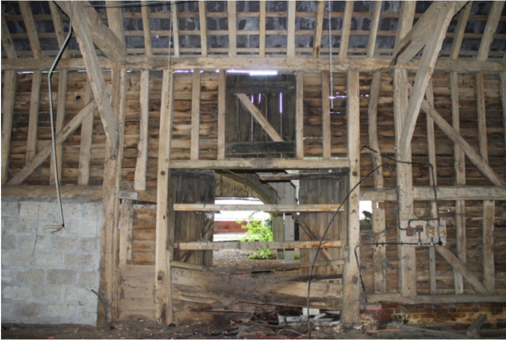
Plate 13 Barn 2a, showing jowled bases to rear barn doors, threshold leap and inserted pitching door – view south
