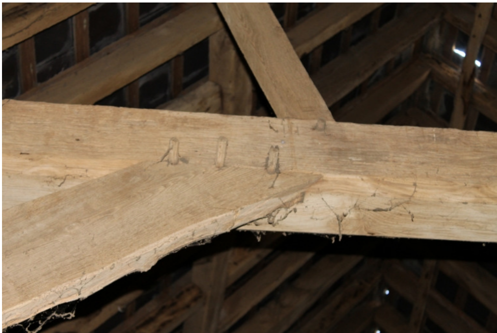
Plate 16 Barn 2a, chiselled carpenters' marks 'III' on tie beam and strut of truss C
