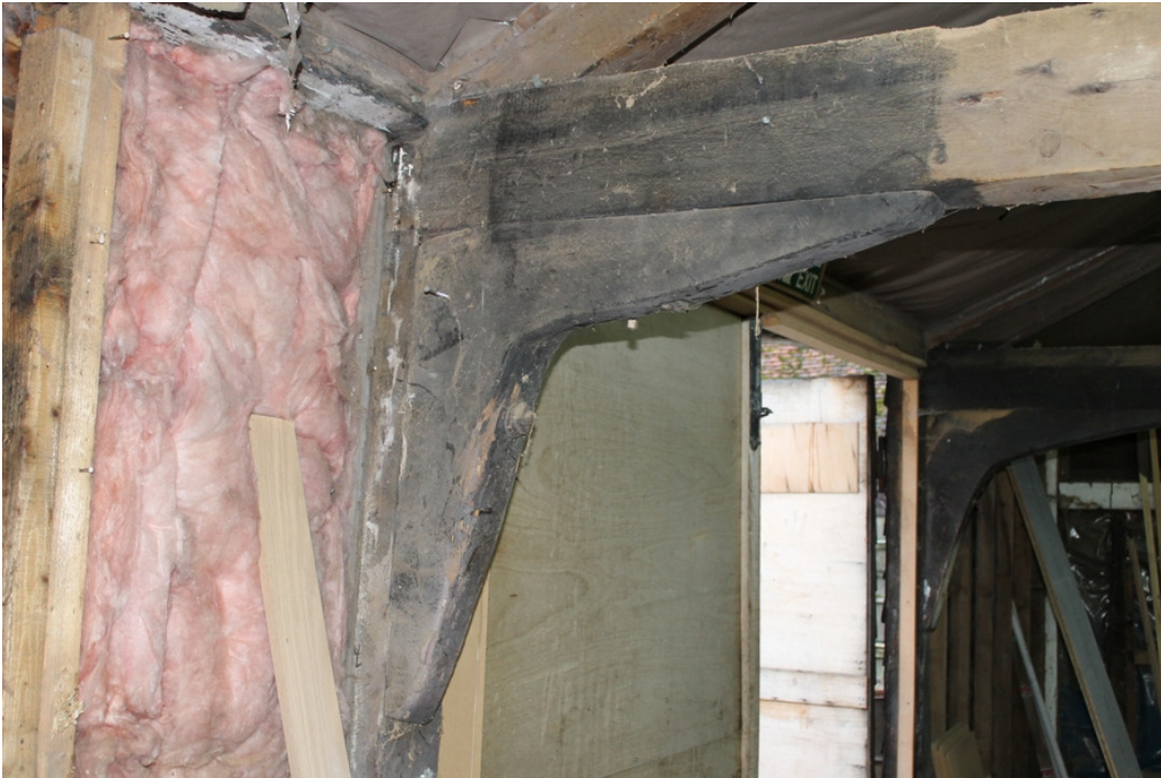
Plate 15 Knee brace to south-east post of truss A, with tie beam carried on the head of the post and the wall plate supported by the tie beam - view east
