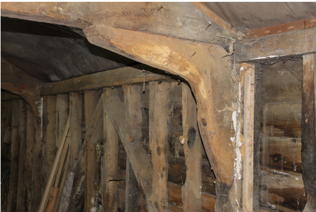
Plate 14 Knee brace to north-west post of truss A, with tie beam sitting on top of wall plate - view south-west
