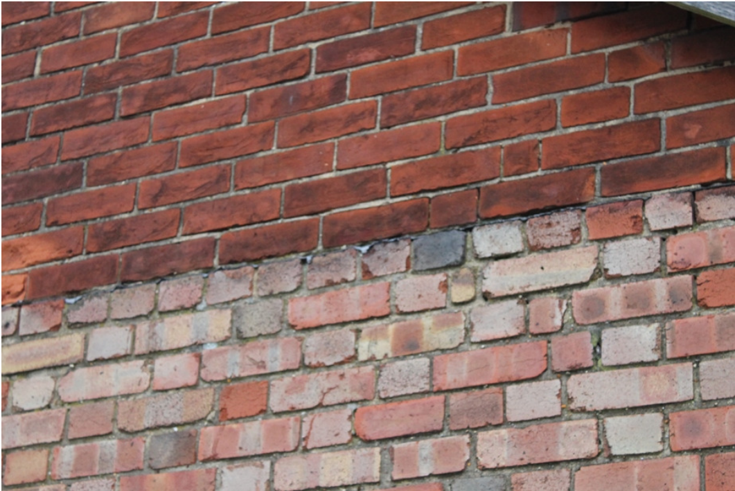
Plate 5 Remains of lead flashing between the Fletton bricks and soft reds of the gable on the south-east elevation of the brick barn, indicative of a mono-pitch lean-to - view north
