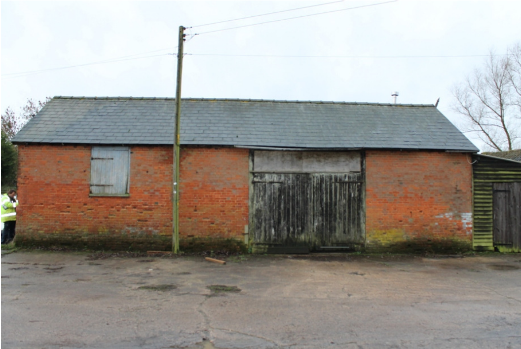
Plate 1 Brick barn at Betts Farm, north-east elevation, with ?original pitching door and later cart doors - view south-west
