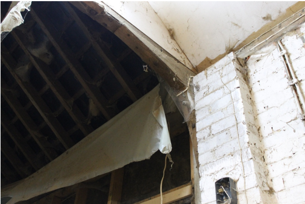
Plate 8 Bolted knee brace to truss B of bay 2 and brick pier of the wall – view north-east
