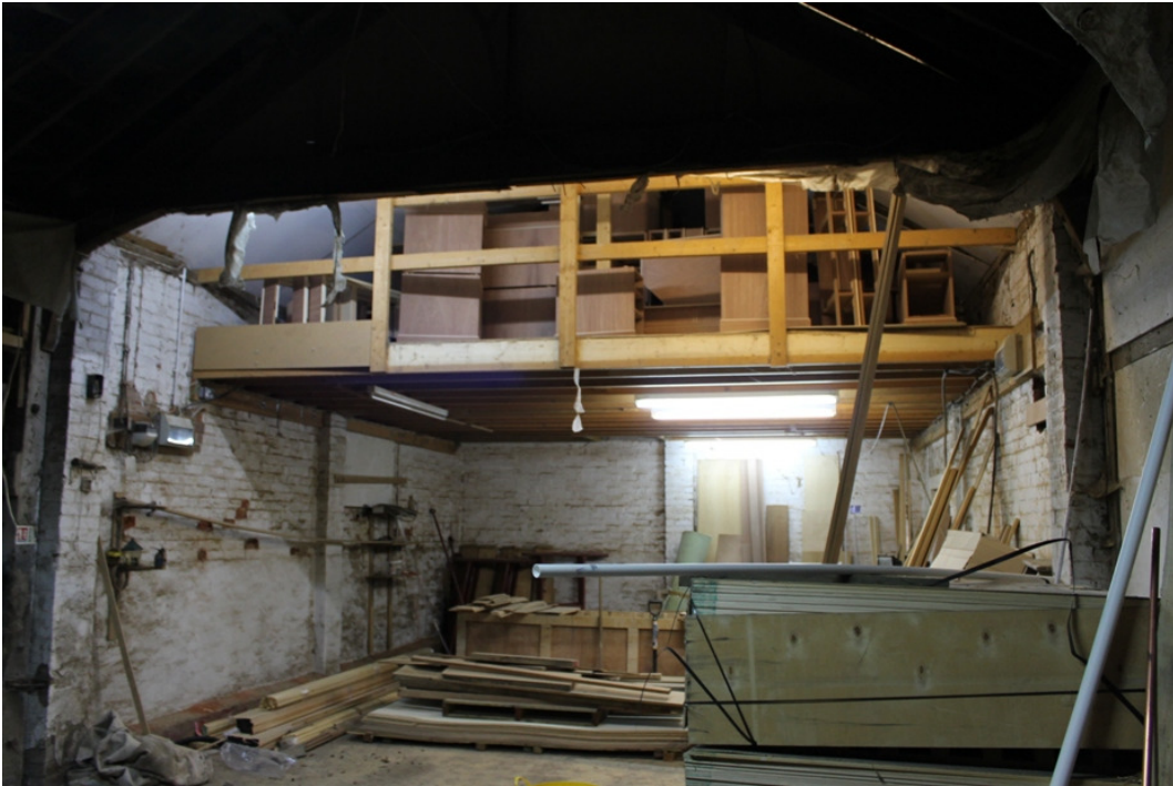
Plate 7 The interior of the brick barn, showing the modern mezzanine blocking the pitching door – view north-west
