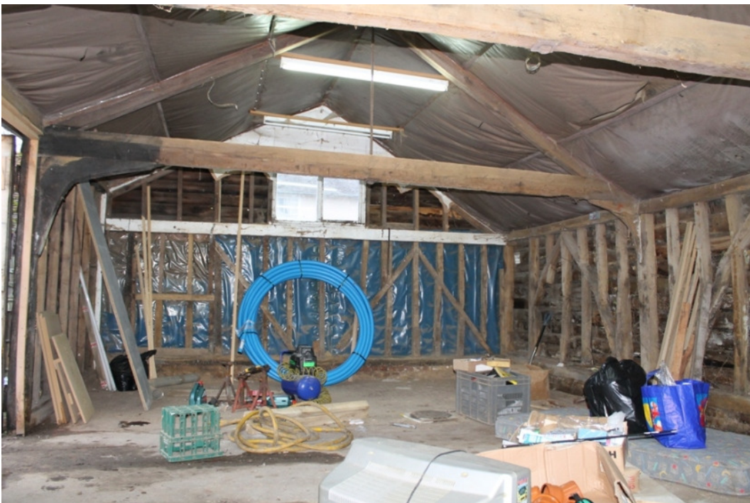
Plate 12 Interior of the converted loose boxes, with the blocked openings on the left and the rebuilt gable with the inserted casement window to the rear - view south-west
