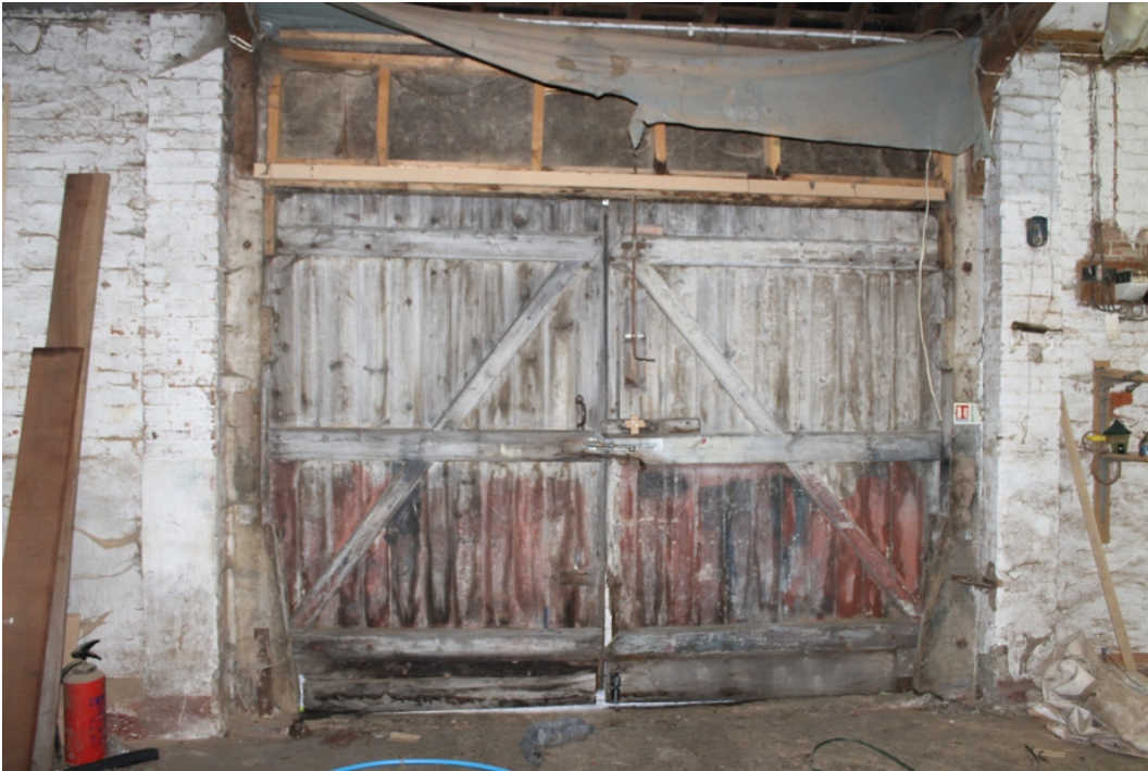
Plate 9 Bay 2 of the brick barn, showing later cart doors attached to original doorposts, sawn from single timbers and incorporating flared bases - view north-east.
