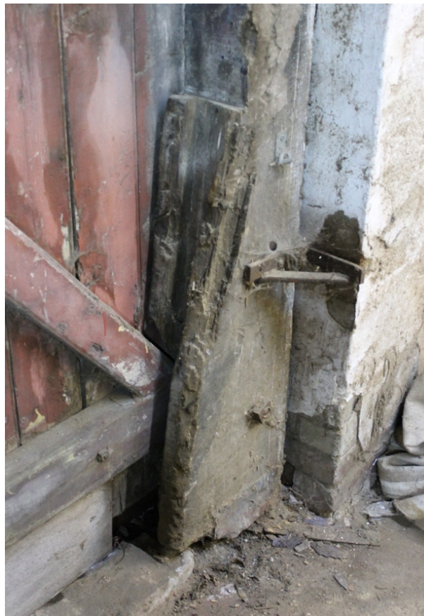
Plate 10 Flared base to truss B, with recess for threshold leap, damaged by the later cart door – view east
