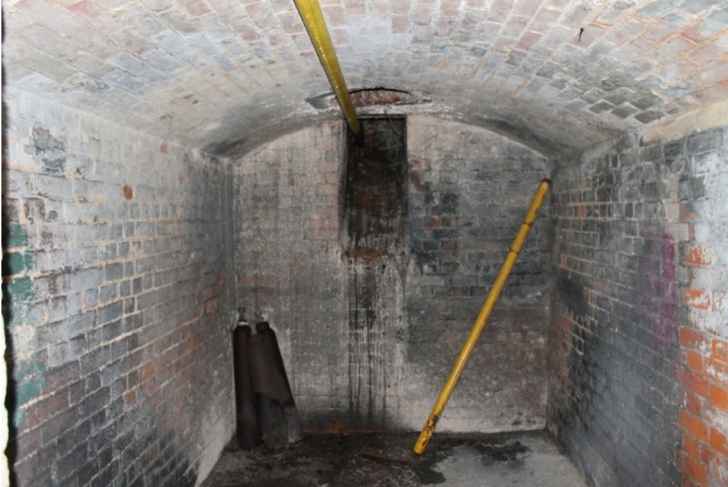
Plate 41 Room 29, the former beer cellar converted to an additional coal store, with a coal chute inserted through the rear wall and the connecting doorway to the wine cellar (in the foreground on the right) bricked in – view north-east
