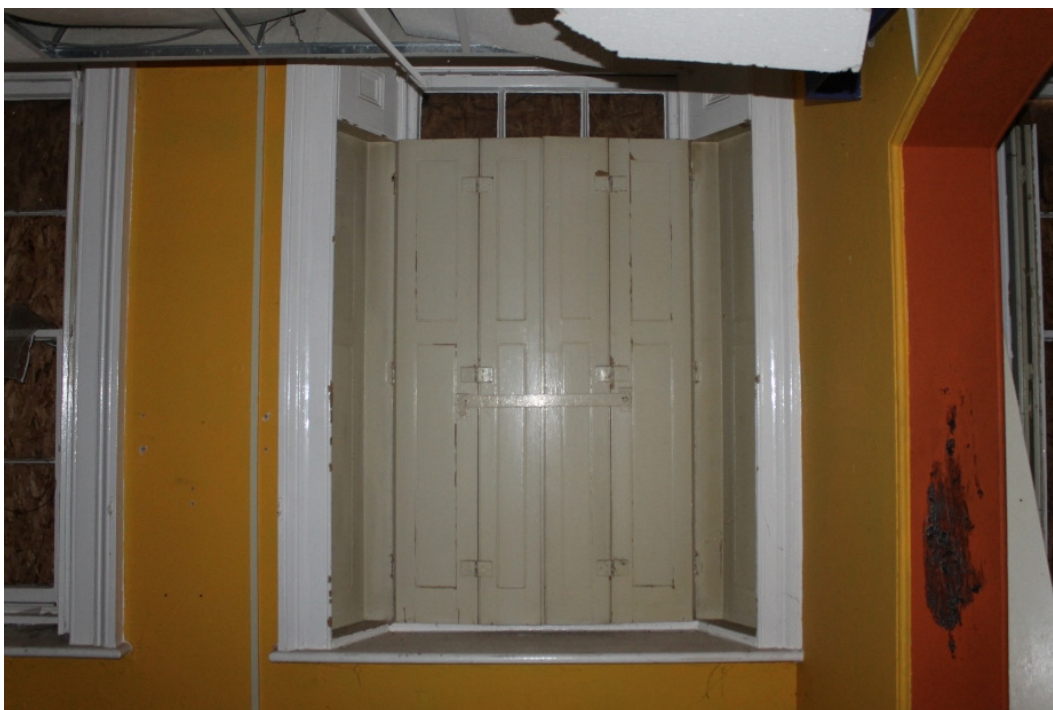
Plate 22 Example of the sash windows with recessed wooden shutters in the ground floor rooms of the 1874-5 building - view south-east
