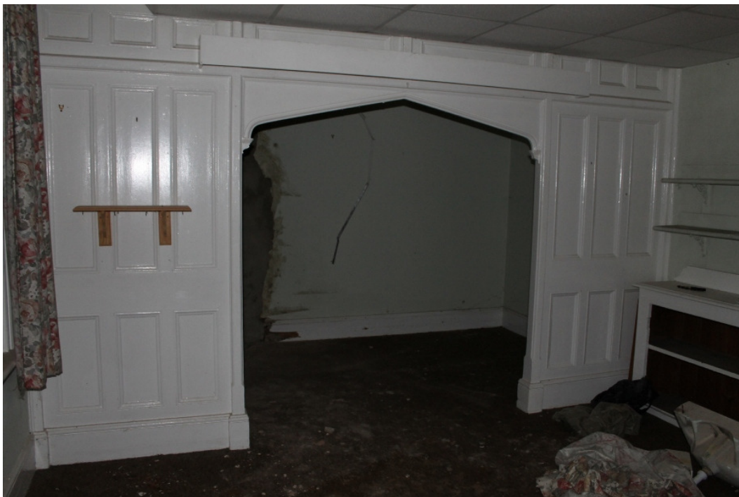
Plate 19 Original wooden partition in room 2 separating the sleeping area from the sitting room – view south-west
