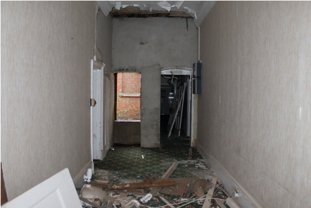
Plate 17 Entrance way iii with the removed staircase and the 1904 toilet block to the rear - view north-west
