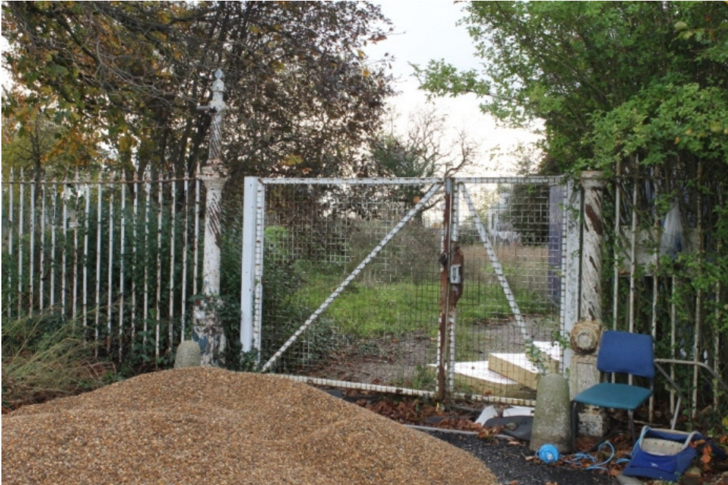
Plate 13 The 1904 railings and barley twist gate posts with integrated gas lamps – view east
