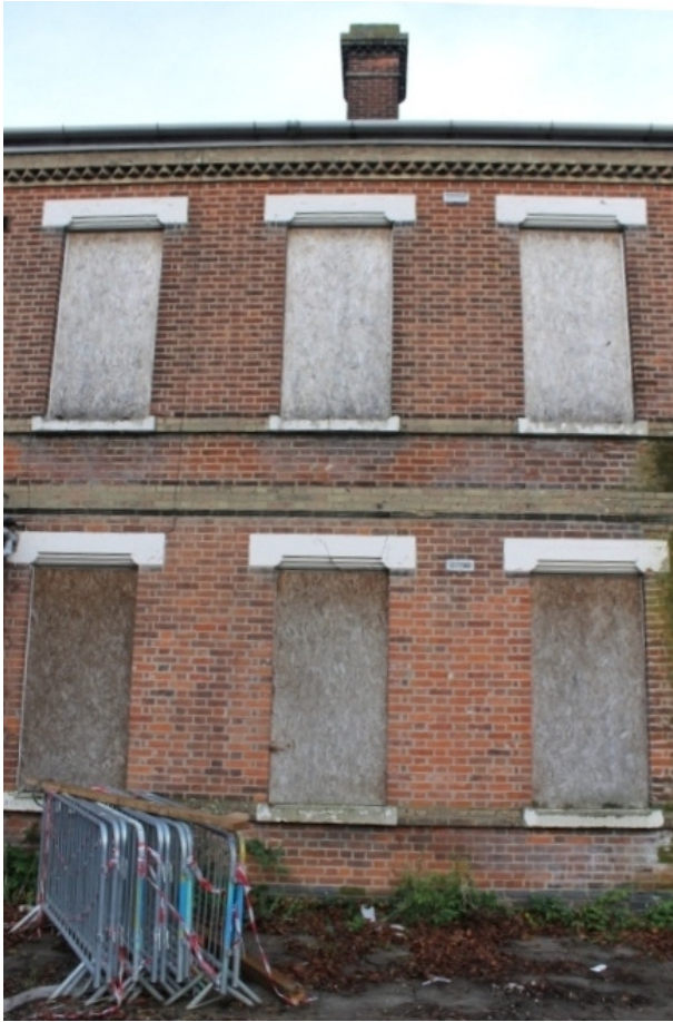
Plate 1 Section of the south-east elevation, showing the windows with their cast lintels and sills and the decorative cornice and string lines of yellow stock brick - view north-west
