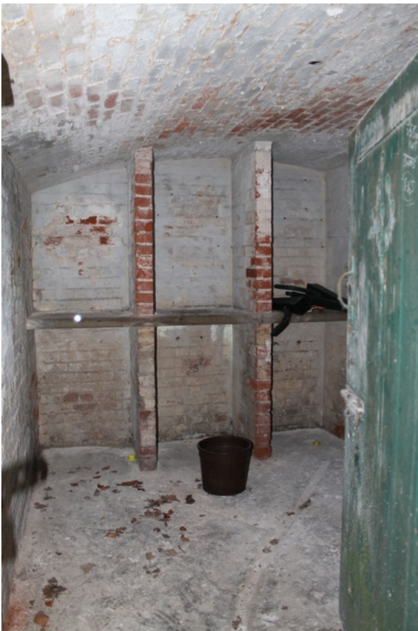
Plate 42 Room 30, the wine cellar viewed through the inserted doorway, with the original sandstone shelves and drainage channel cut into the concrete floor – view north-east
