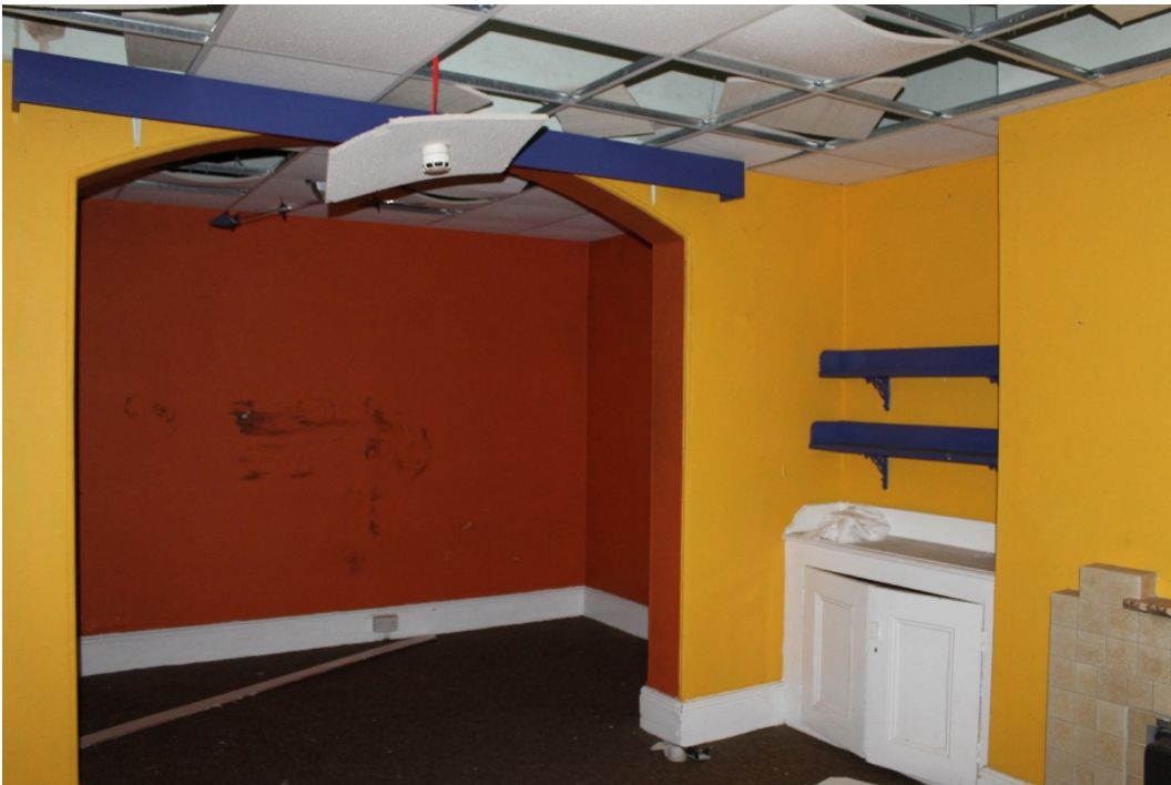
Plate 24 Room 7, formerly the quarters for Officer No.1, showing the brick arch separating the sleeping area from the sitting room, with the original dresser and shelving to the left of the chimney breast – view south
