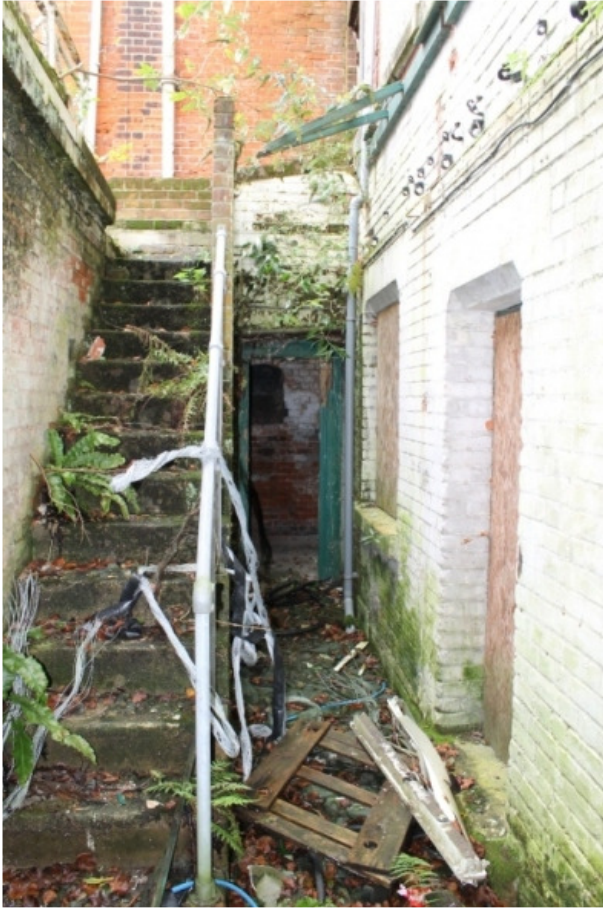
Plate 39 Stairwell vi, leading from the basement kitchen and underground storage area to the yards at the rear of the building: the original coal store is visible at the end of the passage – view north-east
