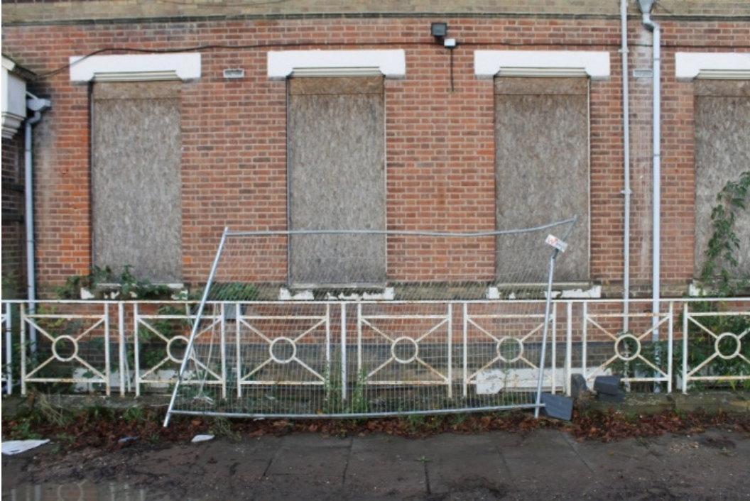
Plate 3 Original railings to the light-well on the south-east elevation - view north-west
