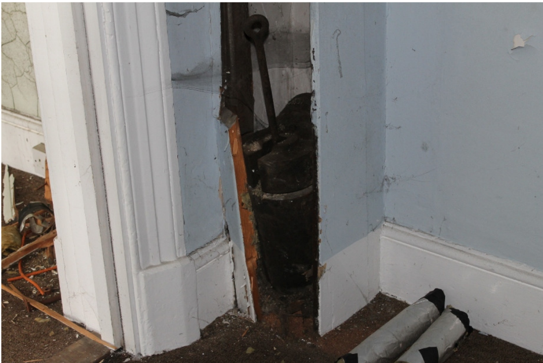
Plate 32 One of the original counter-balances for the food lift, located in the corner of room 18 – view north-east
