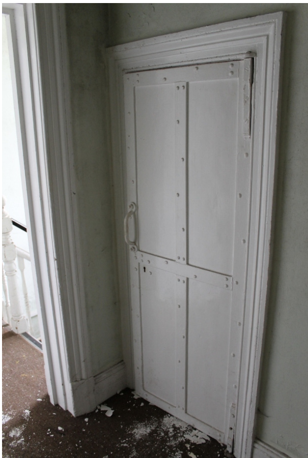
Plate 33 Iron door to strongroom 20, converted from the former servants' quarters for Officers Nos.2 and 3 - view west
