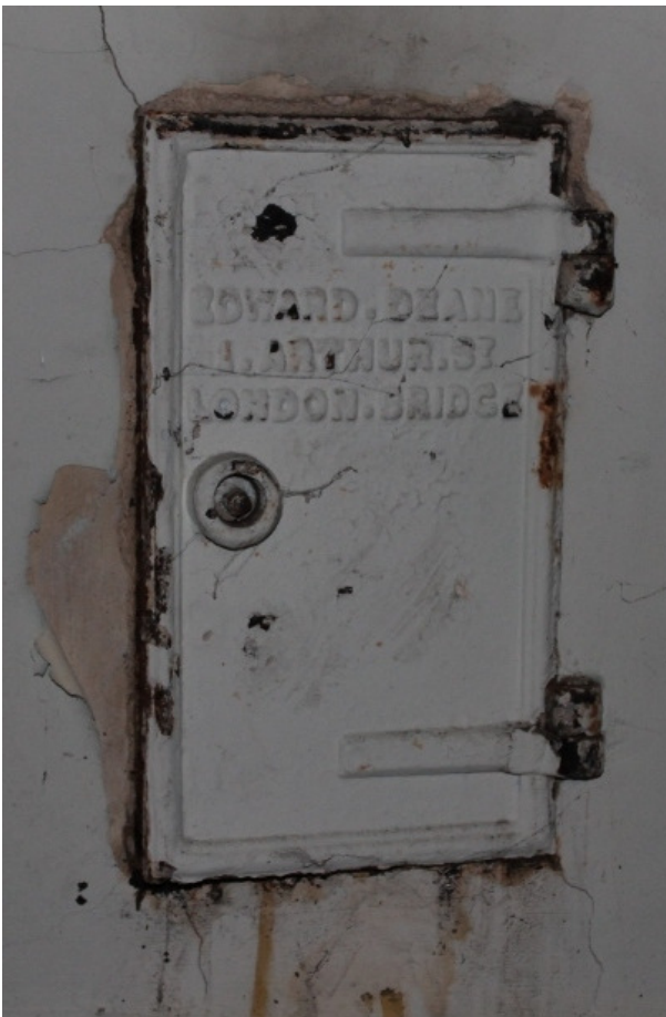
Plate 36 Detail of the original soot door in the first floor wall of stairwell iii
