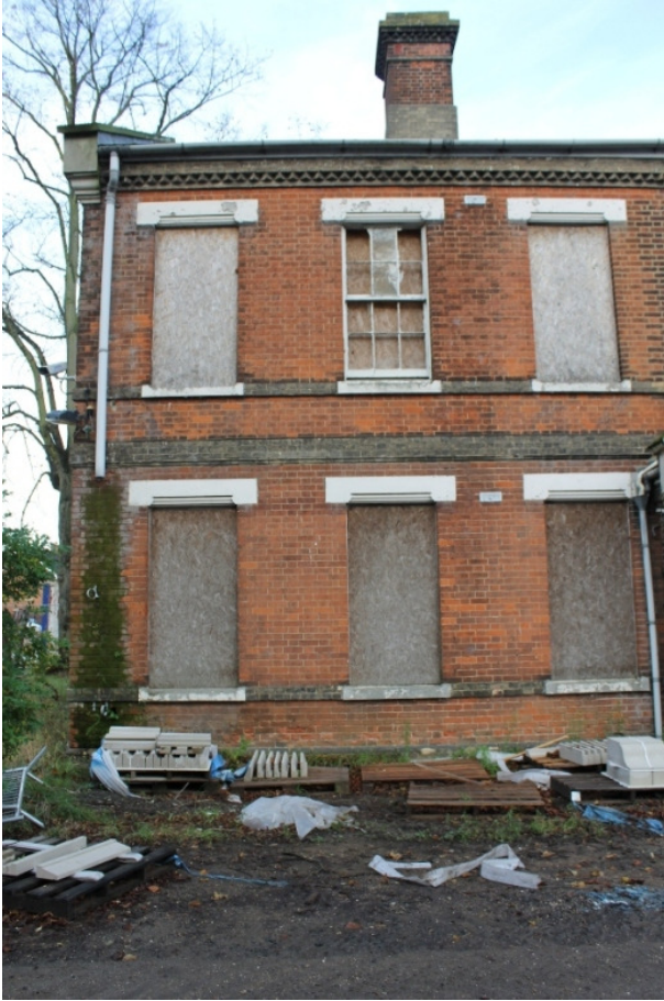
Plate 9 South-east elevation of the 1904 extension to the Officers' Quarters, showing the continuation of the architectural embellishments; the change in the brickwork is visible in the top right of the photograph - view north-west
