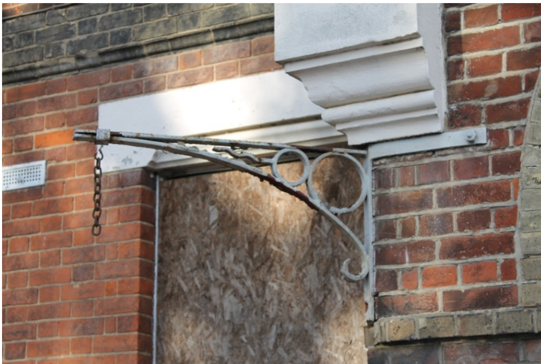
Plate 6 Detail of the iron bracket and chain for the original gas lamp on the corner of entrance way i
