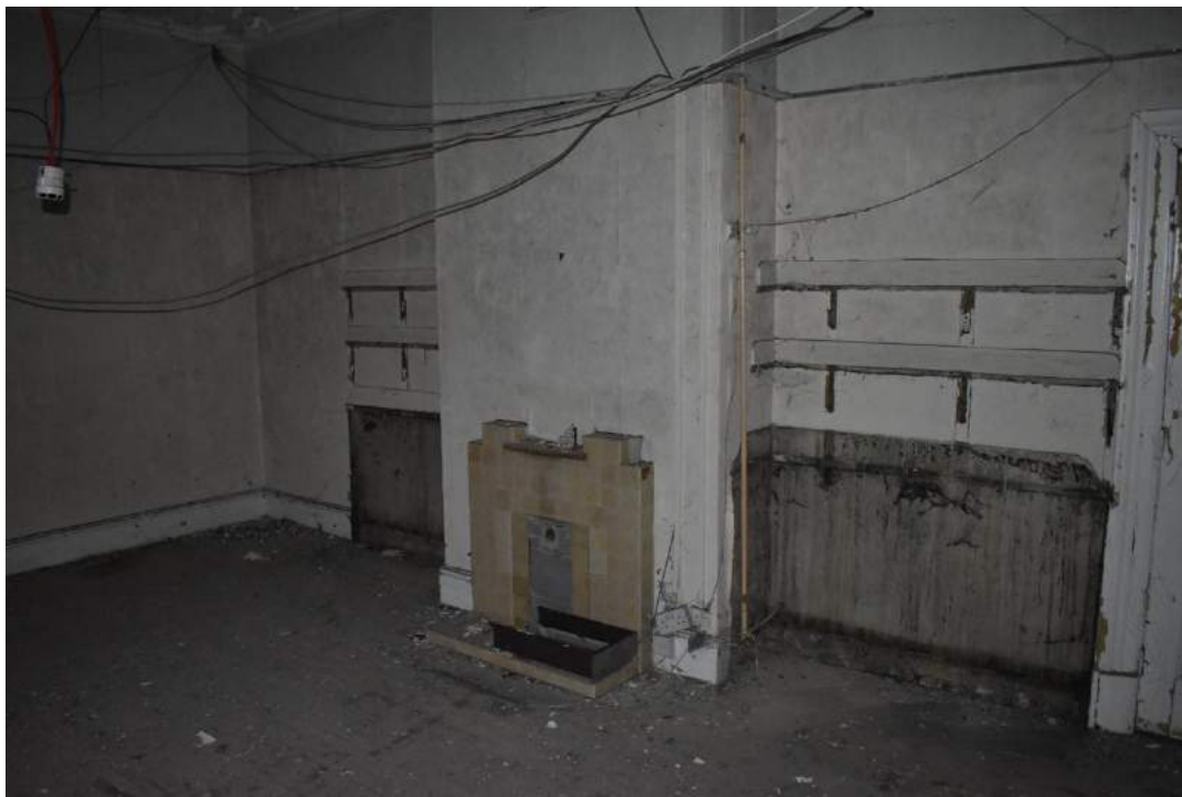
Plate 8 Room 4, formerly the sitting room of the second Field Officer, with the original four-panel door leading to the bedroom of said officer – view west. Photo from November 2013 above, photo from December 2019 below.
