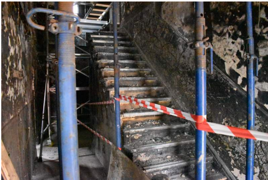
Plate 2 Stairwell iv , showing the original staircase, coat hooks and the entrance to the 1904 lavatory – view north-west. Photo from November 2013 above, photo from December 2019 below.
