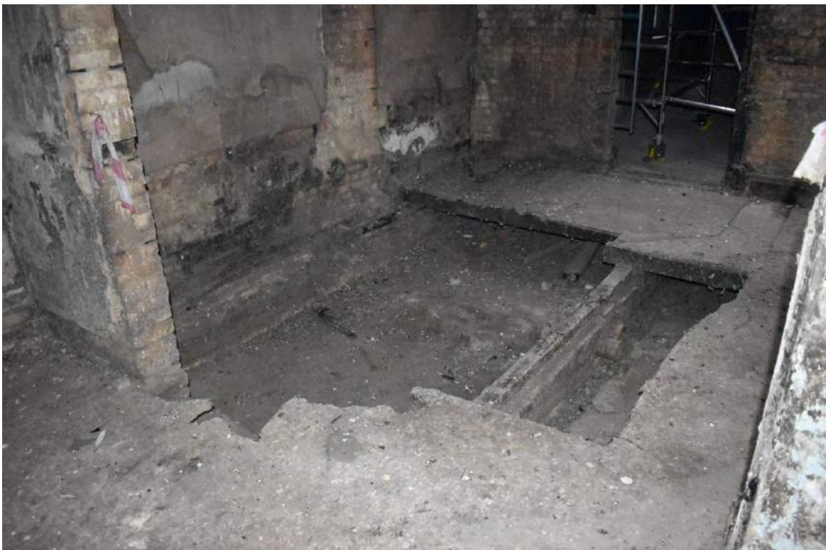
Plate 24 Missing floor in ground-floor on building below room 24, with exposed brick plinths - view north.
