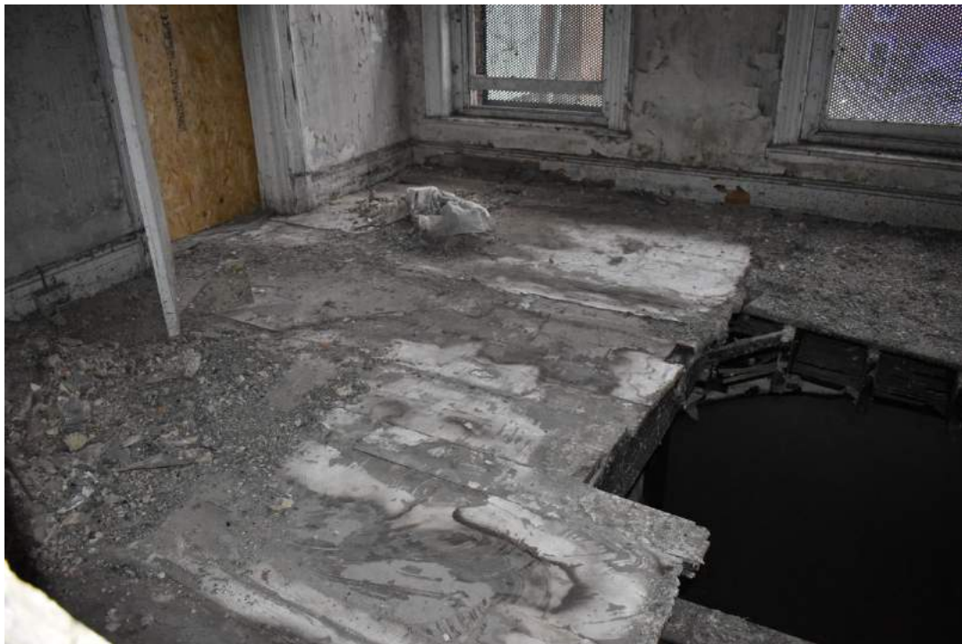
Plate 20 Room 22, formerly the quarters for Officer No.9, showing the relocated doorway and fireplace – view south-west. Photo from November 2013 above, photo from December 2019 below.
