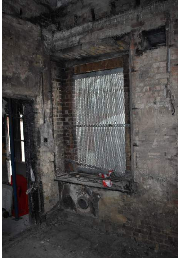
Plate 23 Detail of window opening on ground-floor of building below room 25, showing complete destruction of window-frame by fire – view east.
