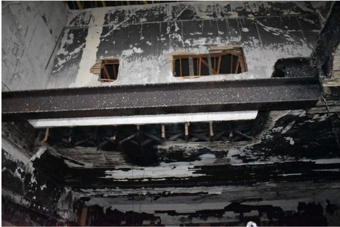
Plate 25 Metal beam that would have supported the floor of room 22 prior to the fire. Herringbone strutting visible behind - view south-east.
