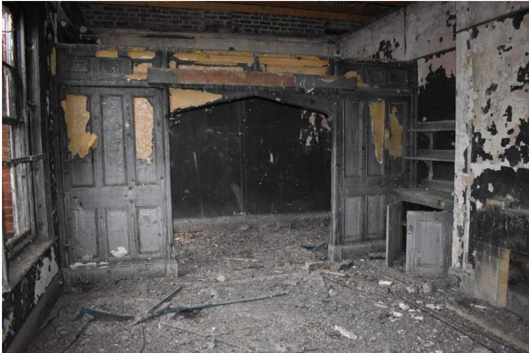
Plate 31 Interior of room 26 showing surviving, but damaged, features - view north-east.
