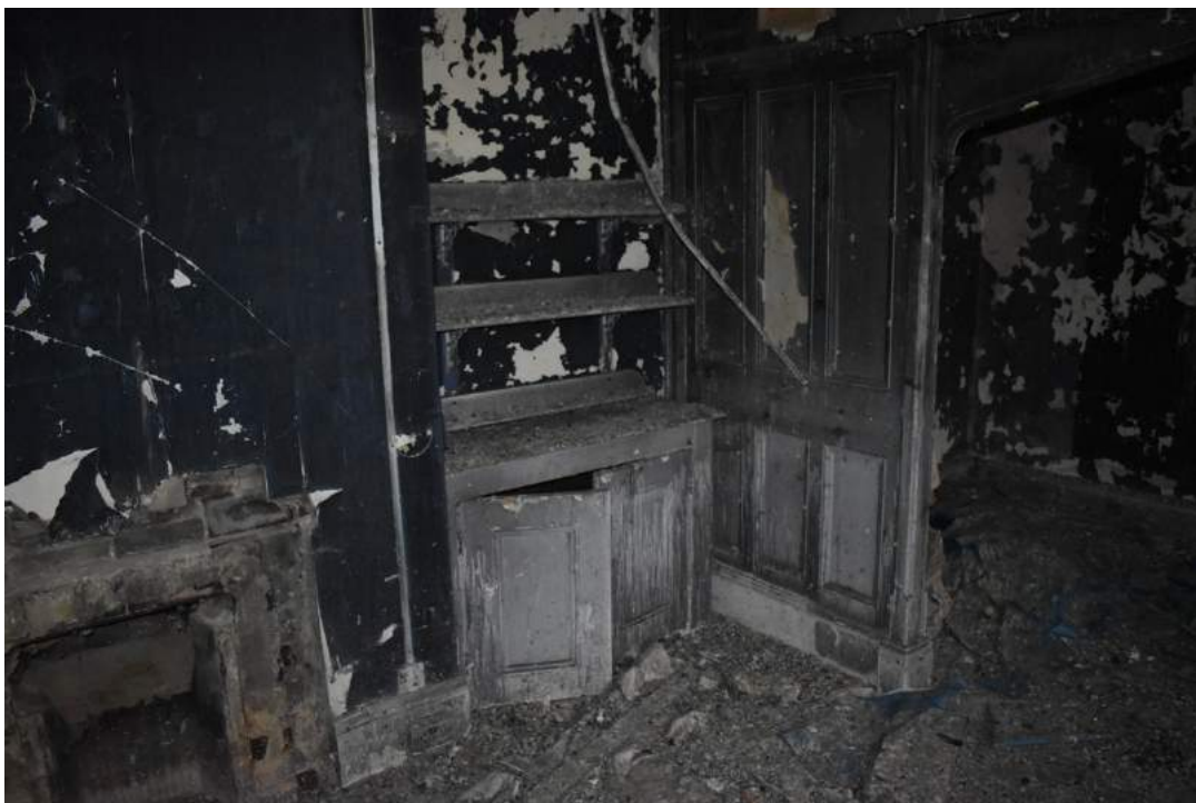
Plate 32 Surviving, but damaged, dresser and shelves in room 27 - view north.
