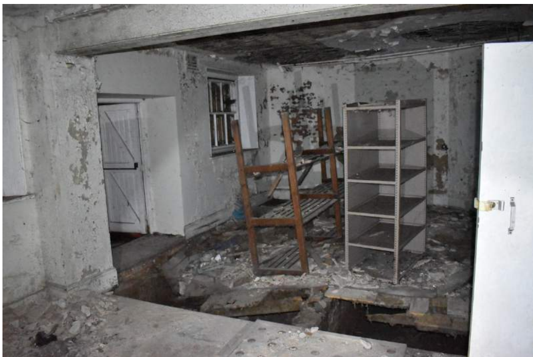
Plate 22 Rooms 39 and 38, the former kitchen and mess manager's room, with the dividing wall removed and a doorway inserted through one of the windows of the mess manager's room – view south. Photo from November 2013 above, photo from December 2019 below.
