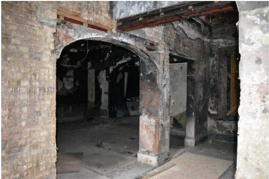
Plate 26 Inserted arch leading into bar with removed wall to right, both supported by metal beams - view west.
