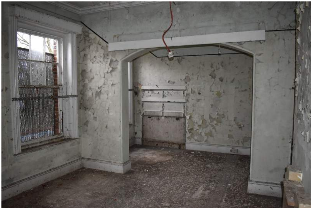
Plate 14 Room 17, the former quarters for Field Officer No.6, showing the repositioned dresser in the sleeping area and the windows without the recessed wooden shutters – view south. Photo from November 2013 above, photo from December 2019 below.
