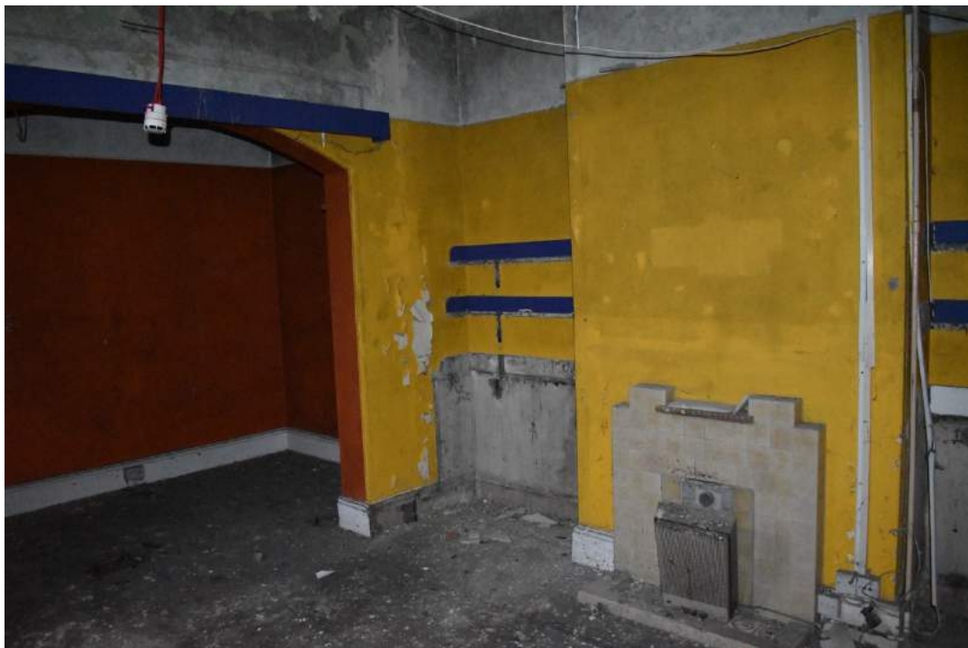
Plate 9 Room 7, formerly the quarters for Officer No.1, showing the brick arch separating the sleeping area from the sitting room, with the original dresser and shelving to the left of the chimney breast – view south. Photo from November 2013 above, photo from December 2019 below.
