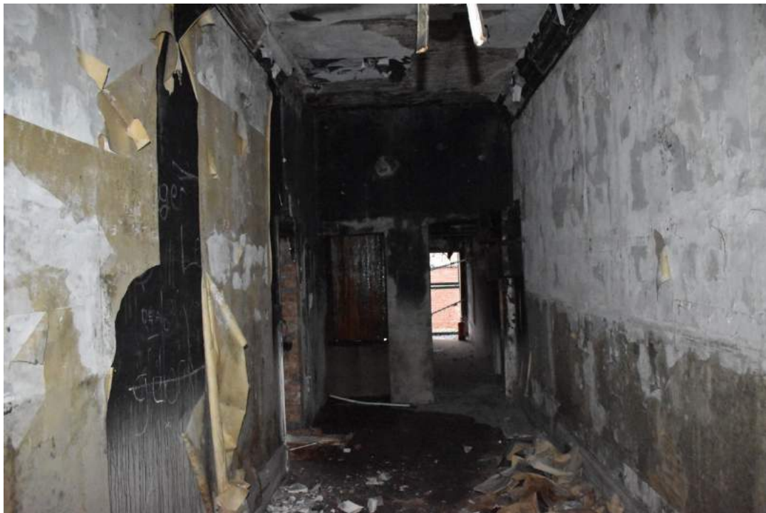
Plate 4 Entrance way iii with the removed staircase and the 1904 toilet block to the rear - view north-west. Photo from November 2013 above, photo from December 2019 below.
