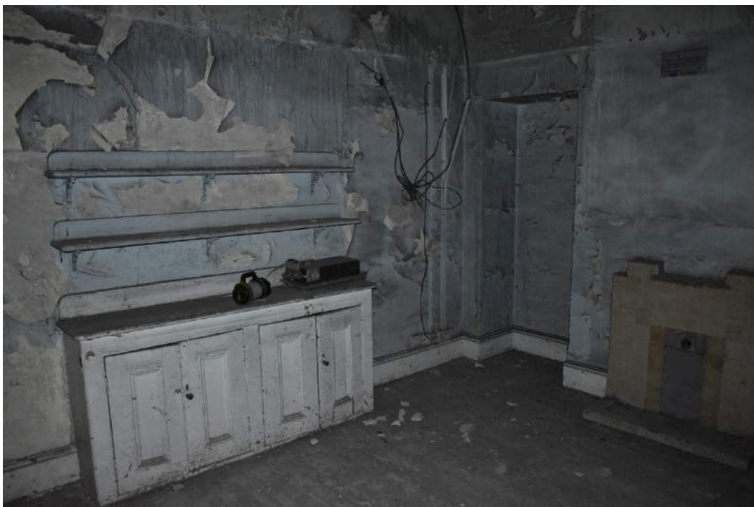
Plate 16 Room 18, formerly quarters for the servants of Officers Nos. 1, 6 and 7, showing the bricked-in original doorway to the left of the chimney breast and the double-width dresser on the dividing wall – view south. Photo from November 2013 above, photo from December 2019 below.
