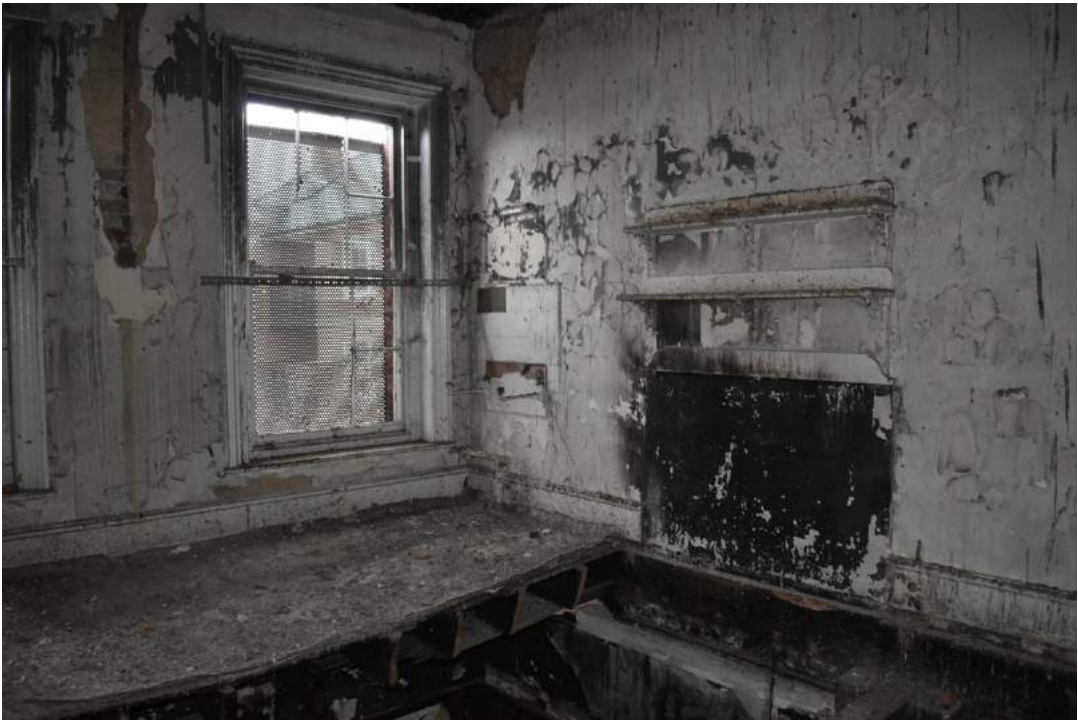
Plate 30 Room 22, showing the missing floor and dresser, but surviving shelves - view north.
