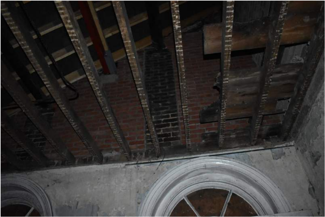
Plate 29 Engineering brick columns supporting purlins socketed into gable brickwork above room 19 - view south-east.
