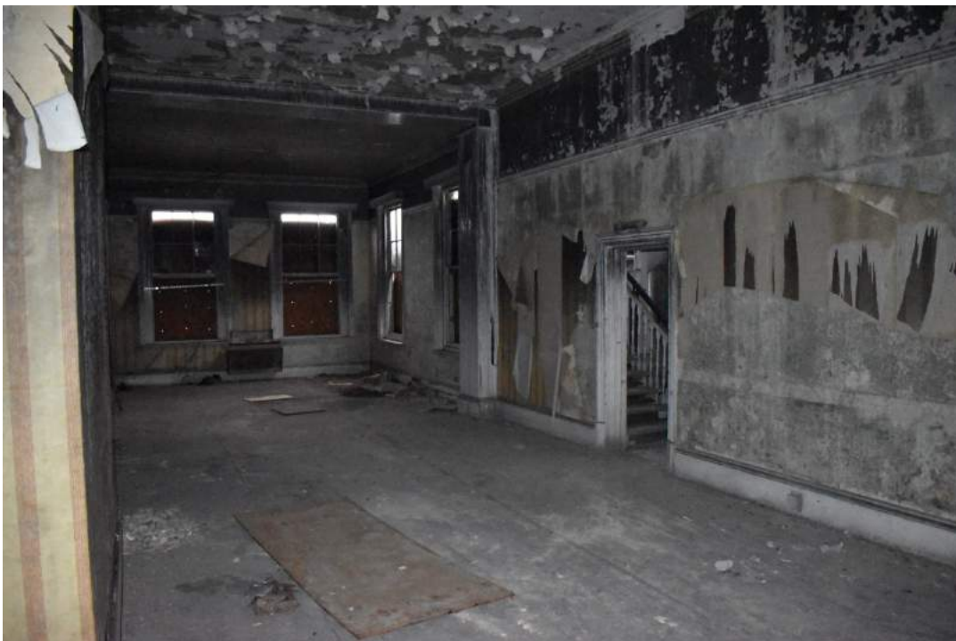
Plate 10 The mess room with the 1922-62 extension to the rear and the original doorway to the servant's stairs in the right-hand wall – view north. Photo from November 2013 above, photo from December 2019 below.
