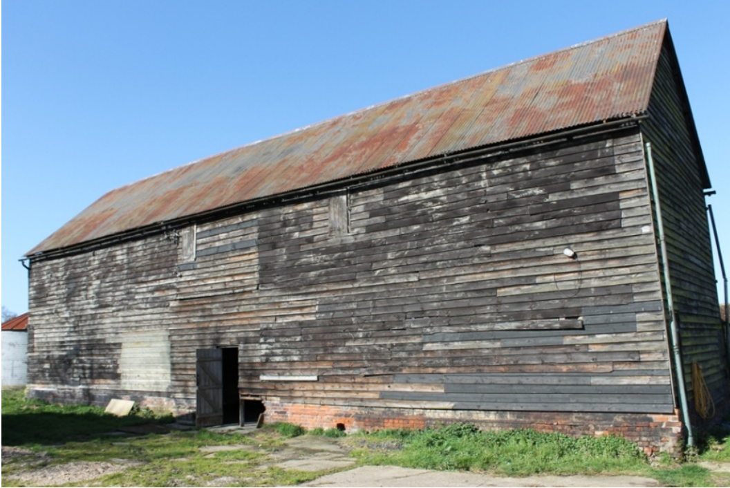
Plate 5 South-east elevation, showing the blocked cart door opening and the inserted pitching doors below the eaves - view south-west
