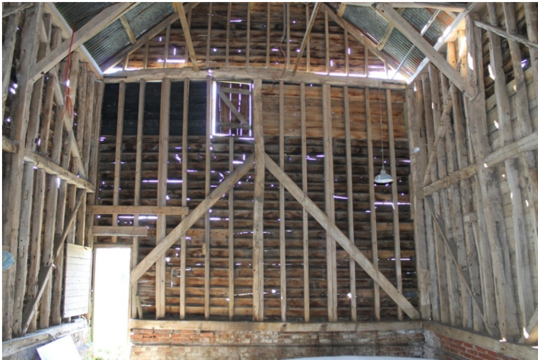
Plate 8 The south-west frame, rebuilt after collapse, with modern machine-cut studs and nailed plank bracing – view south-west
