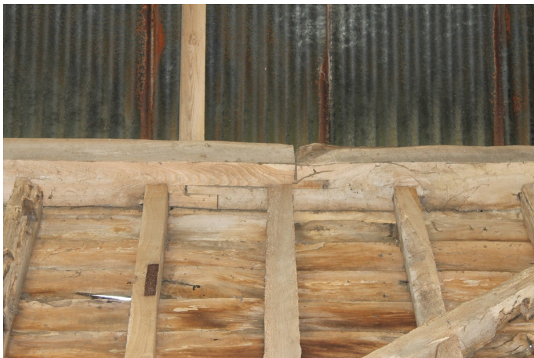
Plate 11 Face-halved scarf joint with bladed abutments, secured by four pegs in the wall plate of bay 5 – view south-east
