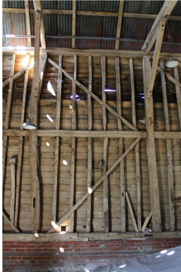
Plate 7 Framing of bay 6, showing the primary bracing forming a diamond pattern - view north-west
