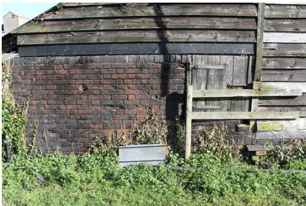
Plate 4 South-west elevation of the lean-to, with Flemish bonded brickwork and the feed door with hinges identical to those of the stable block - view north-east
