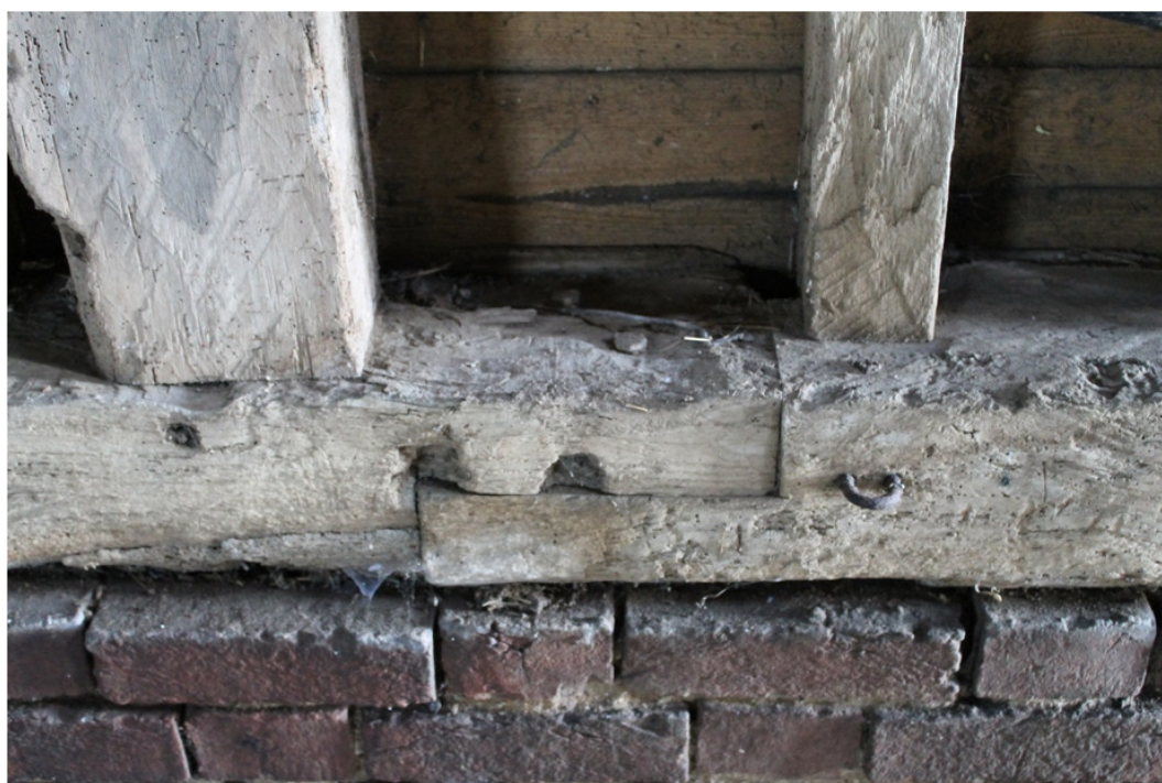
Plate 10 Detail of edge-halved scarf joint, secured by two pegs in the sill beam of bay 6 – view south-east
