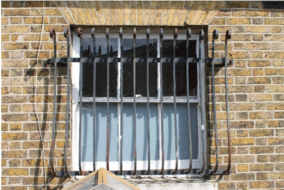
Plate 3 Detail of wrought iron security bars on extension to Spurrier's House - view north-west
