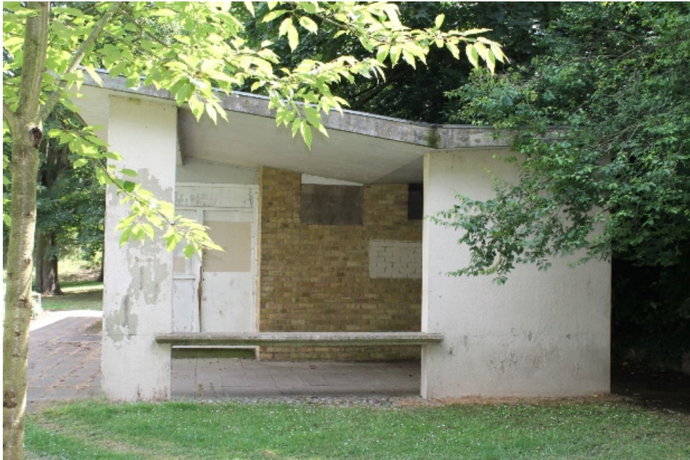
Plate 36 The west end of the Greyhound toilets with the canopy over the bench held by the roof piers - view east
