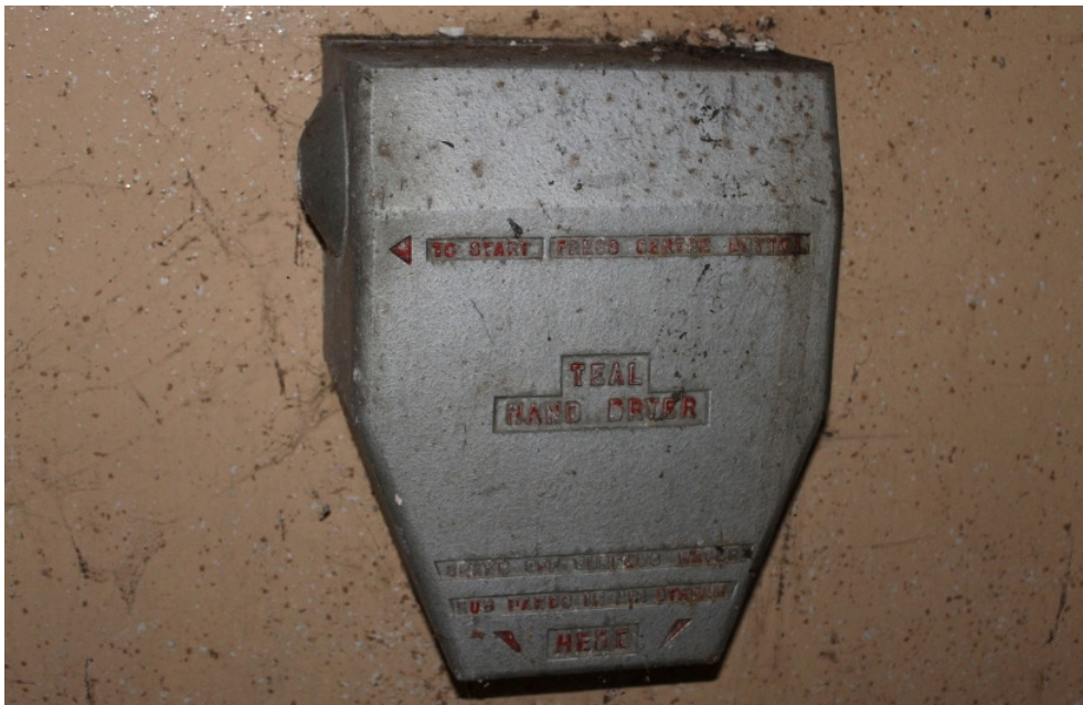
Plate 13 The original 1960s 'Teal' hand-drier in the toilet block at Spurrier's House
