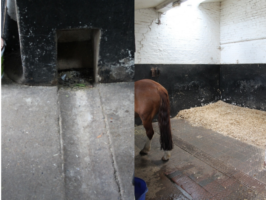
Plate 22 Original drainage gullies and floor surface in the former Spurrier's House stable block
