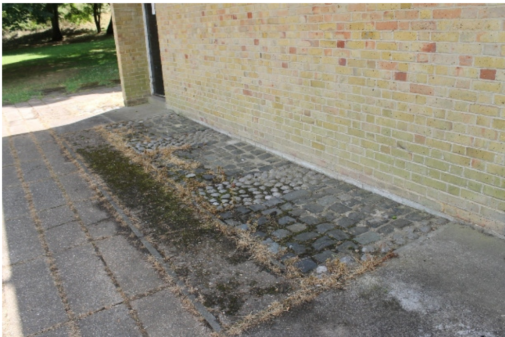
Plate 37 Tactile surface outside the Greyhound toilets, possibly recalling the duck pond of Pets Corner - view east
