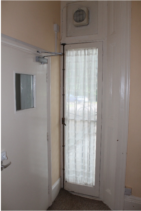
Plate 5 Original French doors of Spurrier's House truncated by inserted stud wall - view north-west
