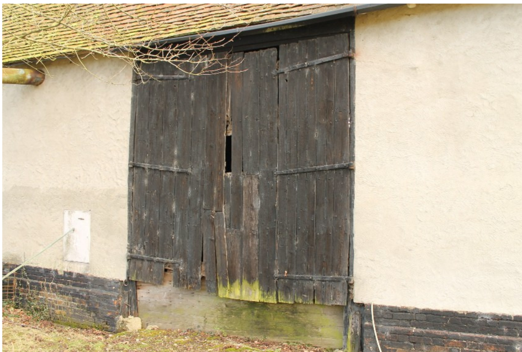
Plate 3 Full-height barn doors in the south-west elevation of the Grain Barn with original strap and pintel hinges - view north
