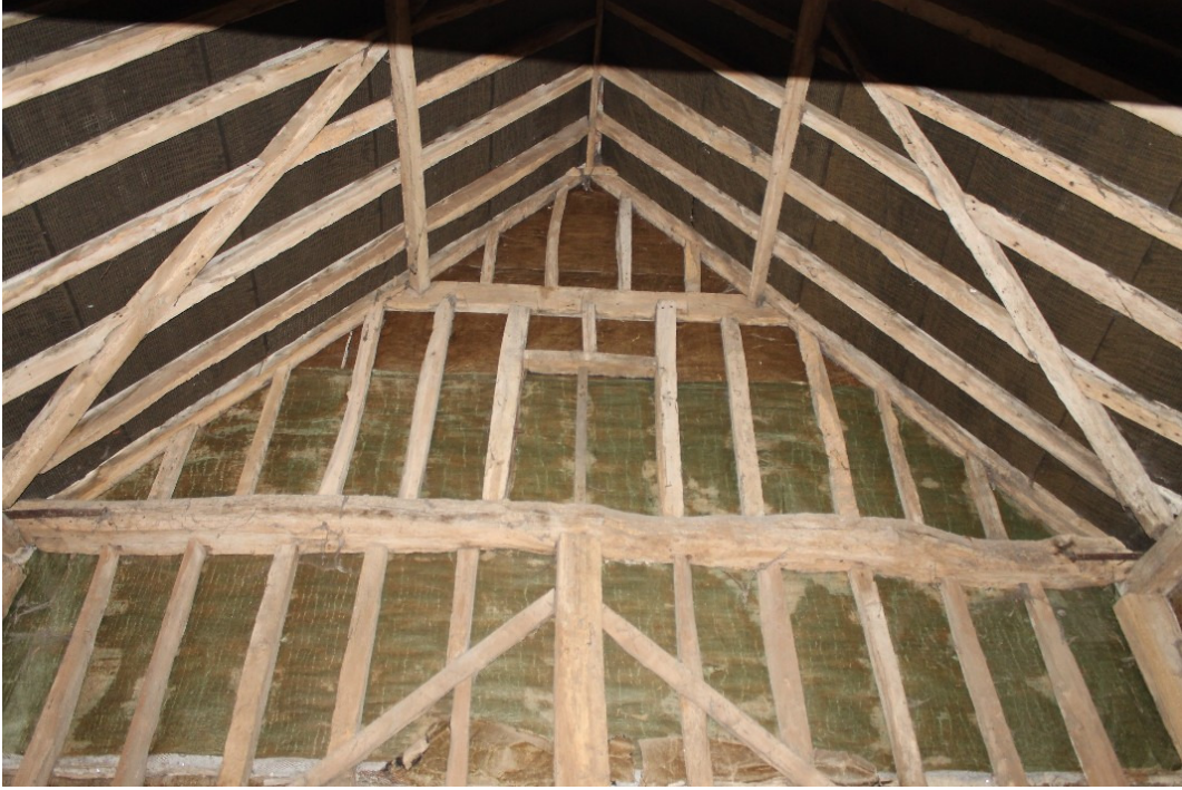
Plate 11 South-west gable frame of the Church Barn with inserted window above the wall plate – view south-west
