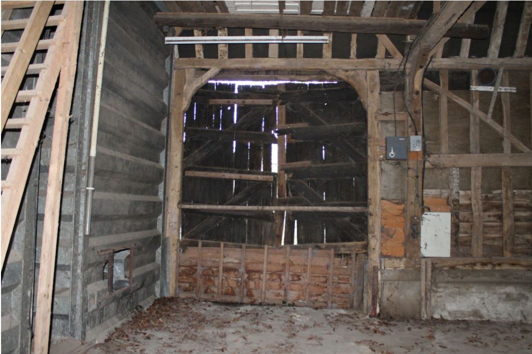
Plate 5 Barn doors in south-west wall of Grain Barn with roughly squared knee braces - view south-west
