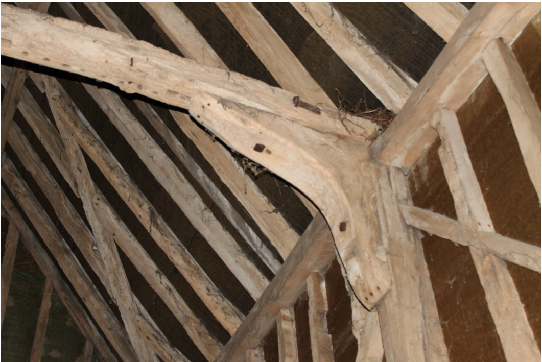
Plate 12 Large hewn knee brace supporting re-used tie beam of truss A in the Church Barn - view west
