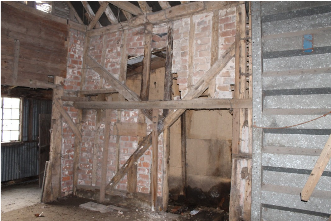
Plate 6 South-east wall of the Grain Barn midstre showing the Y-shaped bracing and brick noggin - view east
