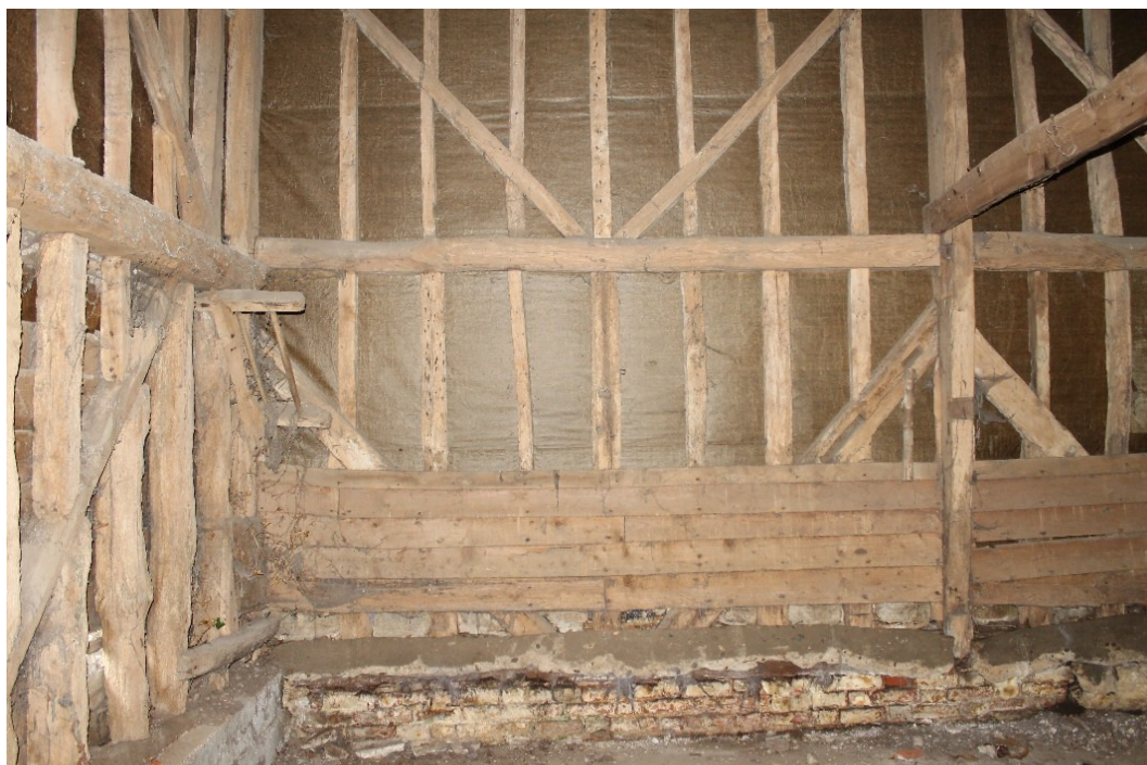
Plate 14 Plank cladding to wall of bay 1 and remains of hay rack, indicating bays 1-3 of the Church Barn were once used to house animals - view north-west
