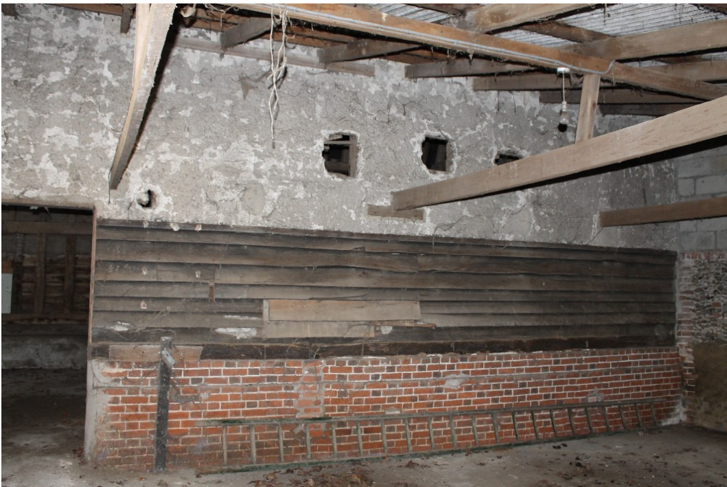
Plate 2 Detail of the brick plinth to the Grain Barn with weatherboard above this and then render covering the upper portion of the frame – view west.
