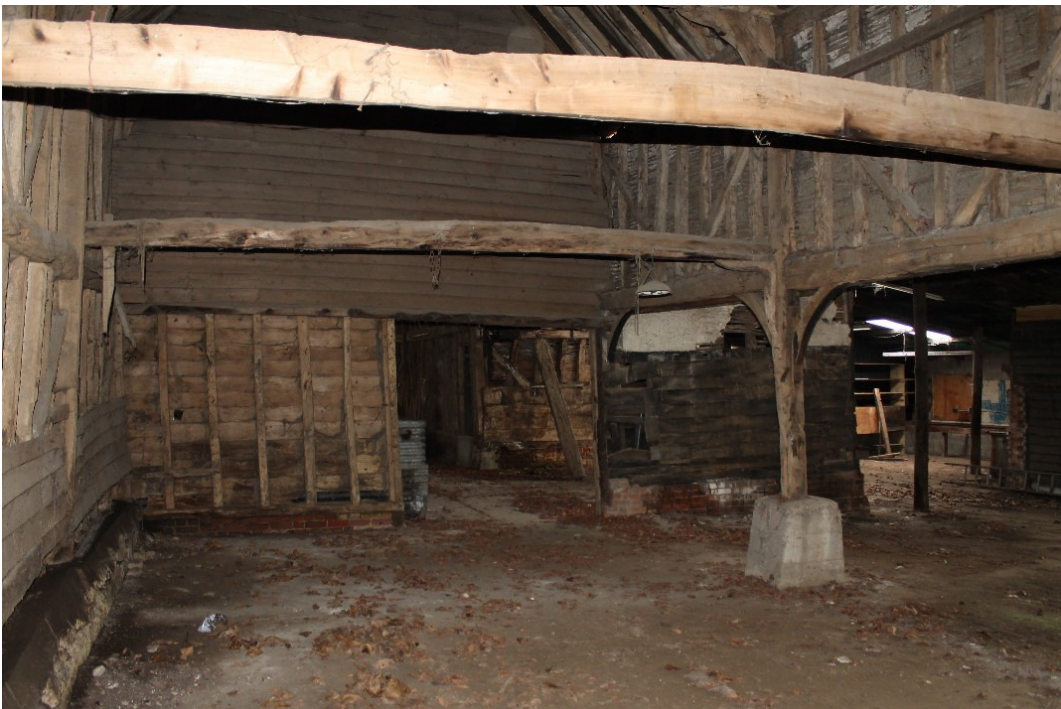
Plate 10 The interior of bays 2-3 in the Church Barn, converted to a cart lodge by the removal of the lower framing – view east
