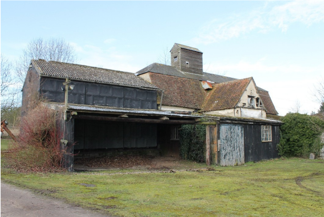
Plate 1 North-east elevation of the Grain Barn, partially obscured by 20th-century outbuildings - view north-west
