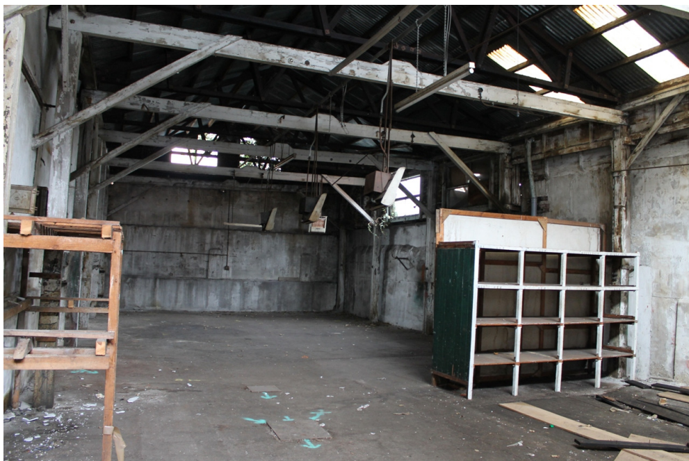
Plate 9 Interior of the workshop, showing the original timber frame and the later roof - view north-west
