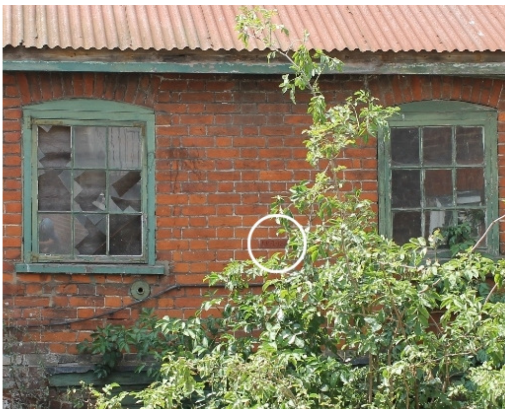
Plate 2 East elevation of the converted 1830 house with the date brick circled – view west
