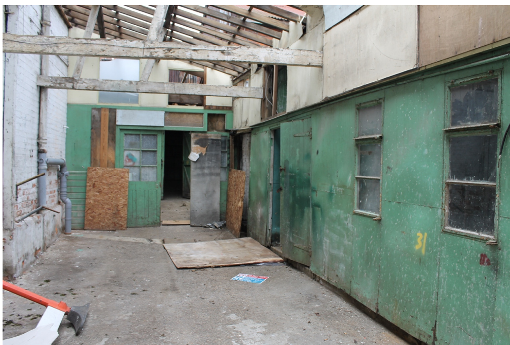
Plate 13 Inserted metal-framed windows in the south wall of the wooden shed – view west
