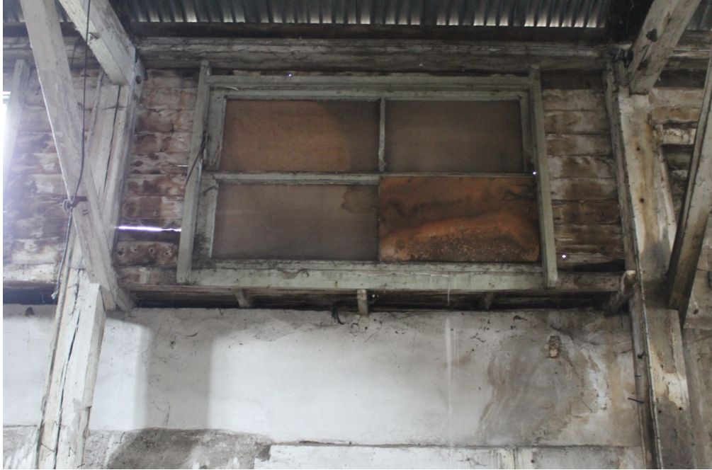
Plate 10 North wall of the workshop, showing the structure built on the adjoining property wall - view north
