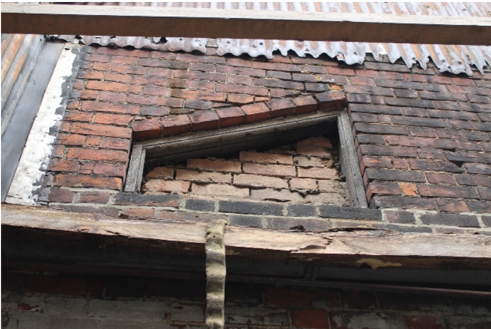
Plate 4 The rebuilt first floor wall of the converted 1830 house, showing the irregular-shaped window – view north
