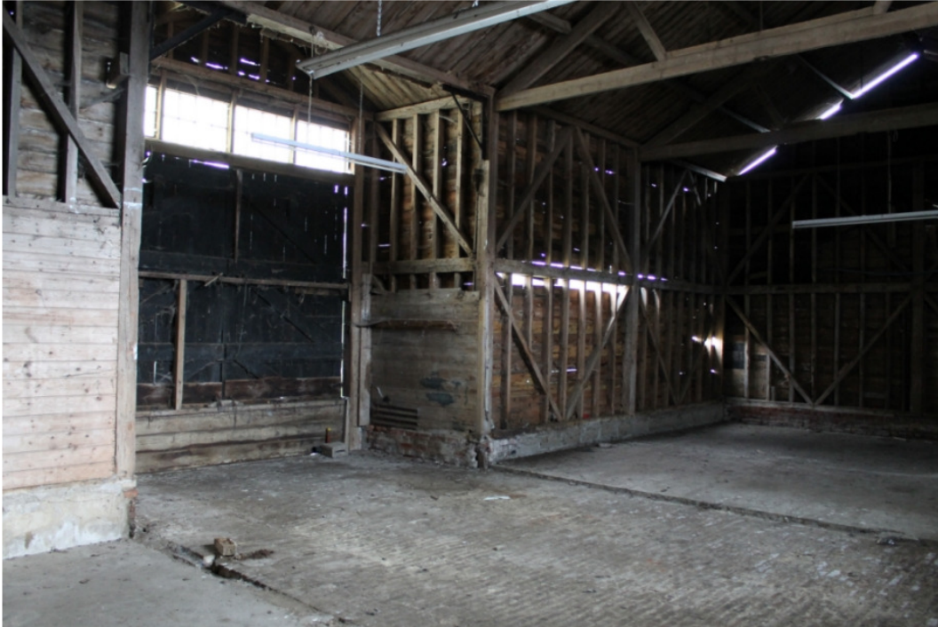
Plate 5 Interior of the barn showing the midstreay threshold leap and brick threshing floor – view east
