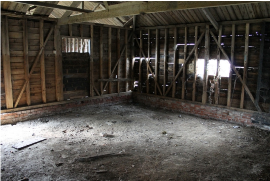
Plate 19 Chaise house interior showing the inserted and subsequently blocked doorway to the 'four-bayed' cattle shed - view south-west
