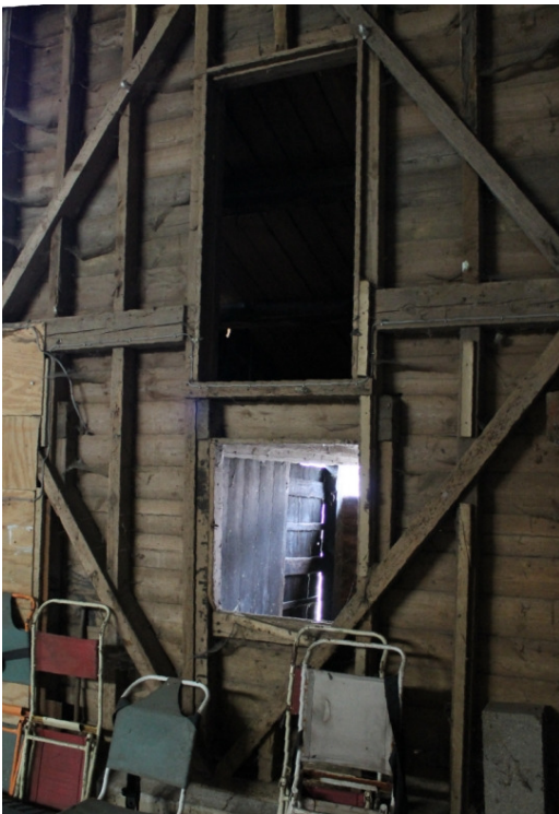
Plate 6 Barn, bay 3 showing inserted hatch to cattle shed and inserted doorway to chaff loft - view north-west
