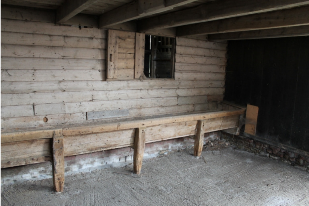
Plate 26 Lean-to cattle shed showing manger with chaff loft above and hatch into main barn – view north
