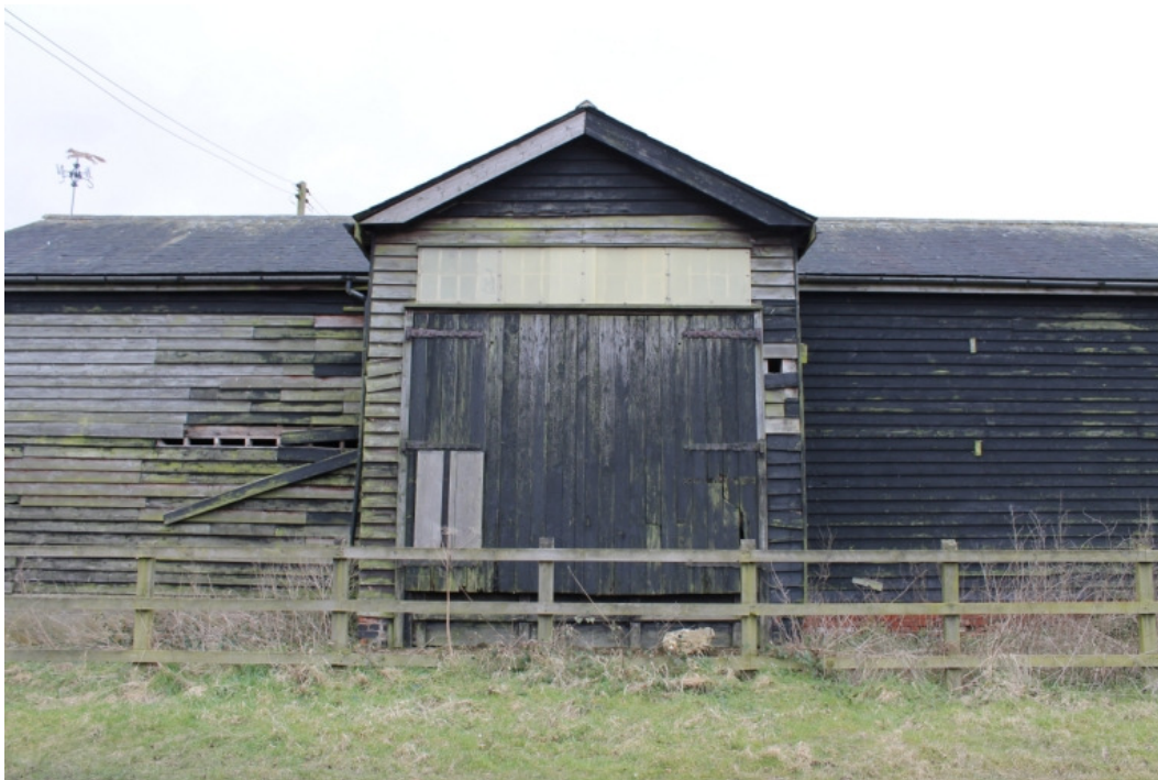
Plate 3 Midstrey to barn with original doors, threshold leap and inserted metal-framed windows – view south-east
