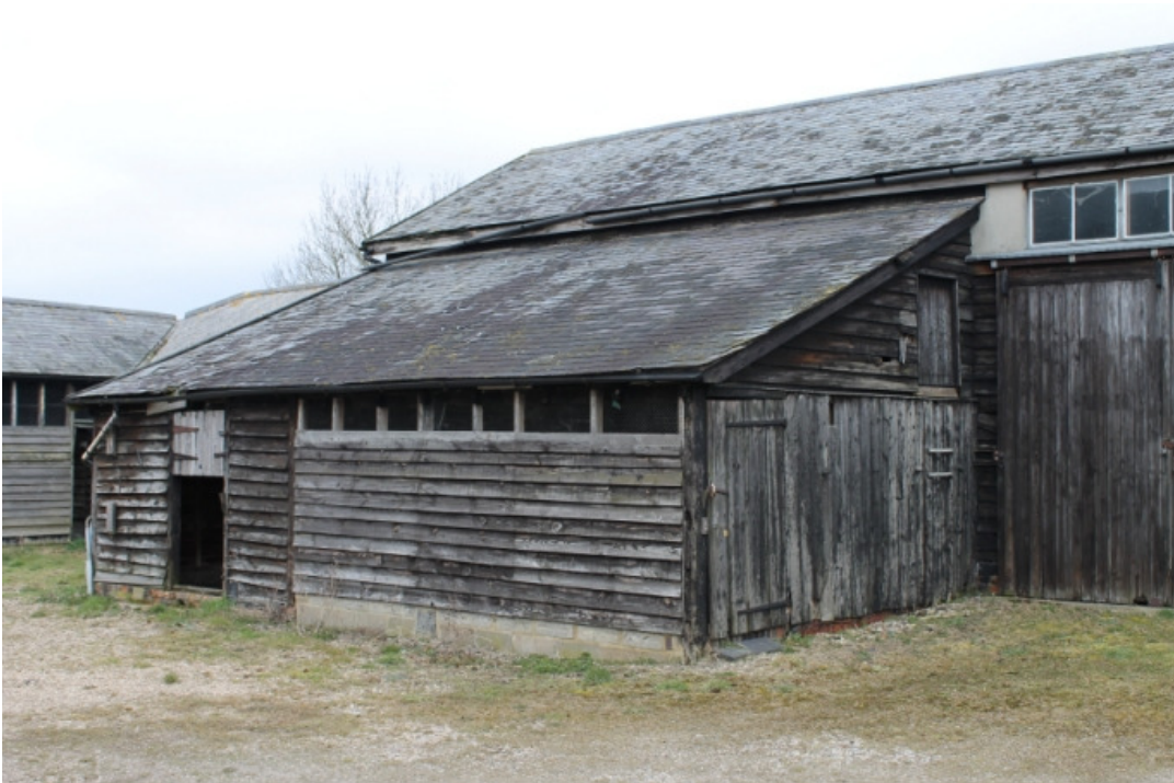
Plate 23 Lean-to cattle shed showing blocked open front and door to chaff loft - view north-west
