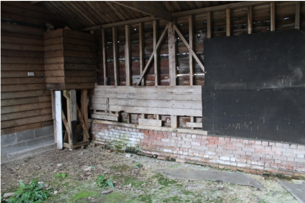
Plate 21 Interior of the 'four-bayed' cattle shed showing the remains of the manger - view west
