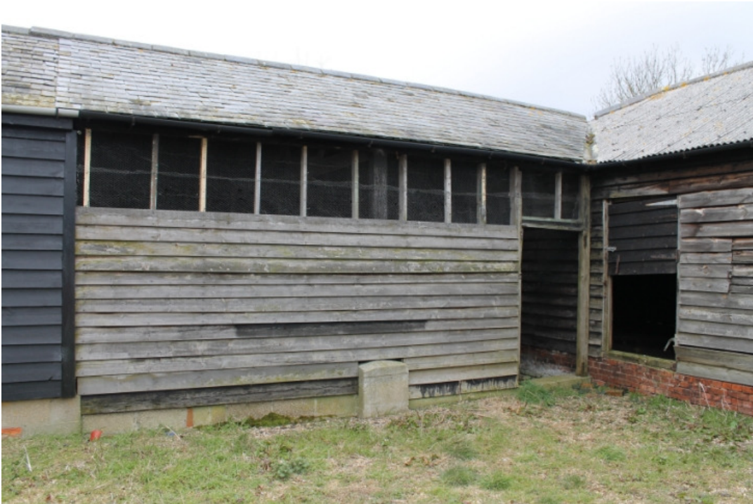
Plate 20 'Four-bayed' cattle shed showing the blocked open front with the chaise house to the right - view west
