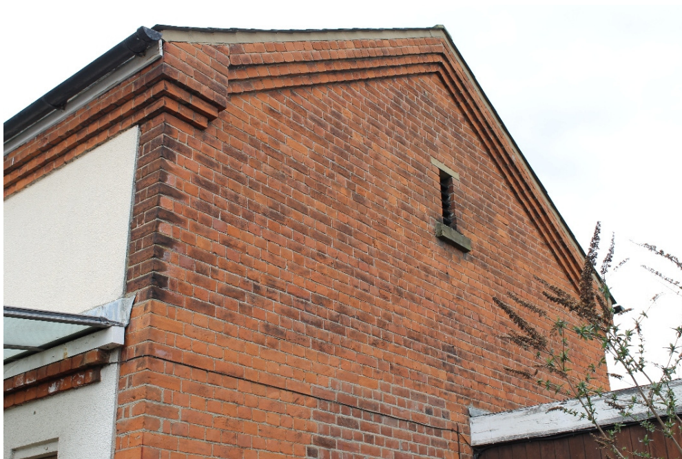
Plate 10 East elevation of MEE 03, showing ventilation louvre in gable end - view north-west
