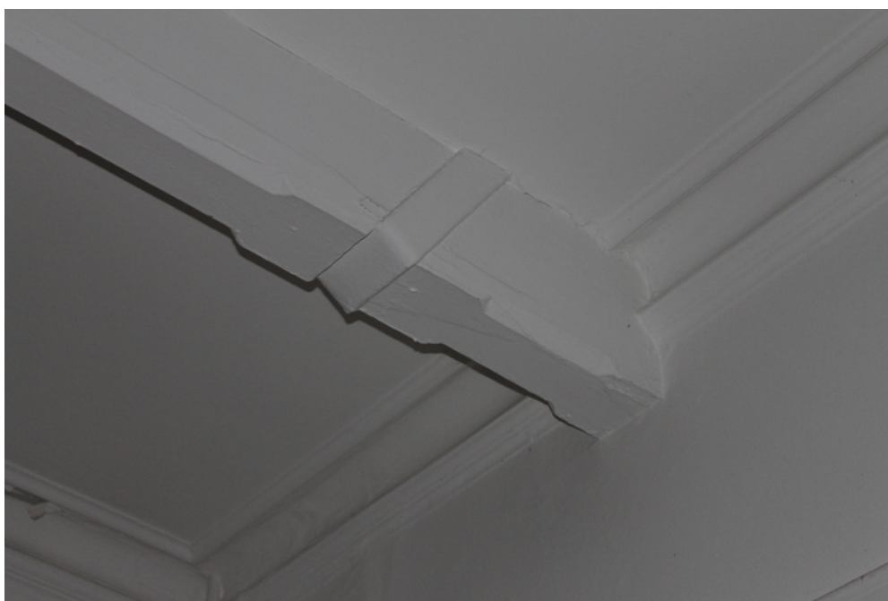
Plate 28 MEE 17 exposed chamfered tie beam of roof truss, with recess for iron strapping
