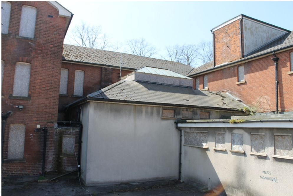
Plate 18 - The Billiard Room with the 1958-61 service area to the right - view south-west
