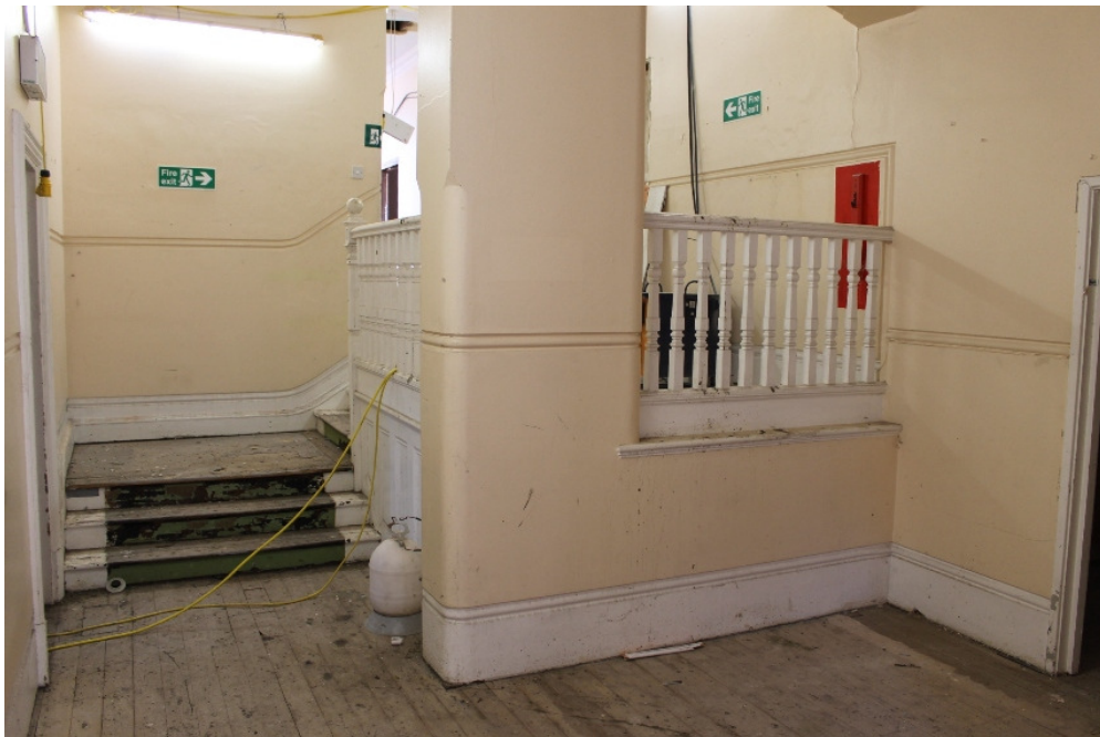
Plate 46 HYD 08 original balustrades to landing with entrance to the former north stairs on the right - view south
