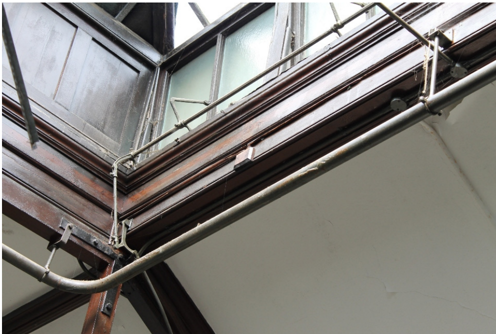
Plate 42 HYD 08 Billiard Room, detail of the metal armatures governing the opening and closing of the lantern windows
