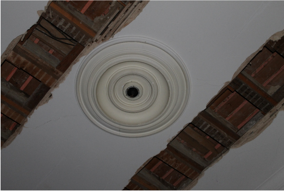
Plate 37 HYD 08 original plaster light fixture in Mess and Ante Rooms
