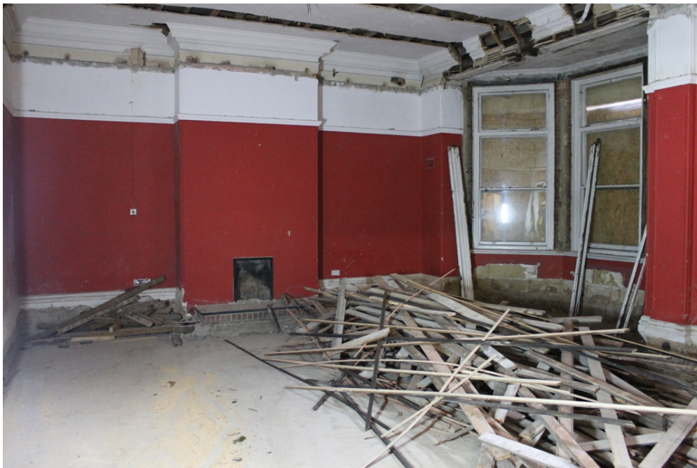
Plate 36 HYD 08 Ante Room, showing the working fireplace and evidence for the lowered ceiling – view south
