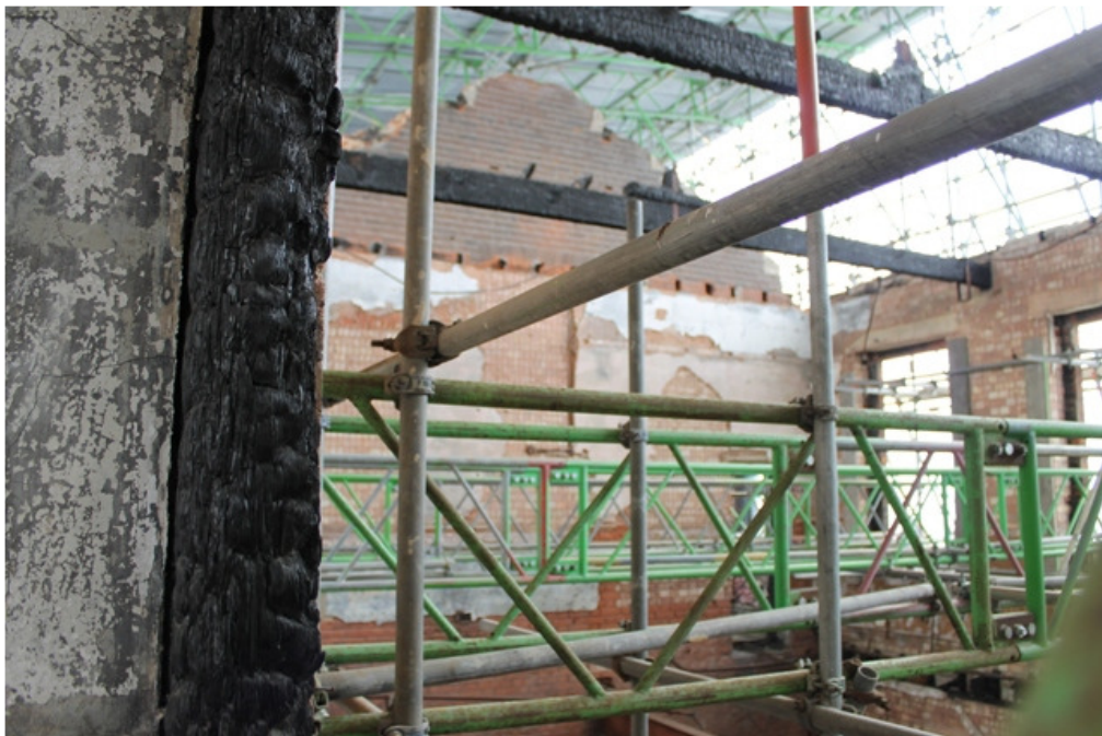
Plate 57 Charred tie beams of HYD 11, showing evidence for king post roof trusses – view south-east
